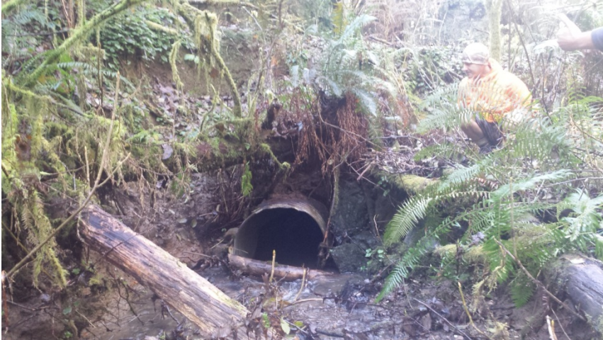
Figure 1. WQ1- View looking downstream to inlet of 48" diameter culvert on Class I tributary of Janes Creek. Photo taken by RWB staff Joelle Geppert December 28, 2016.
