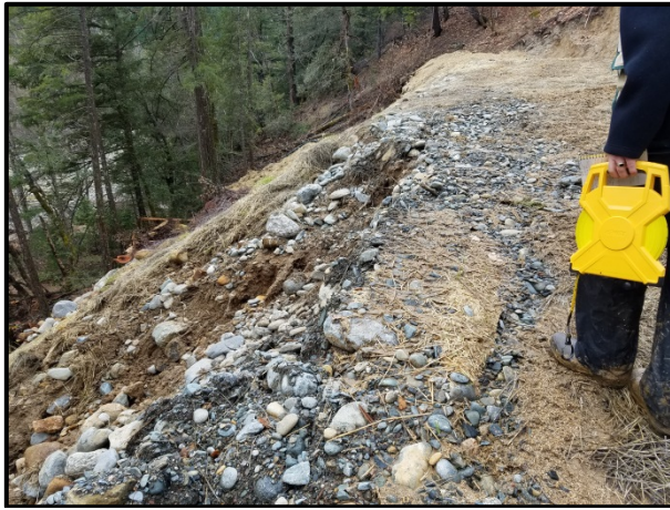
Photo 11: Erosion of the fillslope (Graham Brown, December 20, 2016)
