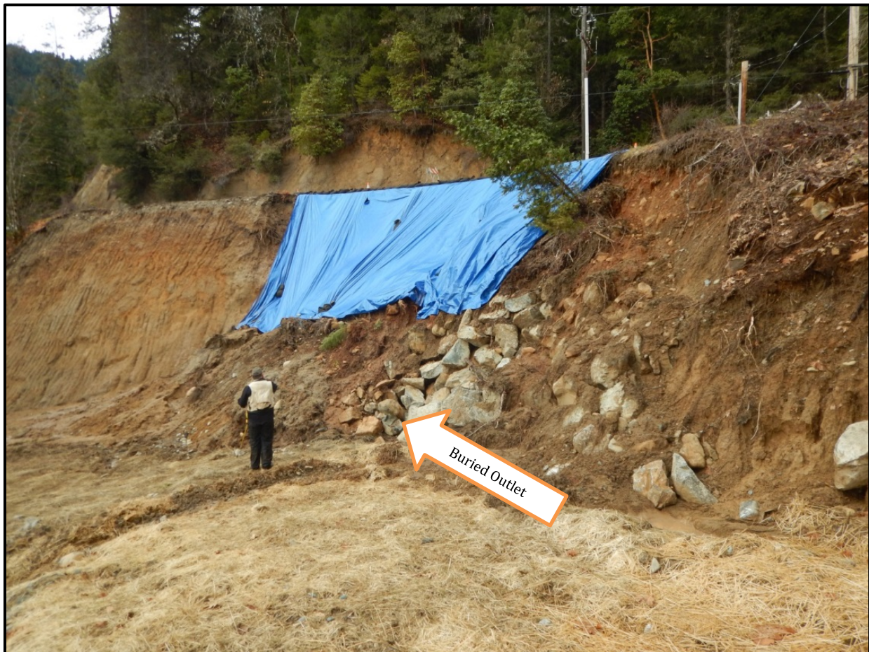
Photo 1: The failing cutslope (Graham Brown, December 20, 2016)
