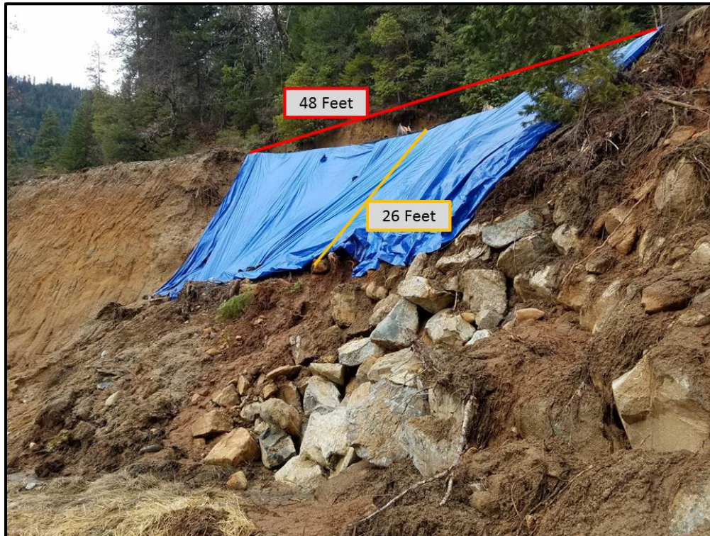
Photo 2: Annotated figure illustrating dimensions of the failed cutslope (Graham Brown, December 20, 2016)
