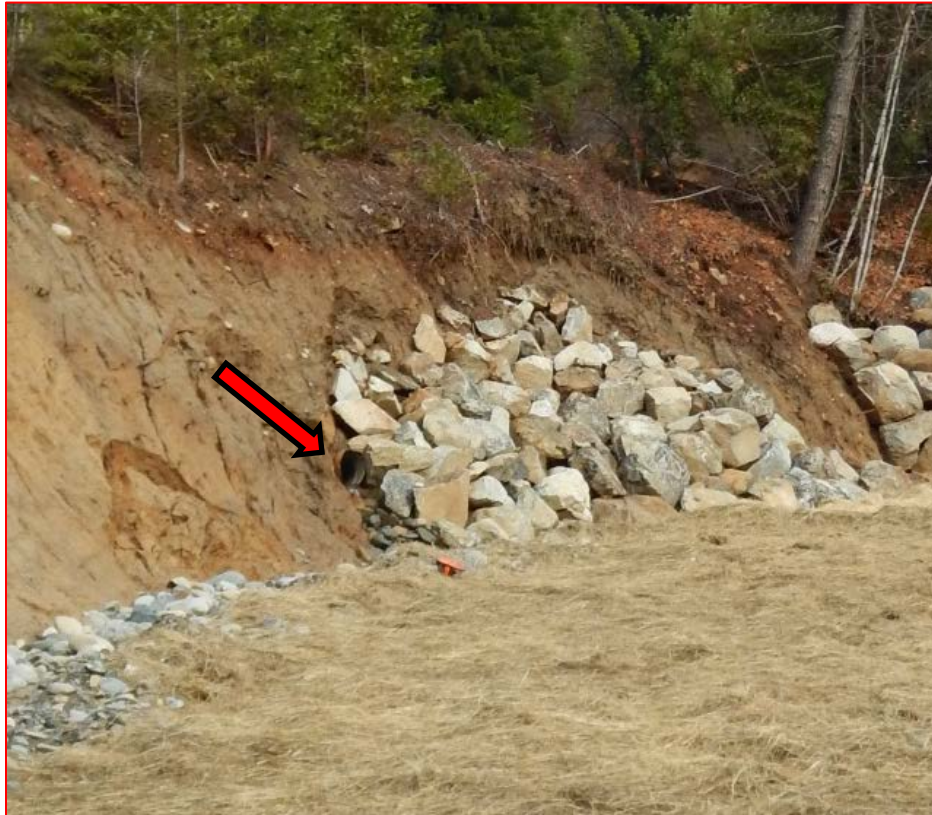
Figure 5: 18-inch CMP outlet of the Class II watercourse crossing on Trinity Alps Road
