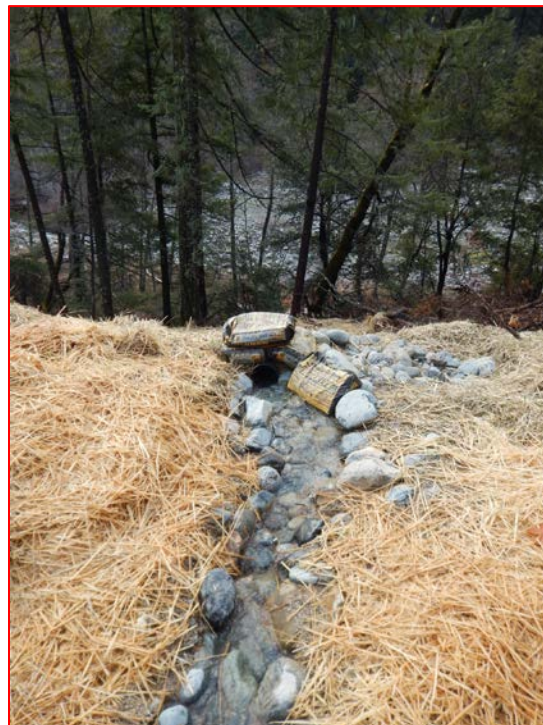
Figure 7: Inlet of six-inch plastic pipe that extends to the floodplain of Stuart Fork
