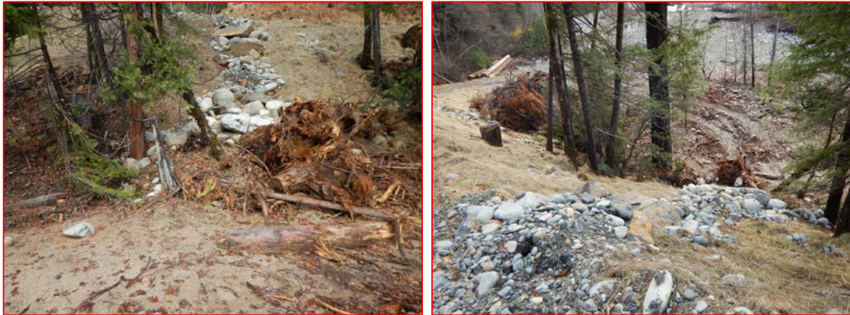
Figure 3: Failure in fill slope of new seasonal road construction, from below (left) and above (right)
