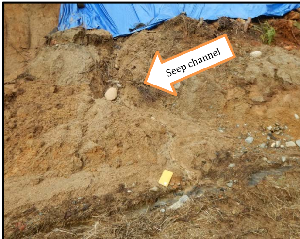
Photo 4: Seep on west side of cutslope failure (Graham Brown, December 20, 2016)
