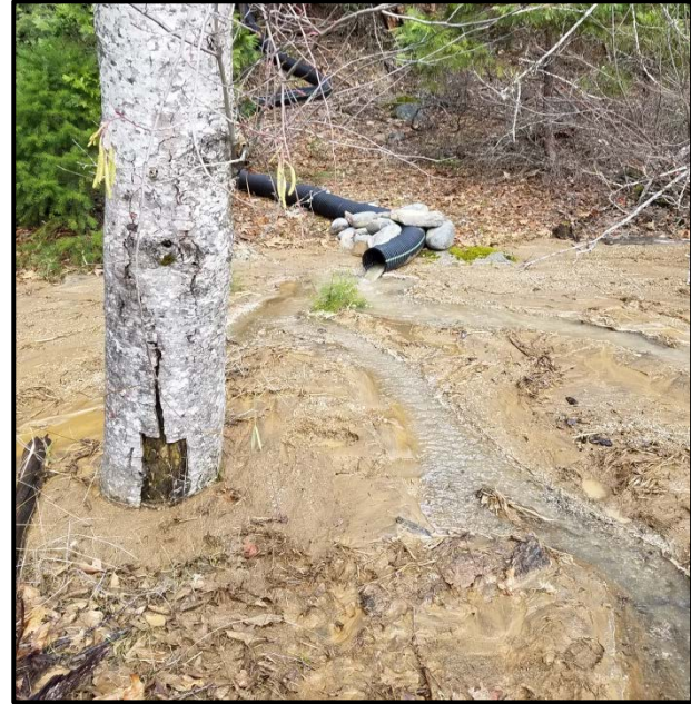
Photo 7: Plastic flexible pipe discharging onto Class I floodplain of Stuart Fork (Graham Brown, December 20, 2016)
