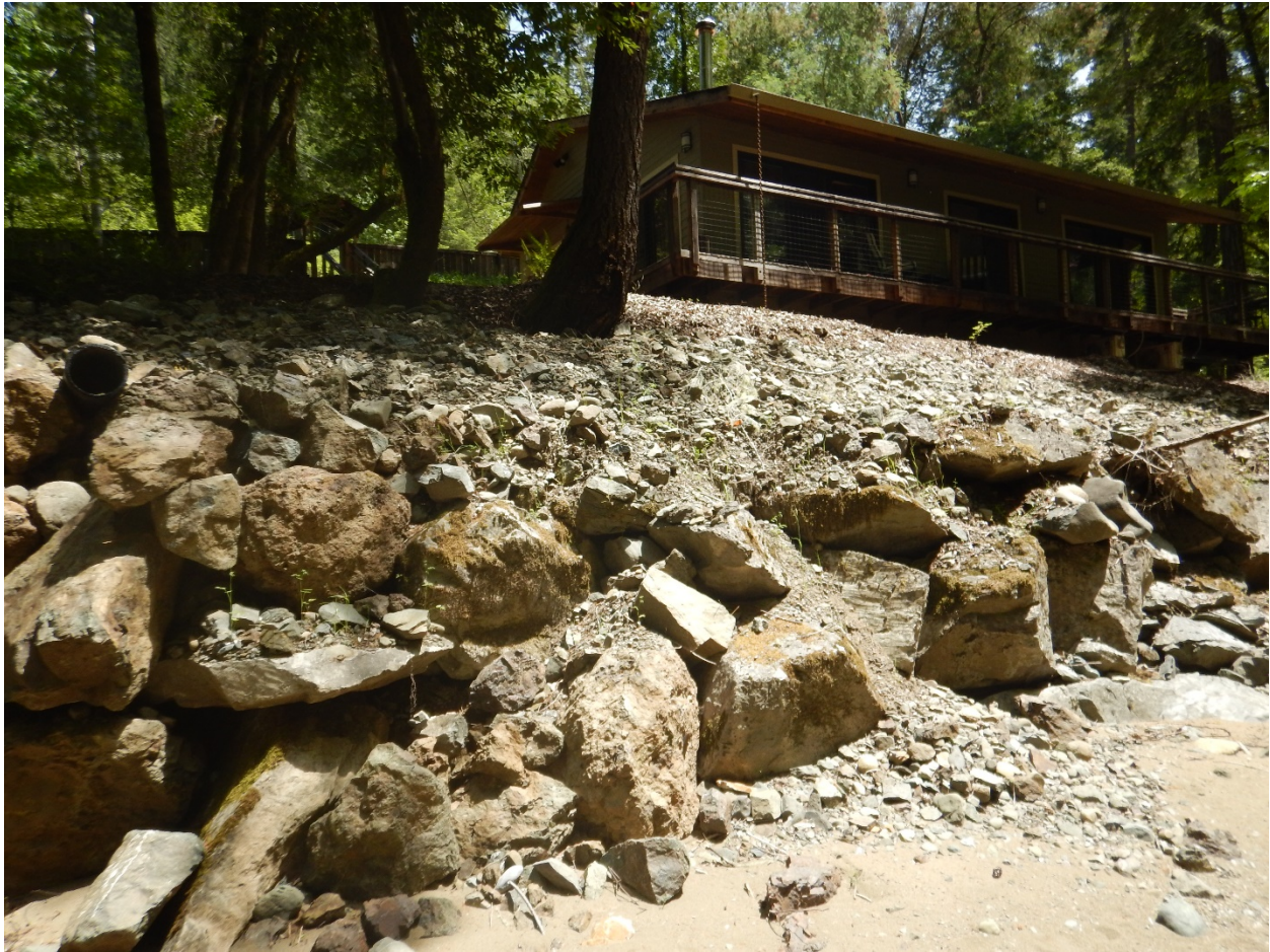
Figure 11: Small-diameter fill material has been placed above the existing rip-rap and it is falling down into the channel. Photo taken by Kaete King 5/10/2018.
