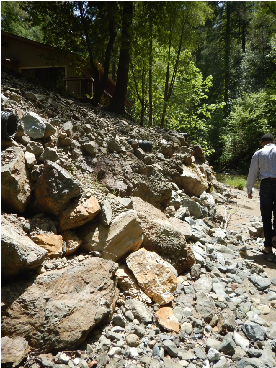
Figure 9: Post-construction rip rap and fill in area that was to be left undisturbed. Smaller fill material is spilling down between rip rap. Notice poorly installed planting tubes. Photo taken by Kaete King 5/10/2018.
