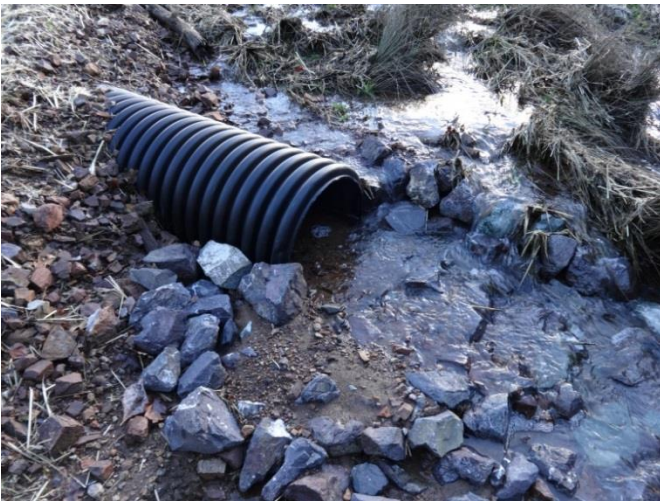
Image 47 shows the outlet of a recently installed culvert delivering into a stream. Note the sediment deposits in the culvert reducing carrying capacity and providing evidence of upstream erosion, sediment delivery and transport. (Brandon Rose photo 118).
