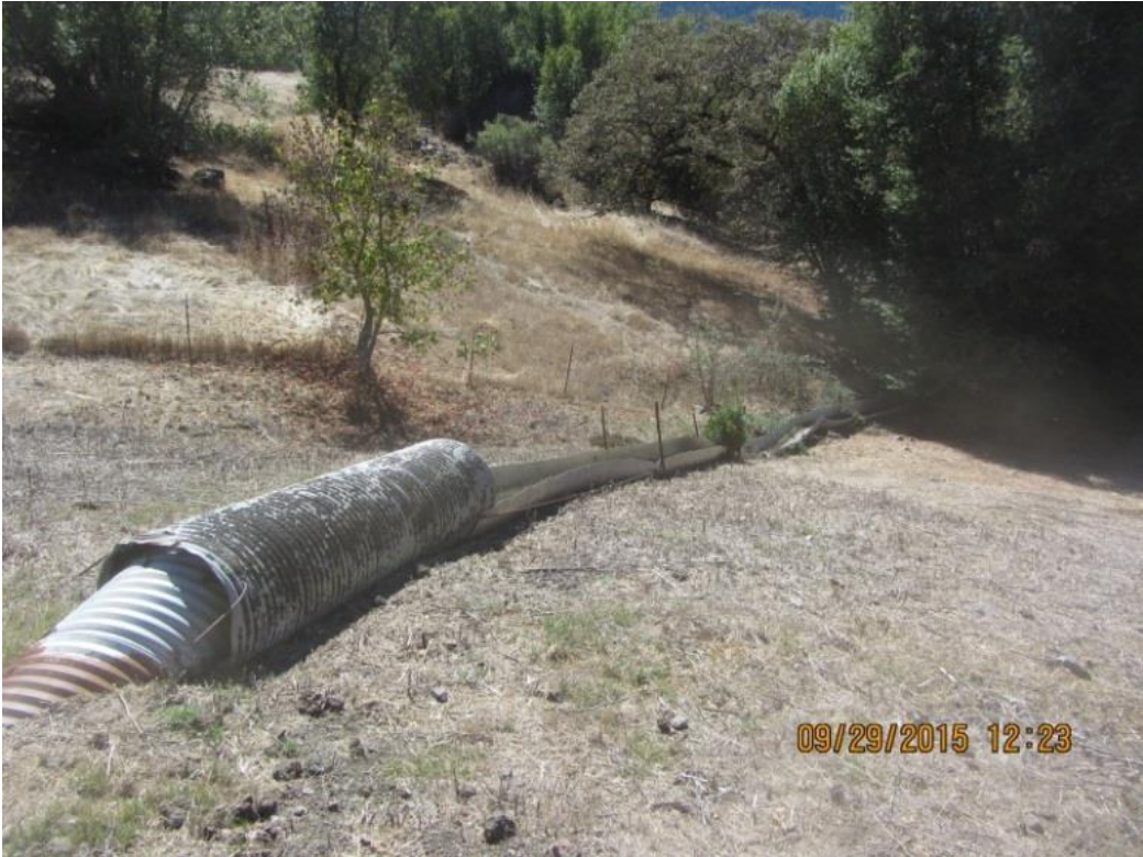
Image 28 shows the outfall from the smaller pond (GPS 9). Note the culvert and half pipe do not appear to be structurally sound; however, the half pipe was carrying flows during the inspection. (IMG_0284)
