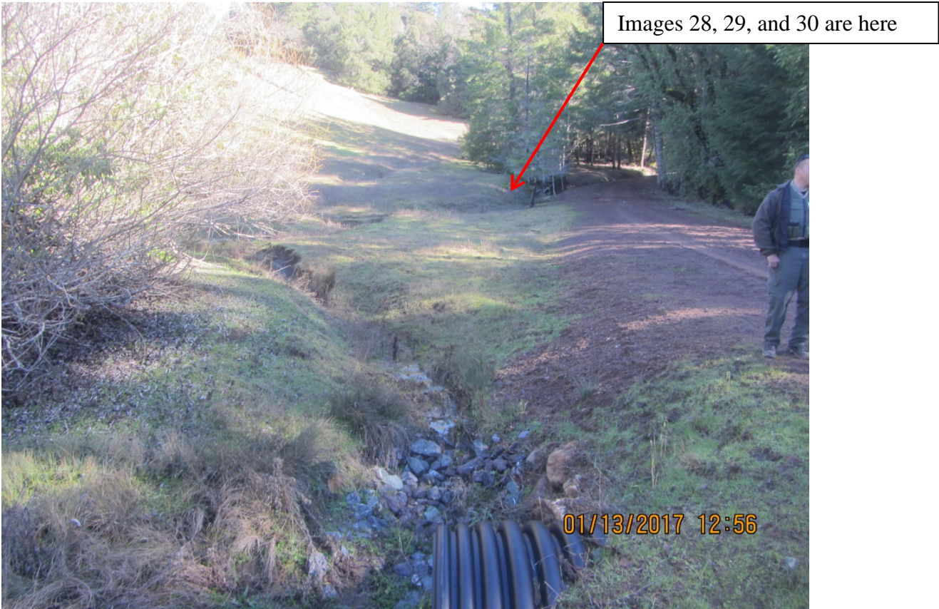
Image 33 shows the inside ditch and intercepted stream leading to the culvert outlet of Stream Crossing 7 in image 32 above. (IMG 3053)
