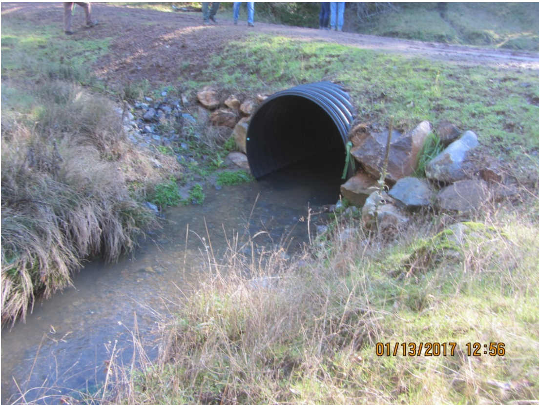
Image 32 shows the outlet of Stream Crossing 7, note the connection of the inside ditch and intercepted stream in the upper left hand corner of the image.
