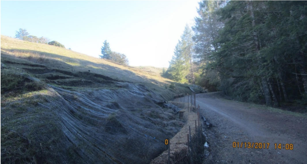
Image 60 shows GIS point Landslide 1; note the multiple scarps slumping towards the road. (IMG 3132_3133 stitch)
