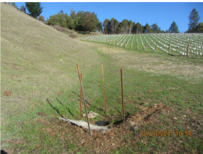
Image 11 shows a subdrain inlet in the location the original stream once flowed. (Image 2928)
