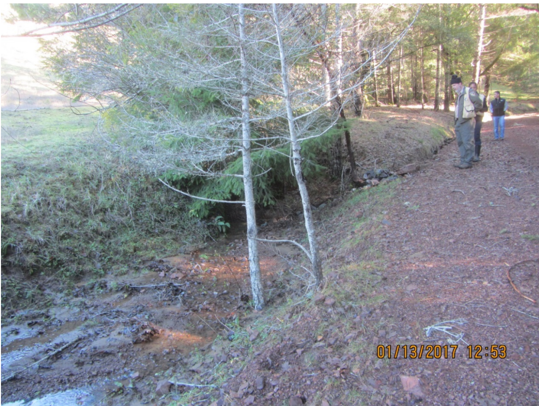
Image 28 shows the connection of an inside ditch and intercepted Class II/III stream to the outlet of Stream Crossing 7. Note the visible sediment deposits in the foreground of the image. (IMG 3044)
