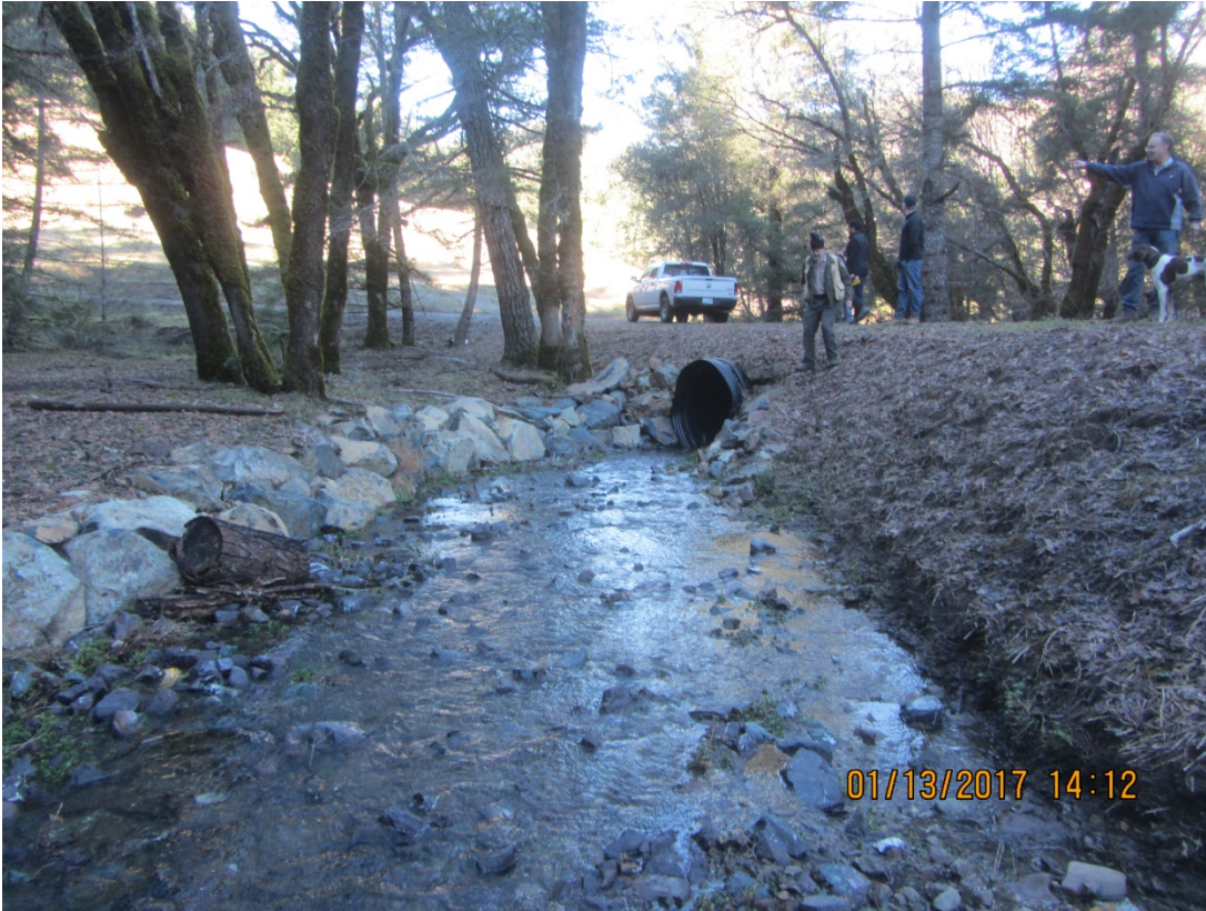
Image 64 shows the inlet of Stream Crossing 19, note the rock fill placed in the stream. (IMG 3143)
