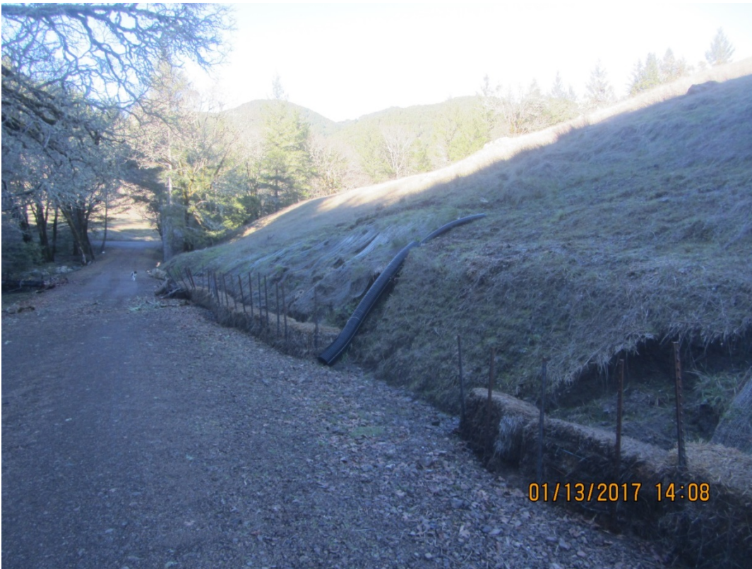
Image 61 shows the Landslide 1 from a different vantage point- of note is that access road in this vicinity parallels a Class I or Large Class II stream for a significant distance, increasing the delivery potential of these unstable slopes. In these images one can also see the connection of the inside ditch along the road with the landslide materials. (IMG 3135)
