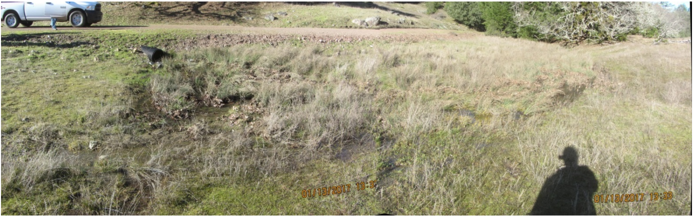
Image 44 shows the outlet of Stream Crossing 12; note the flows from the culvert outlet support a wetland. (IMG 3076-3080 stitch)
