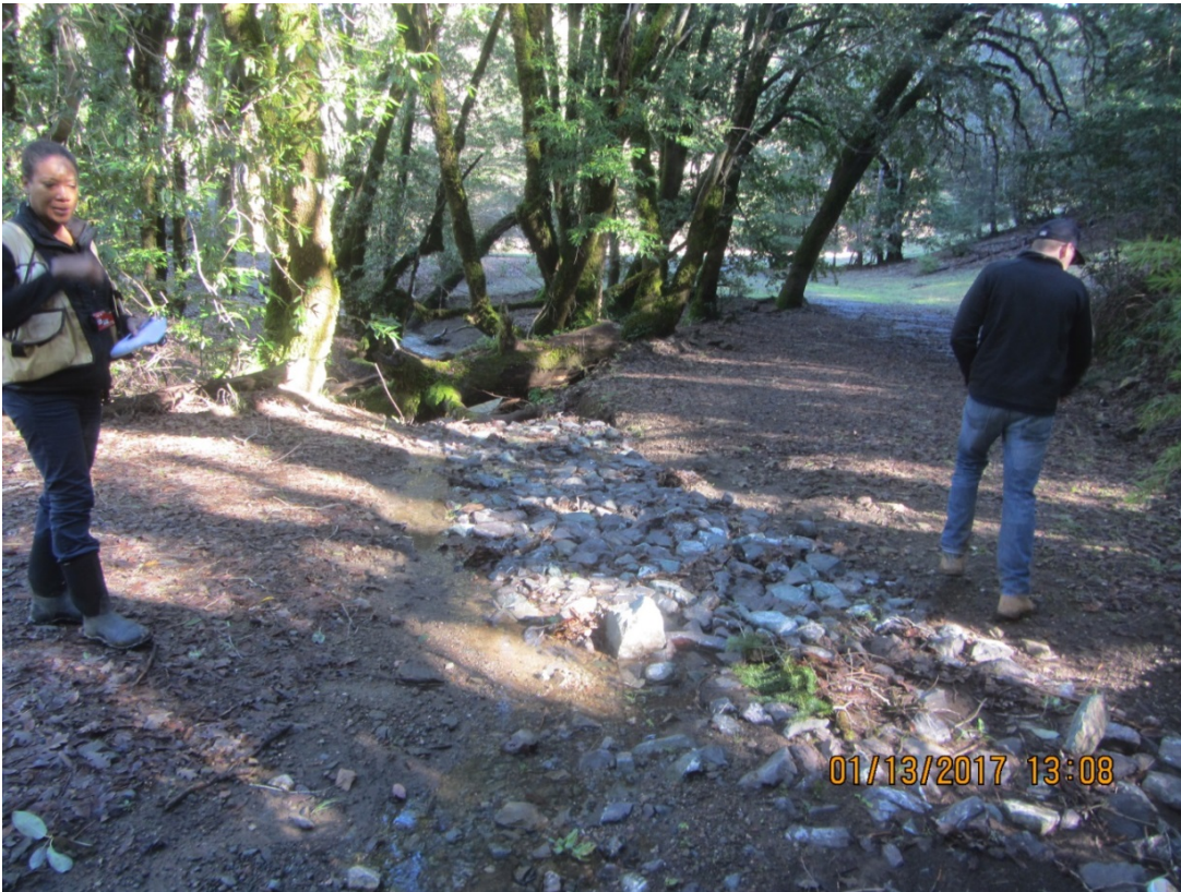
Image 38 shows the Class II stream diversion crossing the road in a shallow ford (installed subsequent to the 2015 inspection,) and the stream diversion leading to the flat that then flows into the inlet of Stream Crossing 8. (IMG 3065)
