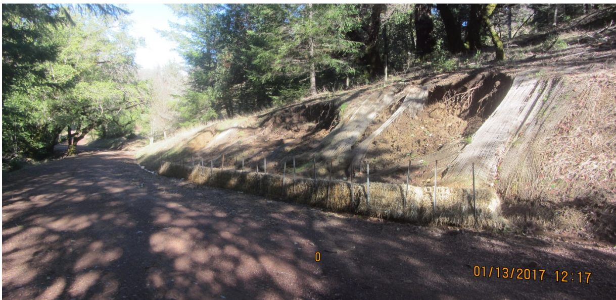
Image 17 shows the bank slump along the access road; note the flow in the ditch along the front of the slump. This flow is continuous to the next cross drain at Stream Crossing 2 where the flow discharges to the culvert inlet. Bank slumps such as this are common along the recent construction of the access road.
