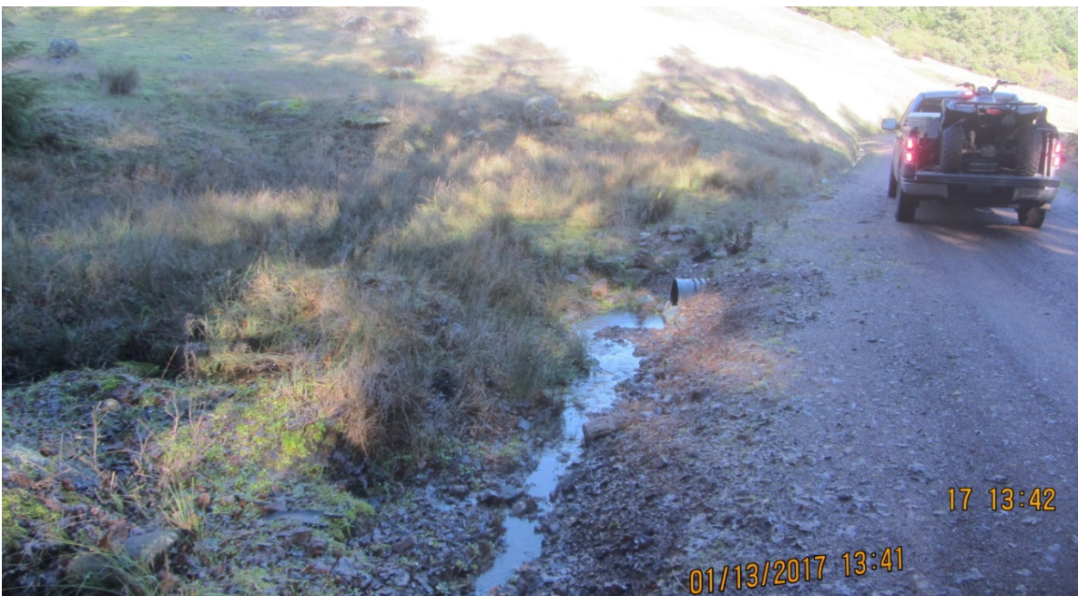
Image 49 shows Stream Crossing 16 inlet; note the connection of the inside ditch along the road to the culvert inlet. The road is constructed through a wetland in this location. (IMG 3092-3094 stitch)
