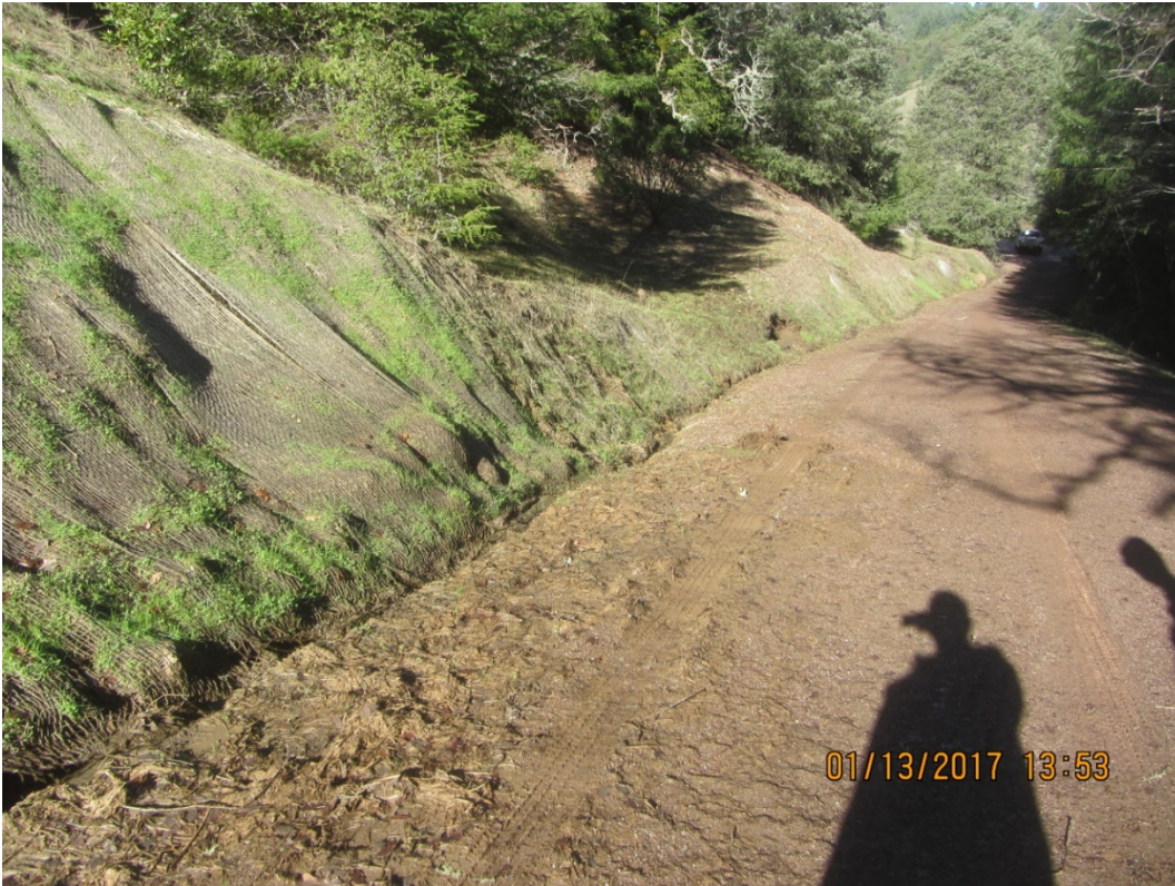
Image 55 shows a series of unstable cut banks on the approach to Stream Crossing 17. Note the long unbroken stretch of inside ditch. The truck in the distance is parked at the crossing.(IMG 3113)
