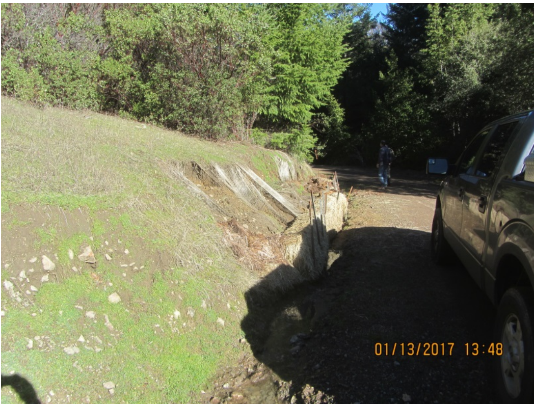
Image 53 shows one of several unstable cut banks on the approach to Stream Crossing 17. (IMG 3106)
