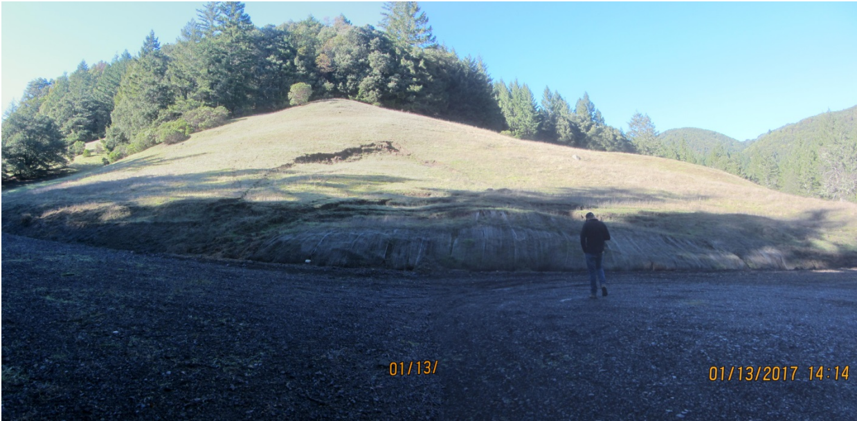
Image 66 shows inspection point Landslide 2 . (IMG 3150-3151 stitch)
