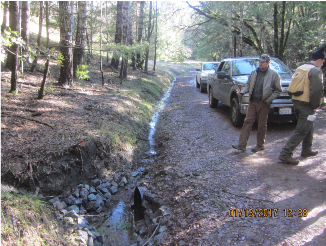
Image 27 shows the connection of the inside ditch to the stream at Stream Crossing 6. (IMG 3035)
