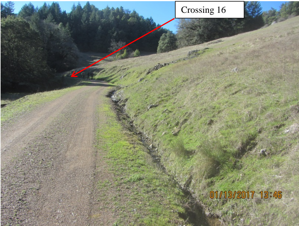
Image 52 shows the long extent of inside Ditch leading from Crossing 16 to an unstable cut bank above Ditch Relief Crossing 17. (IMG 3105)
