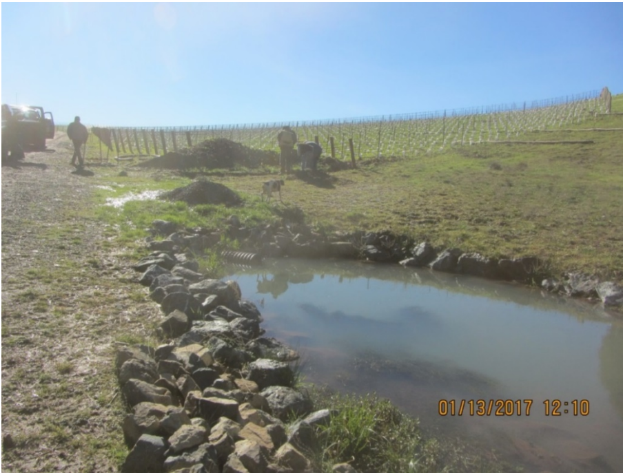
Image 14 looking due South shows the ditch intercepting the buried Class II stream in the background and a culvert leading from the developed vineyard to the detention basin installed in a Class II stream. The retention basin appears to be acting as a settling pond for sediment generated by ditch construction upstream. The road adjacent to the stream is also prone to surface erosion and likely generating sediment during rainfall. We observed that Rock fill appeared placed directly on wetland obligate plant species; Gil Falcone identified the species as sedges ( Carex ) and rushes ( Juncus ). (IMG 2982)
