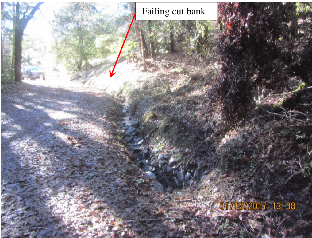
Image 47 shows the inside ditch and the failing cut bank connection. This ditch relief culvert corresponds to Crossing 14 in table 1. (IMG 3088)
