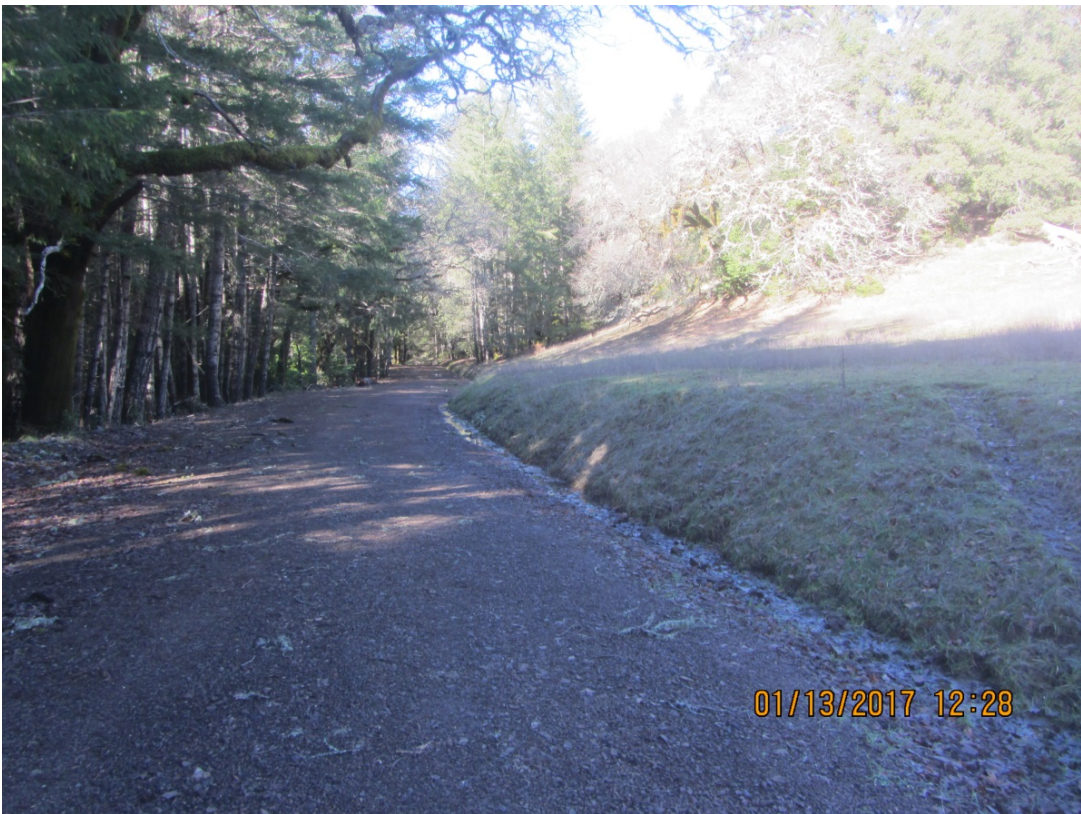
Image 24 shows the inside ditch North of Stream Crossing 4 – note the long length of uninterrupted ditch capturing road surface runoff. (IMG 3027)
