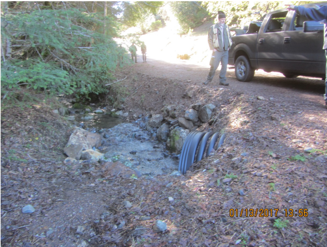
Image 56 shows the inlet of Stream Crossing 17 note the poor alignment of the inlet and the unstable cut bank in the background. (IMG 3117)
