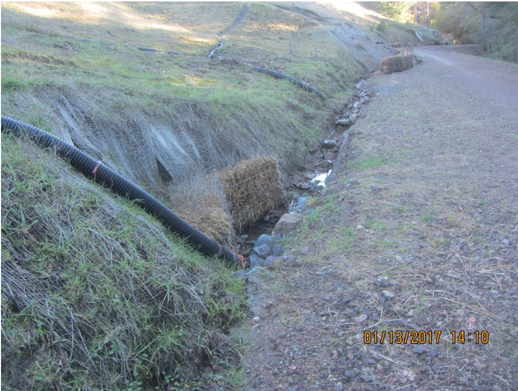
Image 62 shows the inside ditch along the road beneath a series of unstable slopes at inspection point Landslide 1. (IMG 3137)
