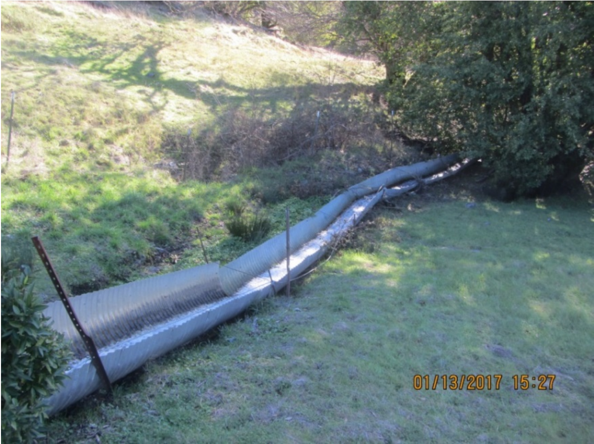
Image 72 shows the spillway of the pond located at GPS8. At the outlet of this structure there is about an 8' drop into an earthen channel that shows signs of down cutting and erosion. (IMG 3188)
