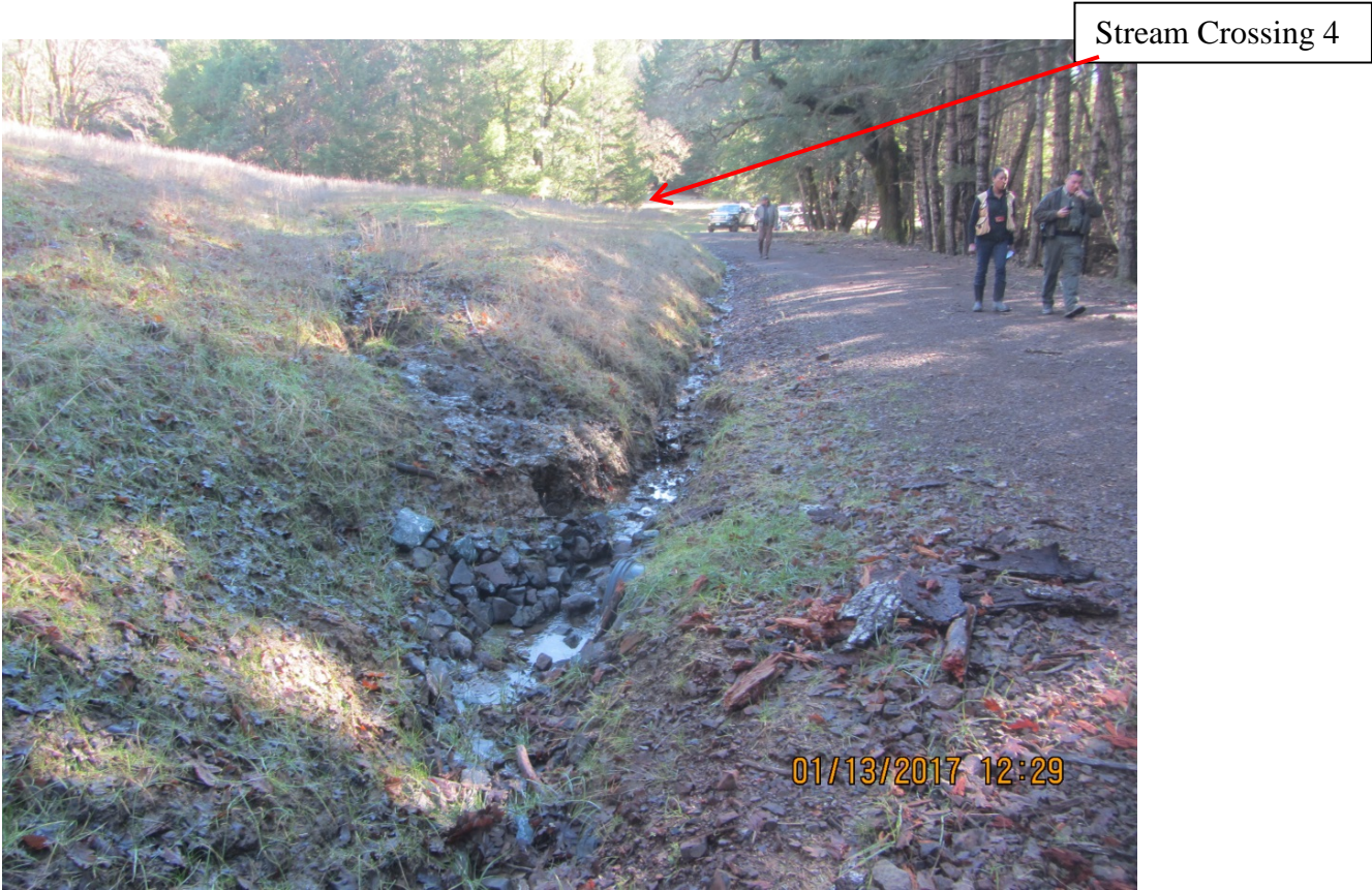
Image 25 shows the inside ditch intercepting a Class III stream originating upslope from a meadow area. (IMG 3030)
