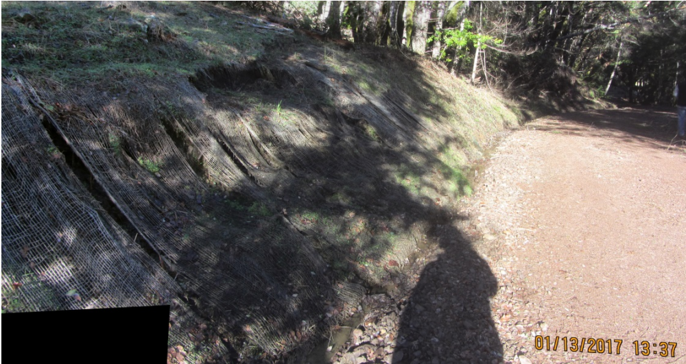
Image 46 shows the failing cut bank treated with jute netting. (IMG 3085-3086 stitch)
