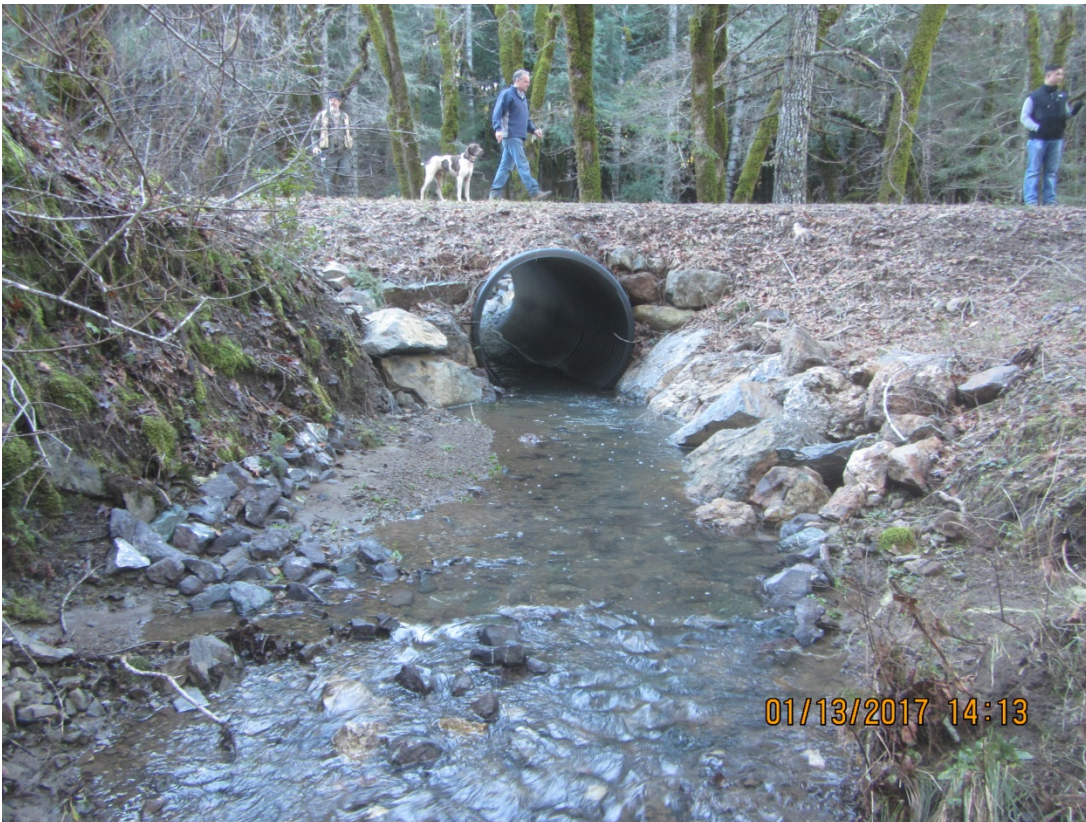
Image 65 shows the outlet of Stream Crossing 19 and rock fill placed in the stream. (IMG 3147)
