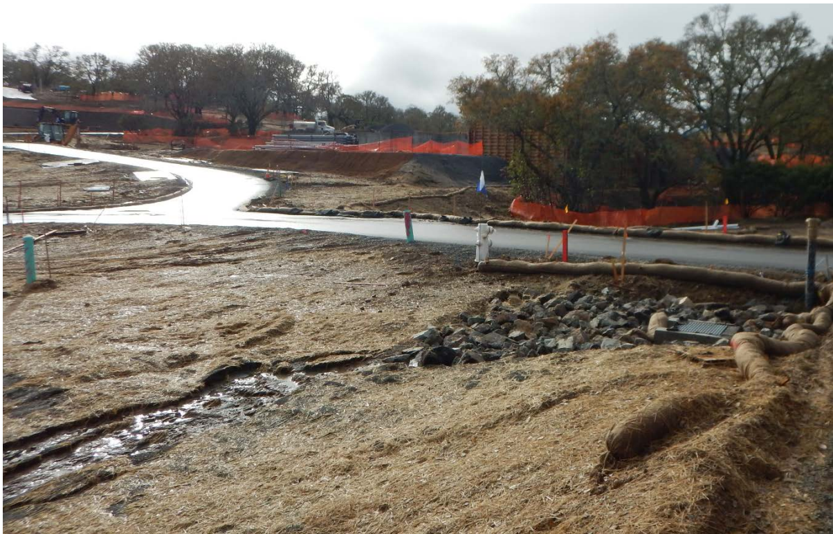
Picture 18 above. Resort Area. BMPs need maintenance and additional sediment controls. Storm water seems to be bypassing the DI causing additional erosion.
