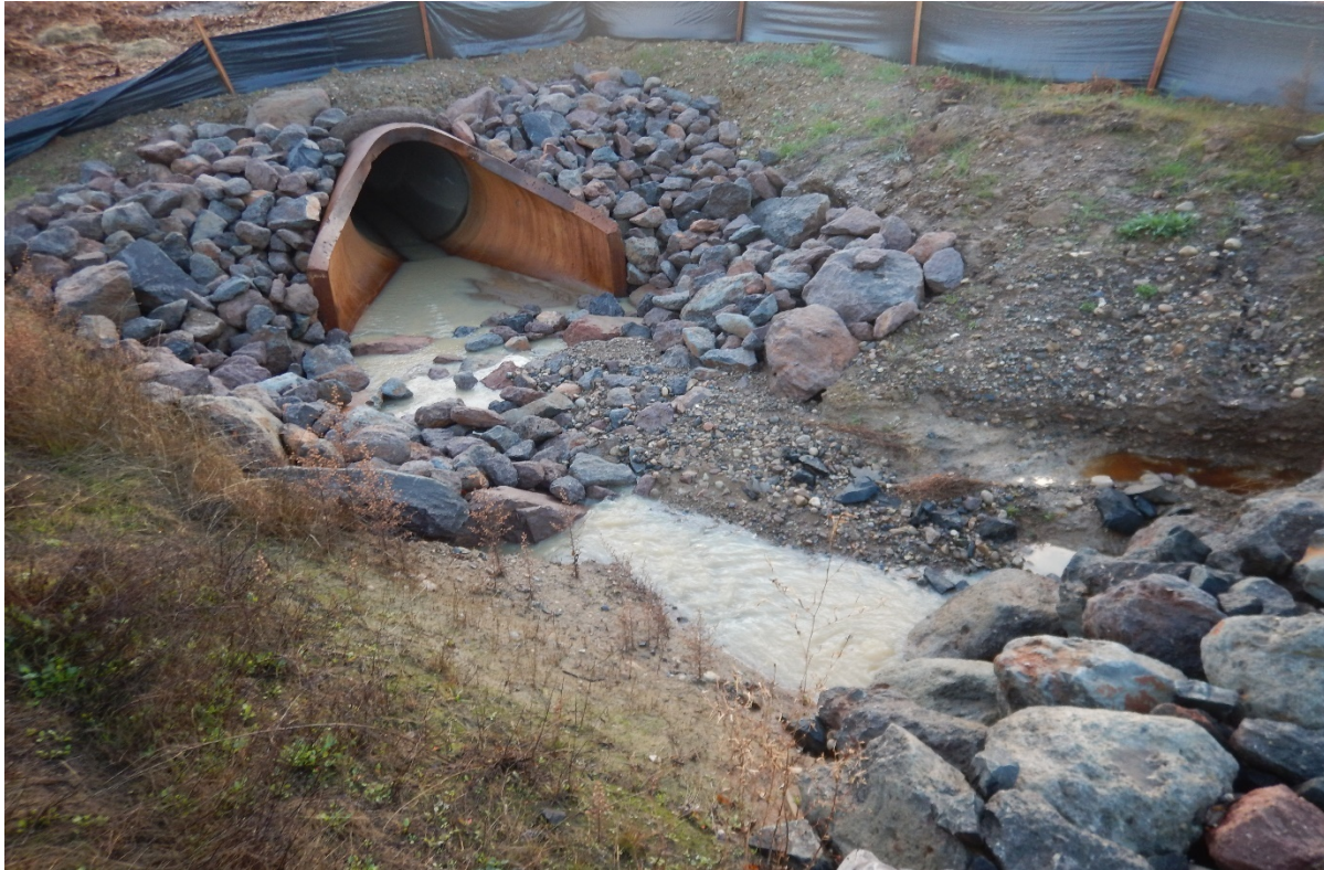
Picture 61 above. Shannon Road. Culvert inlet along Shannon Road that carries flows beneath Passalacqua Rd. Culvert outlets into Foss Creek.
