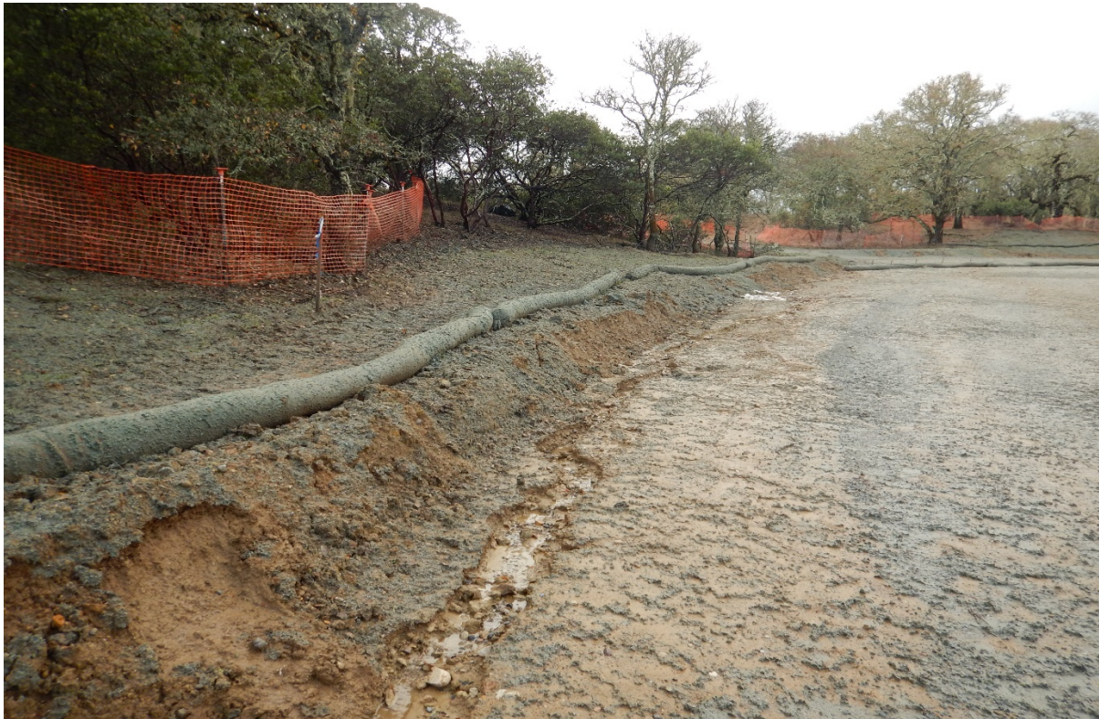
Picture 40 above. Road 8. Inadequate erosion and sediment controls.
