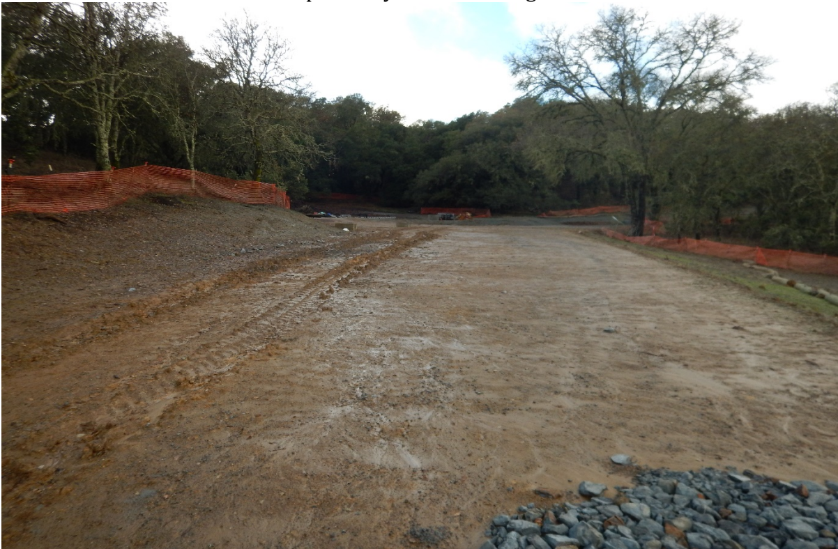
Picture 38 above. Road 8. Sections of road with no erosion and sediment controls.
