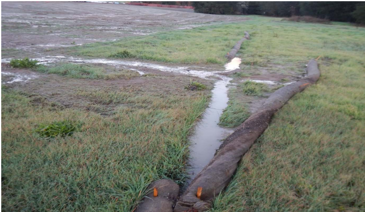
Picture 4 above shows wattles displaced by the storm water flowing off the construction Site towards the City's detention basin.
