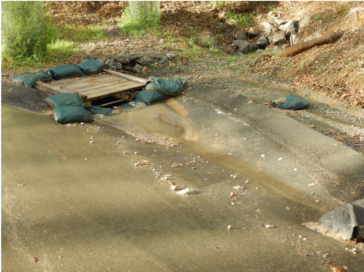
Picture 34 above. Shannon Road. BMPs overwhelmed and in need of maintenance. Sediment discharge to DI.
