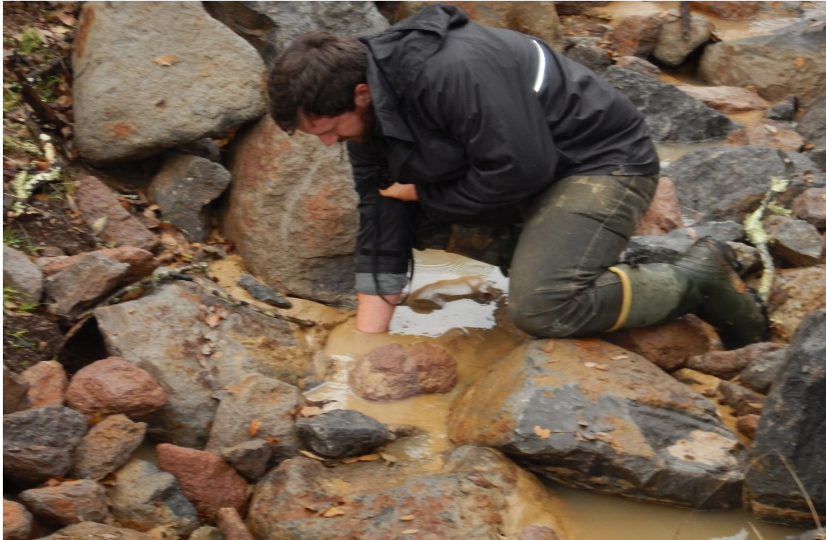
Picture 43 above. Road 8. Large quantities of fine sediment discharged to waters from upstream culvert installation.
