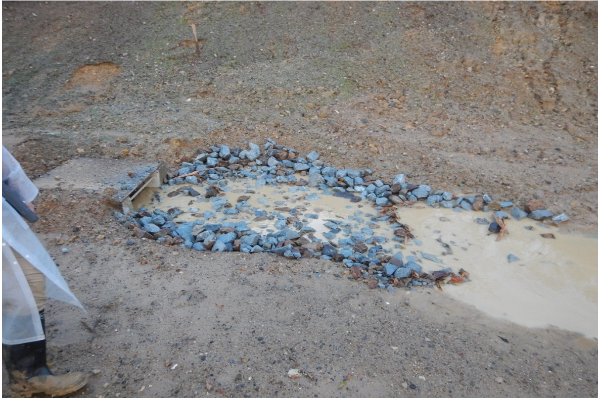
Picture 55 above. Road 5. Inadequate erosion and sediment controls. Discharge of sediment and turbid water to DI.
