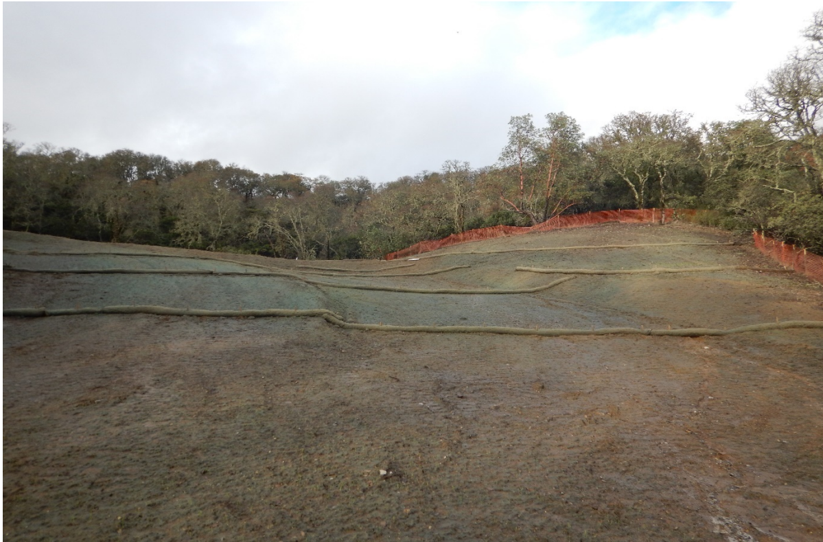
Picture 35 above. Road 8. BMPs present yet there are signs of erosion.
