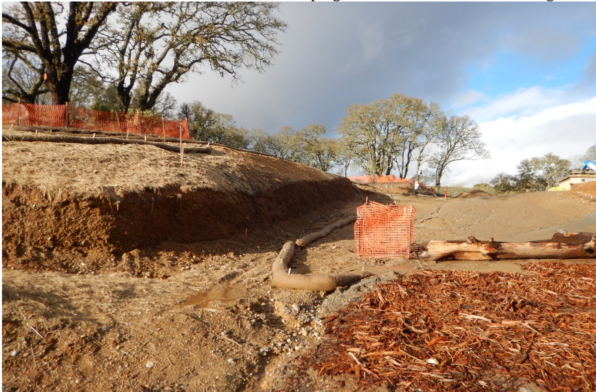
Picture 32 above. Shannon Road. Inadequate erosion and sediment controls.
