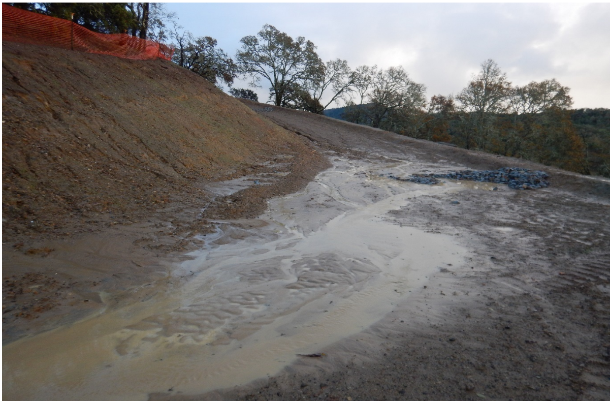
Picture 56 above. Road 5. Inadequate erosion and sediment controls resulting in significant erosion and downstream sedimentation.
