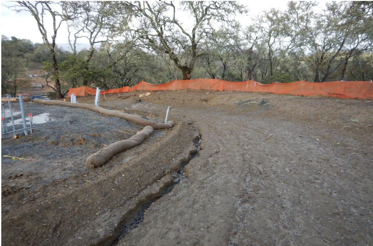
Picture 22 above. Resort Area. Inadequate erosion and sediment controls.
