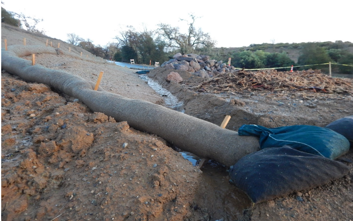
Picture 63 above. Drainage from Passalacqua Rd. Inadequate BMPs. Storm water flows have eroded the tow of the slope and undermined BMPs resulting in discharge to waters.
