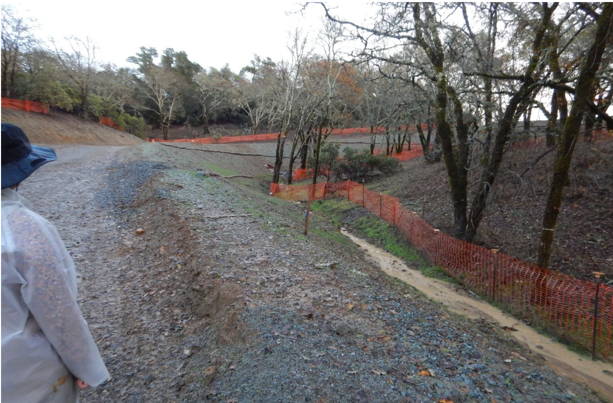
Picture 53 above. Road 5. Inadequate erosion and sediment controls.
