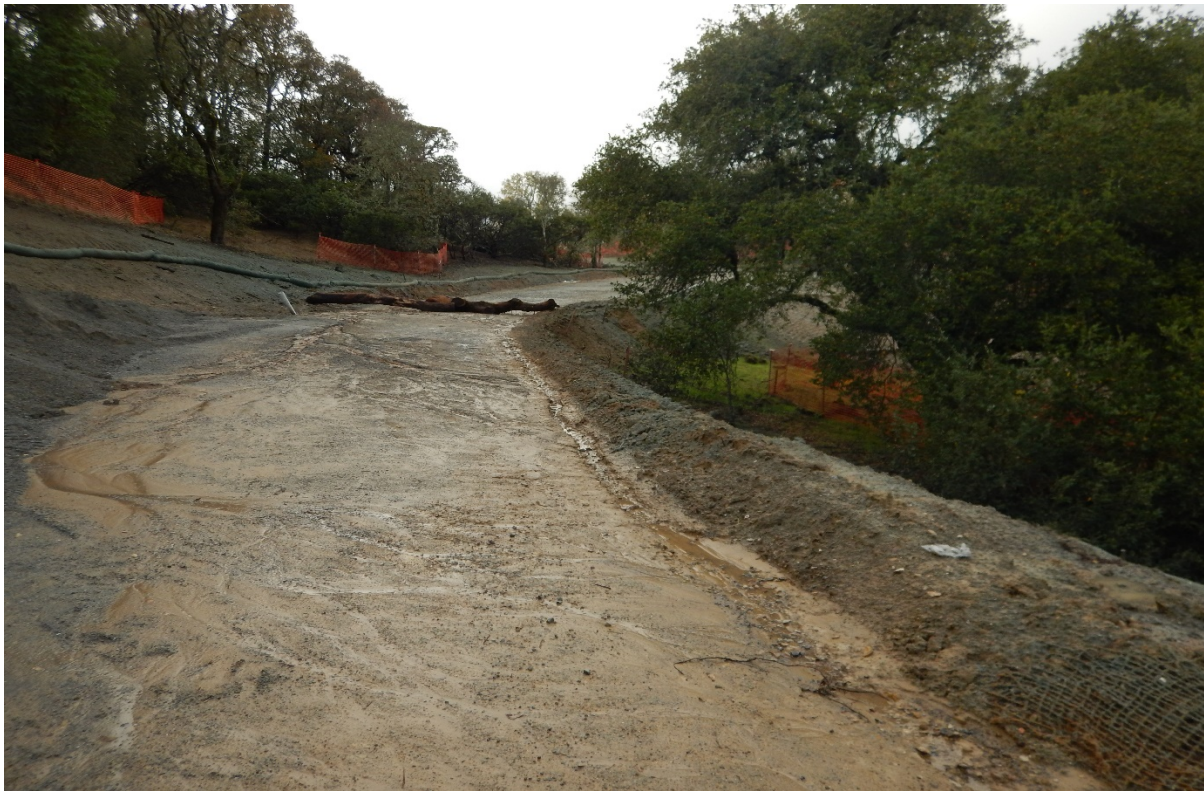
Picture 39 above. Road 8. Sections of road with no erosion and sediment controls.
