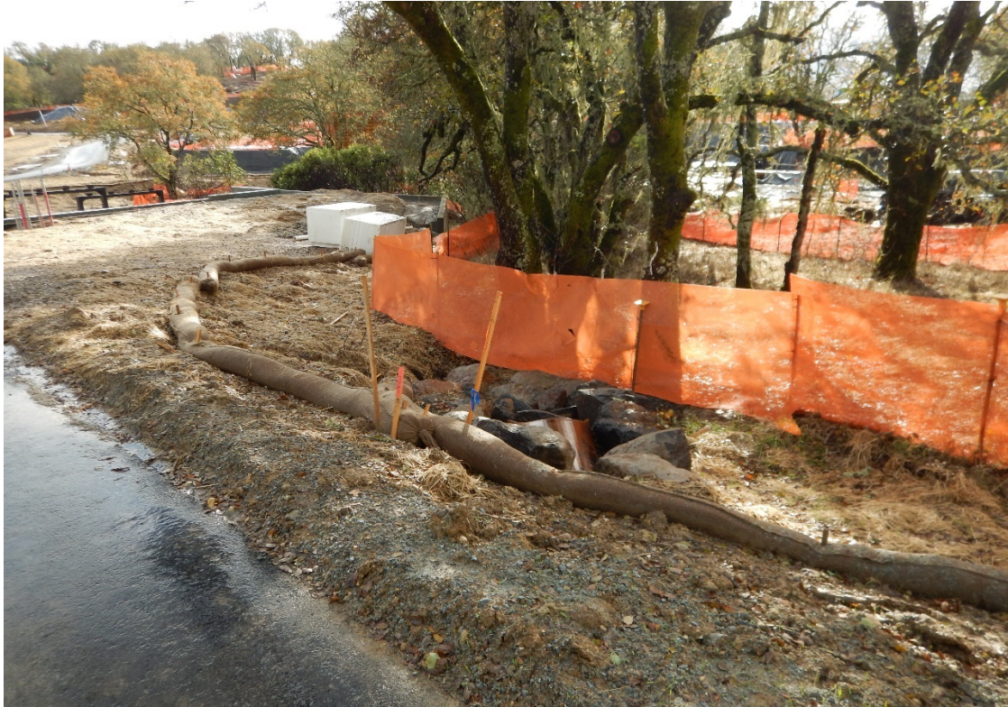
Picture 5 Above. Resort Area. Image show erosion and sediment controls with environmental sensitive area (ESA) fencing.
