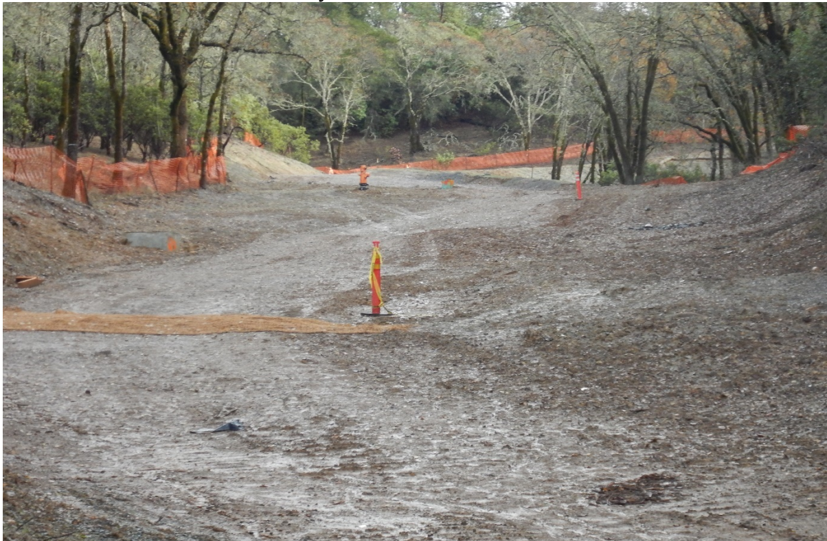
Picture 52 above. Road 5. Inadequate erosion and sediment controls.
