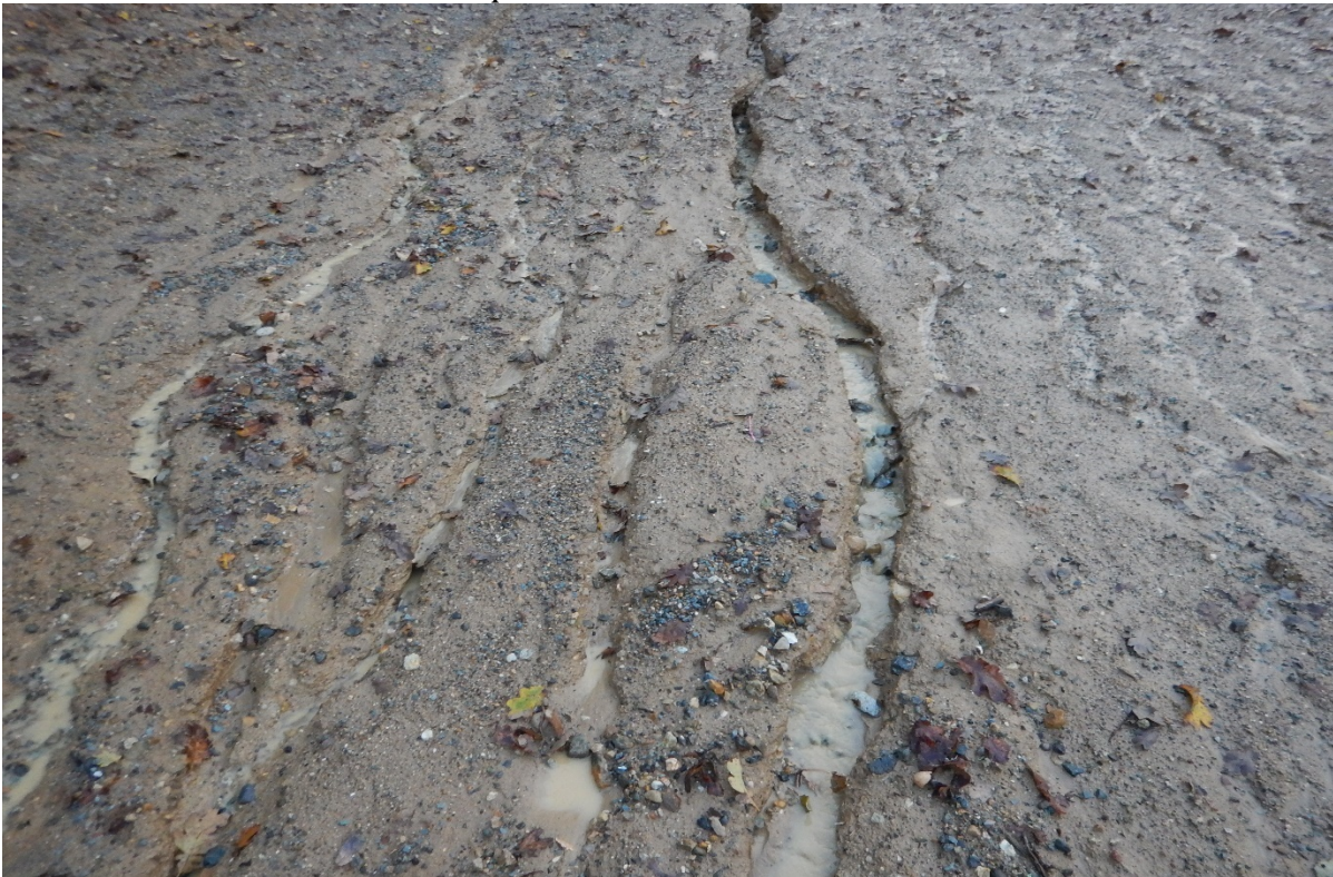
Picture 54 above. Road 5. Inadequate erosion and sediment controls. Rills indicating sediment transport.
