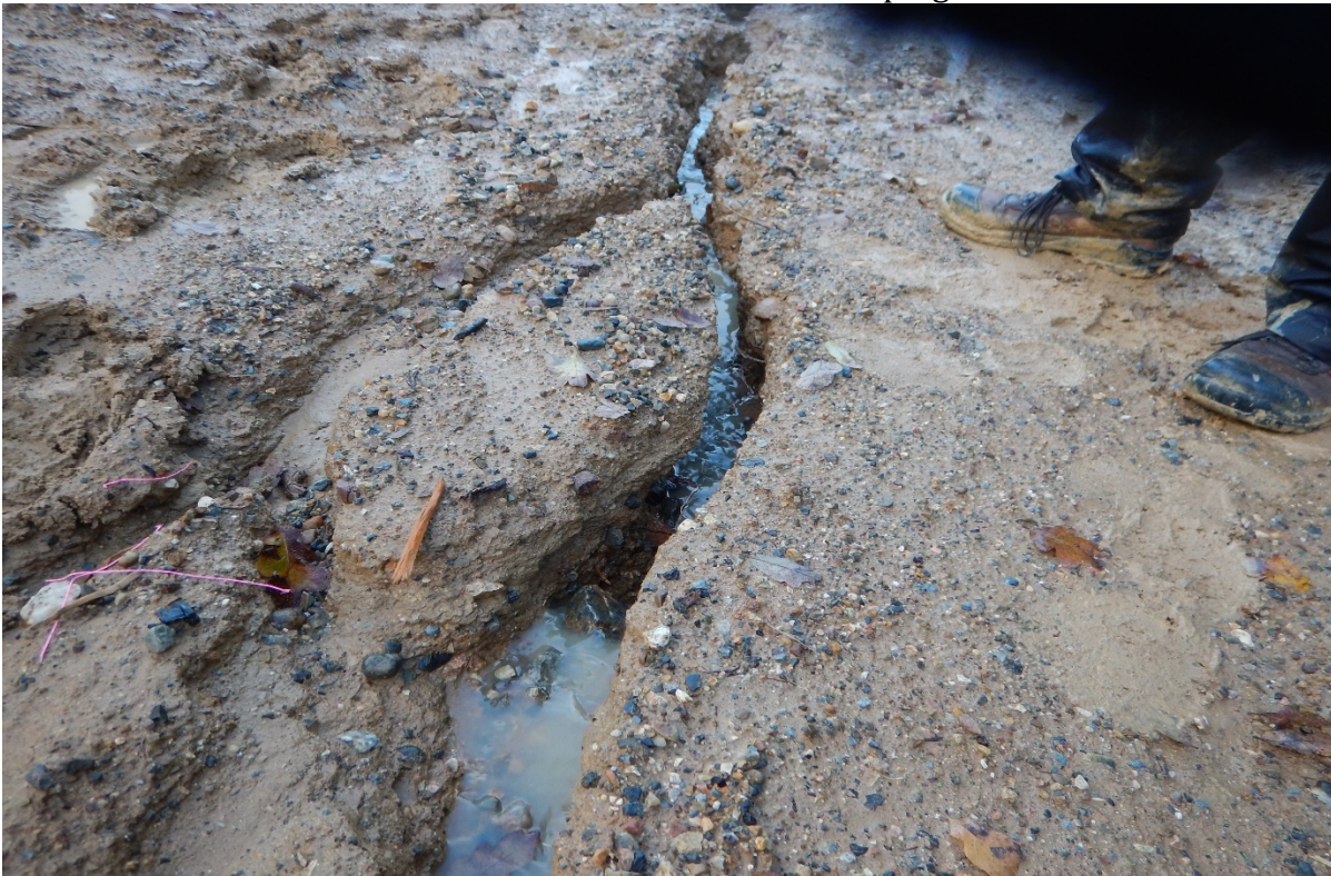
Picture 58 above. Road 5. Inadequate erosion and sediment controls. Rills indicating sediment transport.
