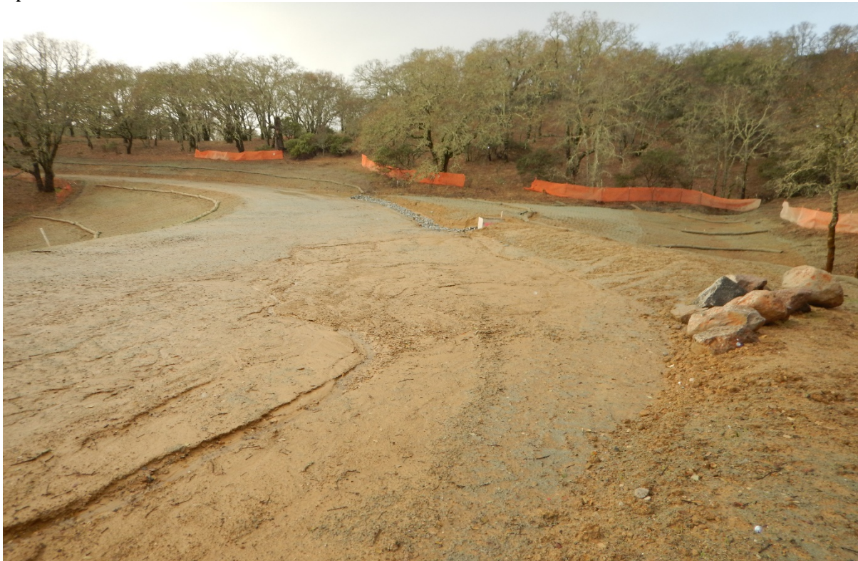
Picture 44 above. Road 8. Inadequate erosion and sediment controls at the newly installed stream crossing.
