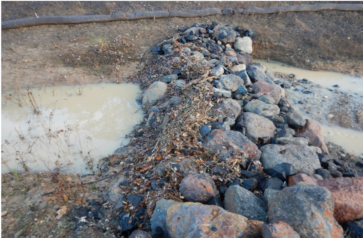
Picture 60 above. Shannon Road. Rack line of debris indicates flows overtopping BMPs and depositing fine sediment and debris downstream.
