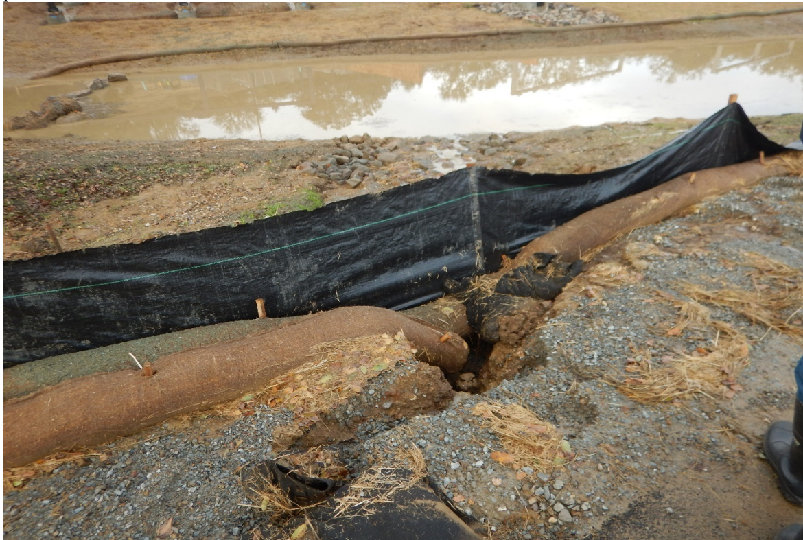
Picture 12 above. Resort Area. More evidence of BMPs needing maintenance that were unable to handle storm water flows.
