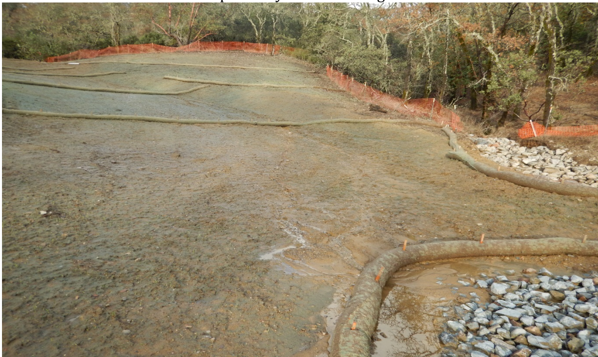
Picture 36 above. Road 8. BMPs present yet there are signs of erosion.
