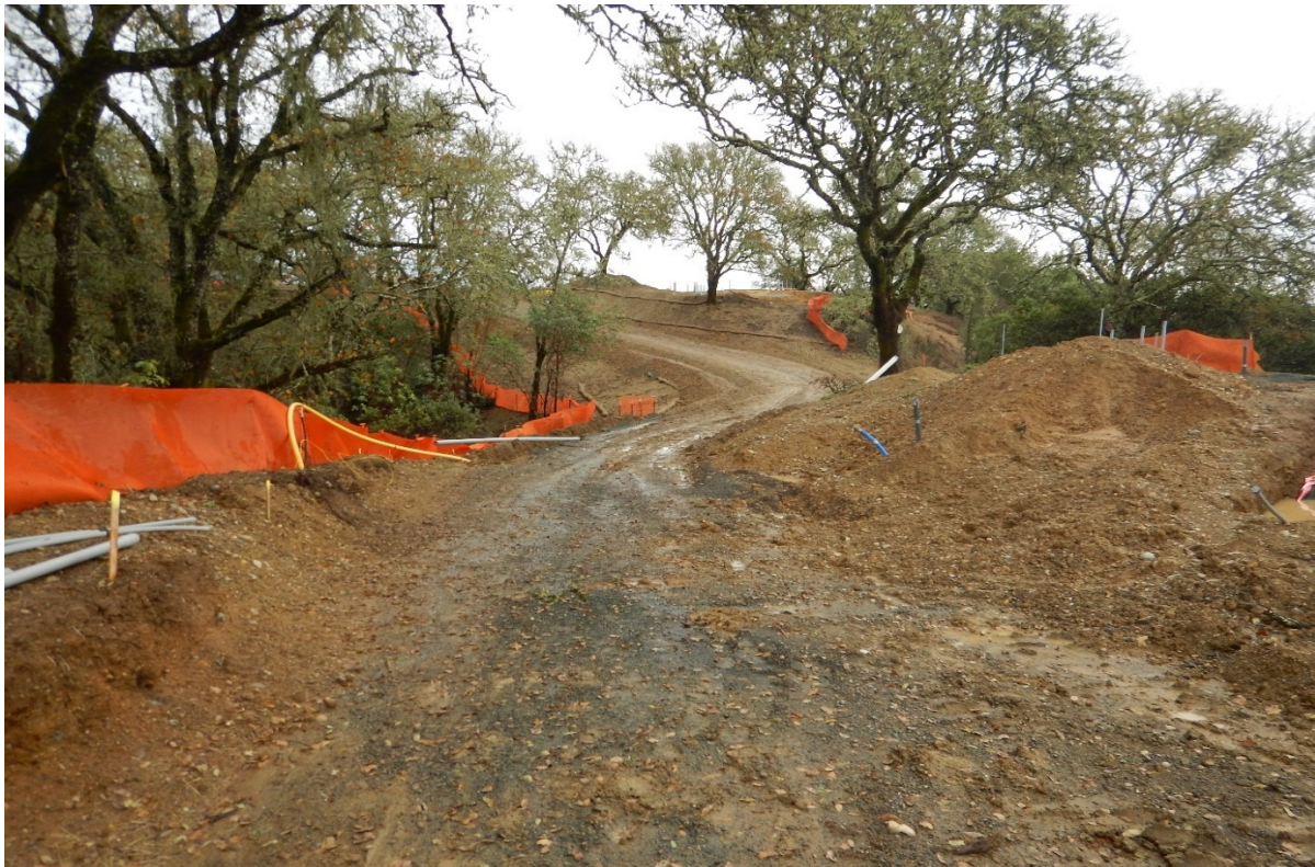
Picture 19 above. Resort Area. Inadequate erosion and sediment controls.
