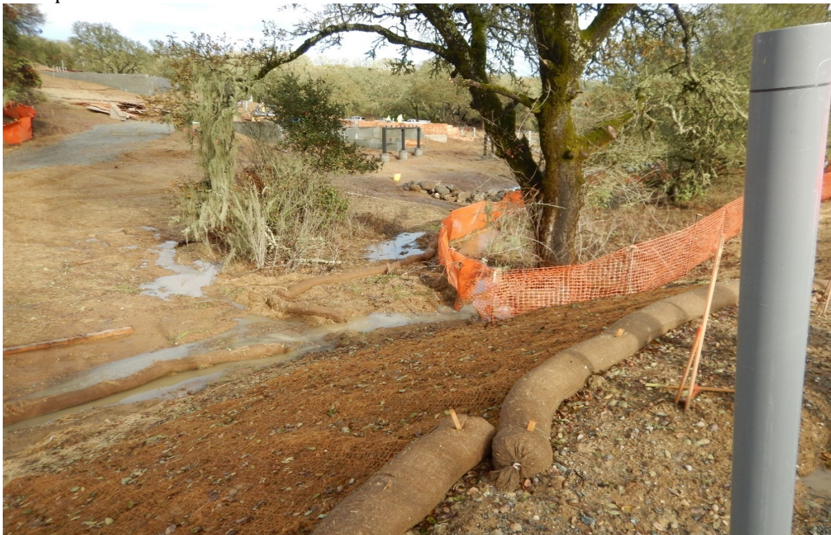
Picture 10 above. Resort Area. BMP maintenance is needed: many areas are overwhelmed by flows.
