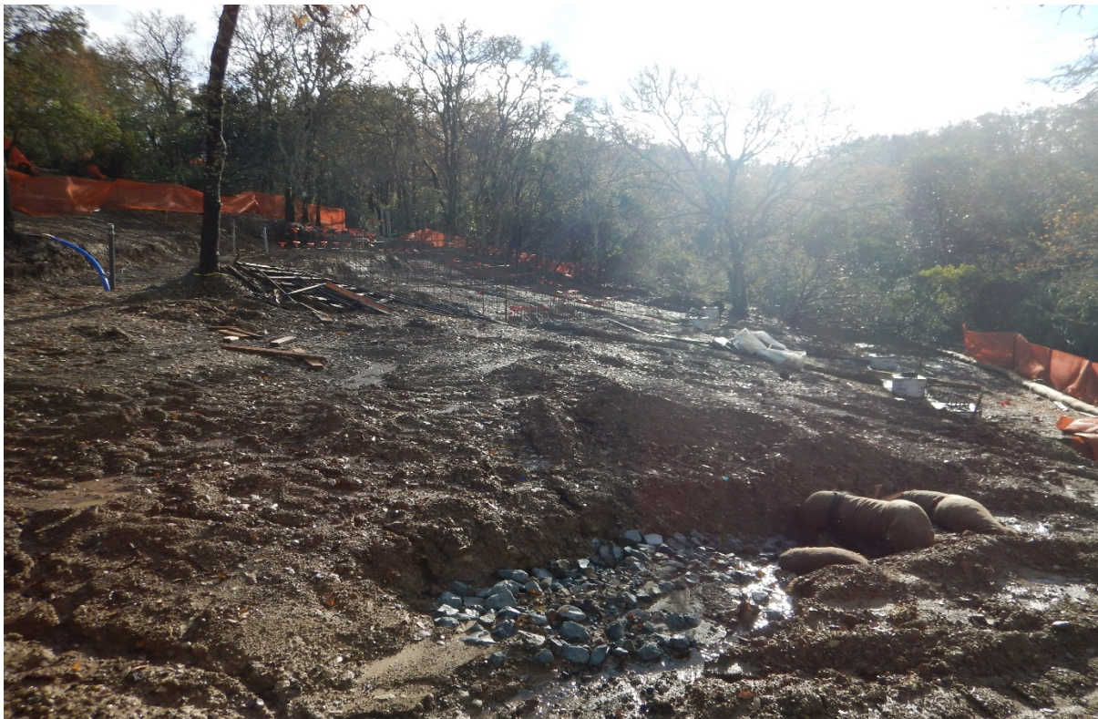
Picture 24 above. Resort Area. Inadequate erosion and sediment controls. Discharge to drain inlet.
