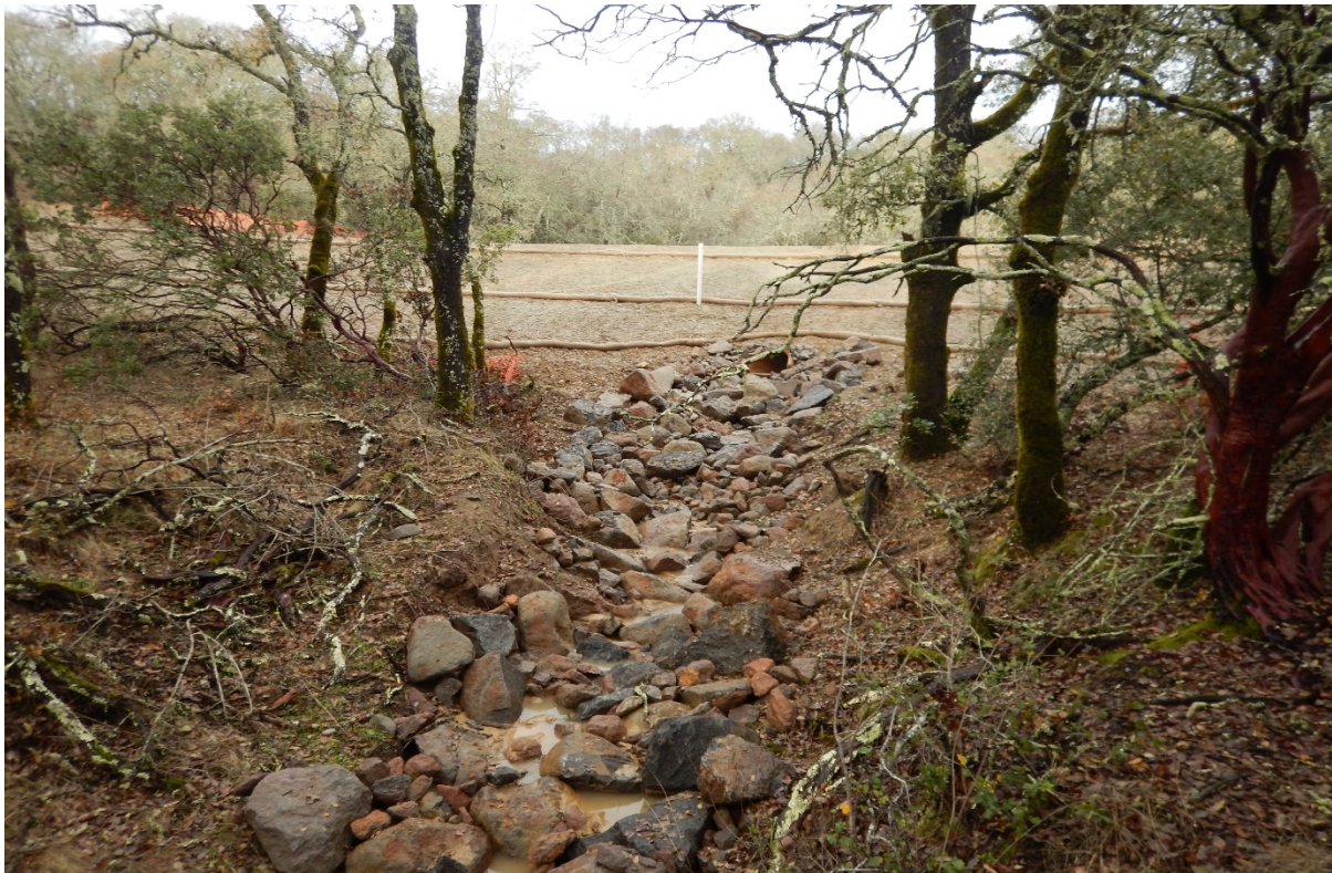
Picture 41 above. Road 8. Culvert outfall with turbid water and fine sediment discharge.
