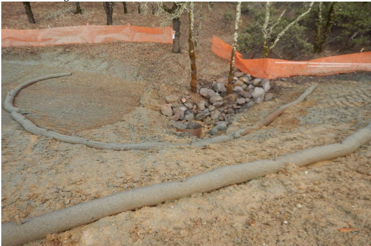
Picture 46 above. Road 8. Inadequate erosion and sediment controls at the newly installed stream crossing.
