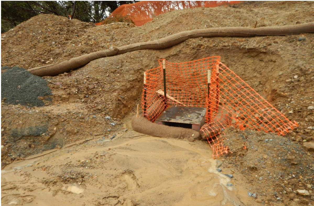
Picture 20 above. Resort Area. Inadequate erosion and sediment controls. Sediment discharge to drain inlet.
