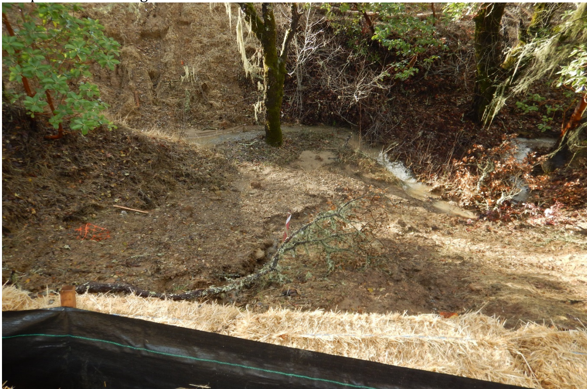
Picture 26 above. Resort Area. Inadequate erosion and sediment controls. BMPs were compromised leading to bank erosion.
