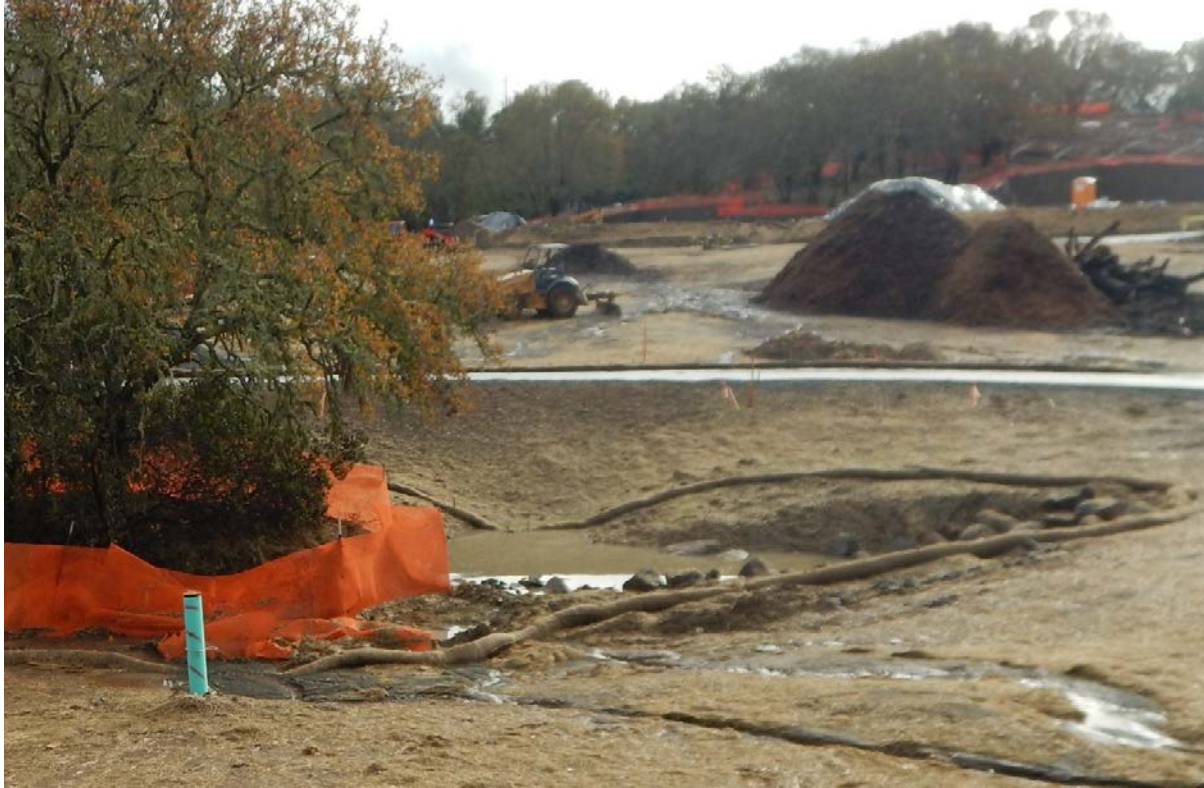
Picture 17 above. Resort Area. BMPs need maintenance and additional sediment controls.
