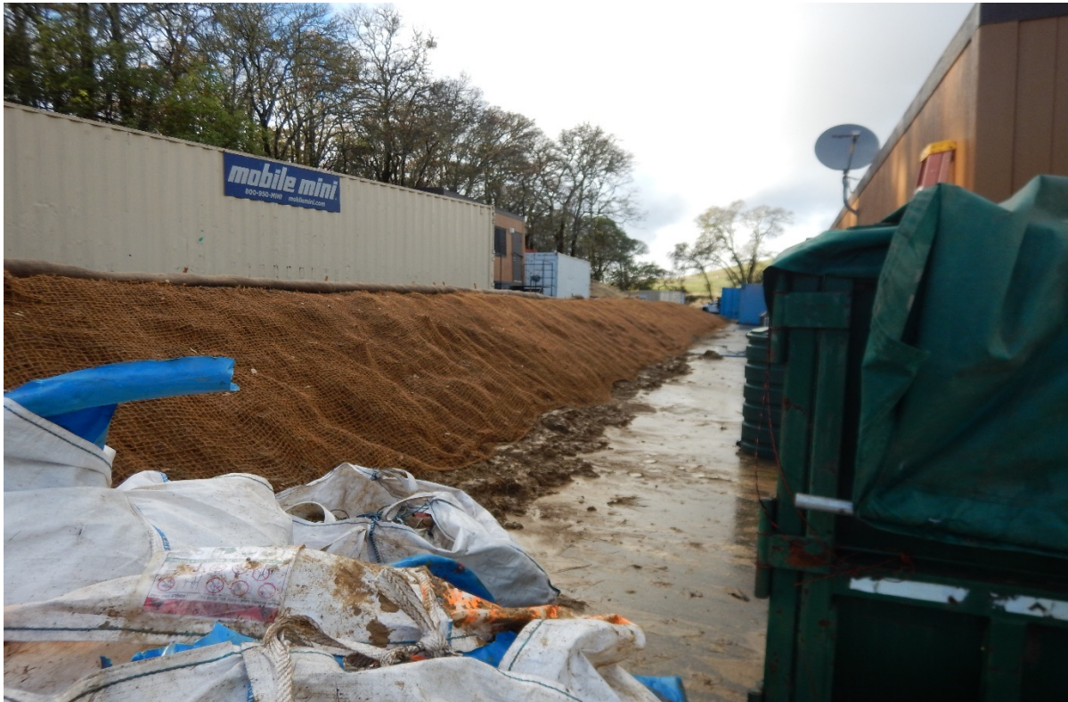
Picture 30 above. Resort Area. BMPs maintenance needed.
