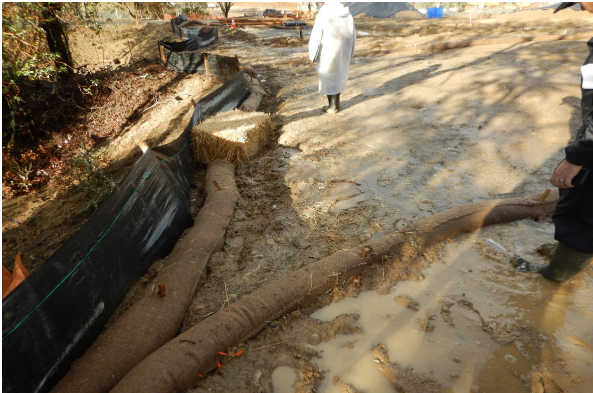
Picture 25 above. Resort Area. Inadequate erosion and sediment controls. BMPs were compromised leading to bank erosion.
