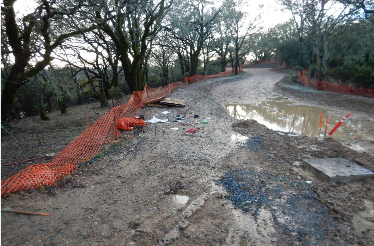
Picture 57 above. Road 5. Trash left onSite. Poor housekeeping.
