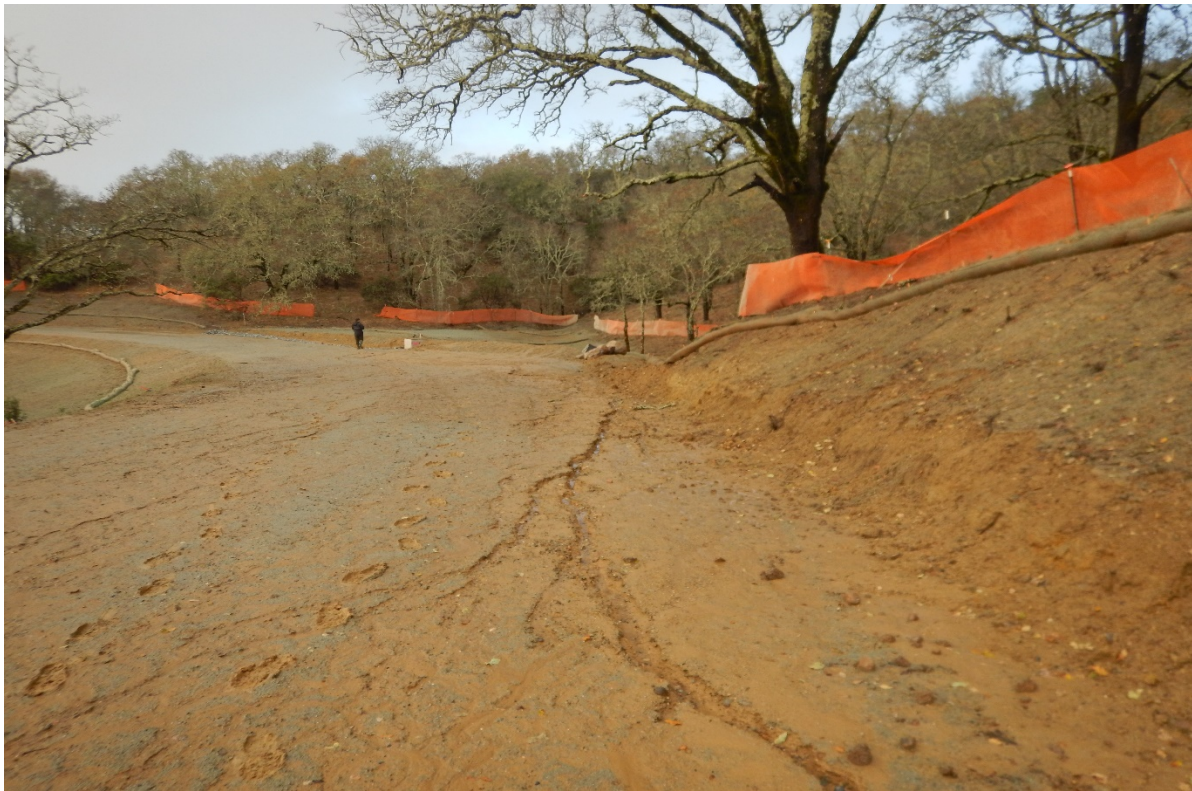
Picture 45 above. Road 8. Inadequate erosion and sediment controls at the newly installed stream crossing.
