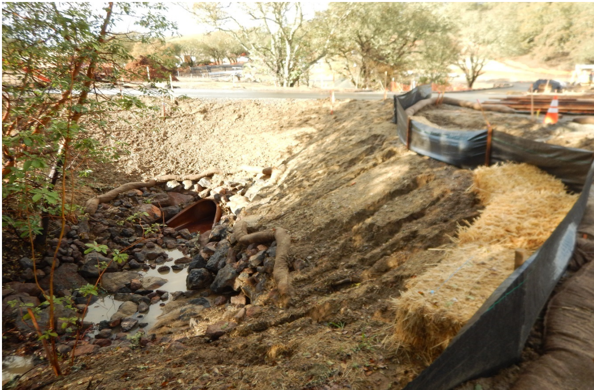
Picture 27 above. Resort Area. Inadequate erosion and sediment controls. BMPs were compromised leading to bank erosion.
