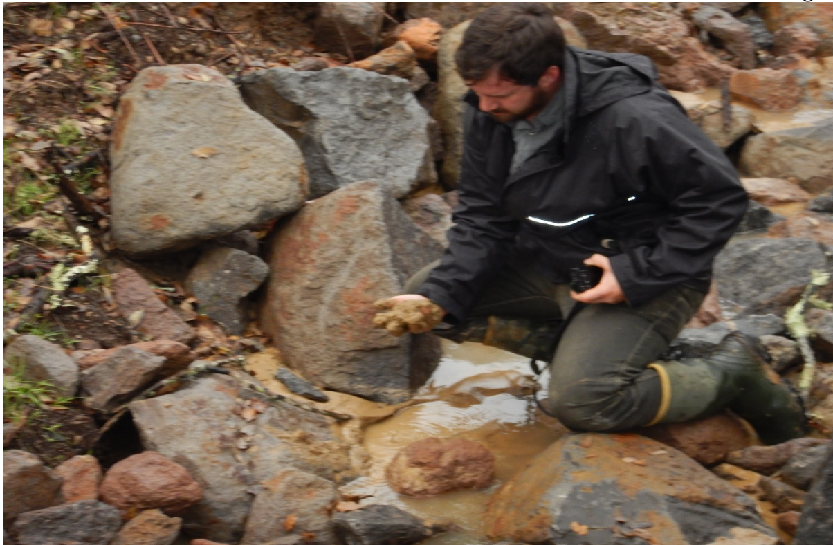
Picture 42 above. Road 8. Large quantities of fine sediment discharged to waters from upstream culvert installation.
