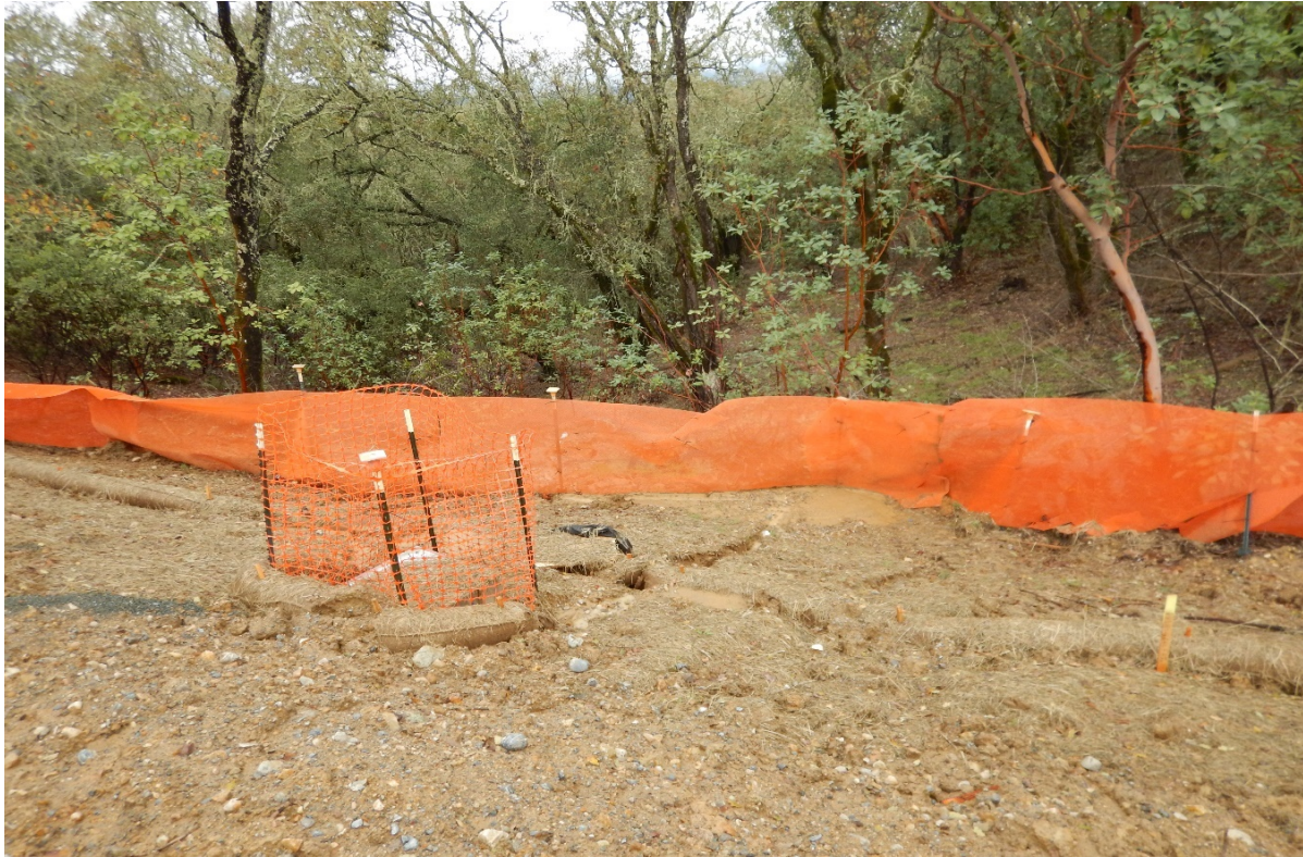
Picture 21 above. Resort Area. Inadequate erosion and sediment controls.
