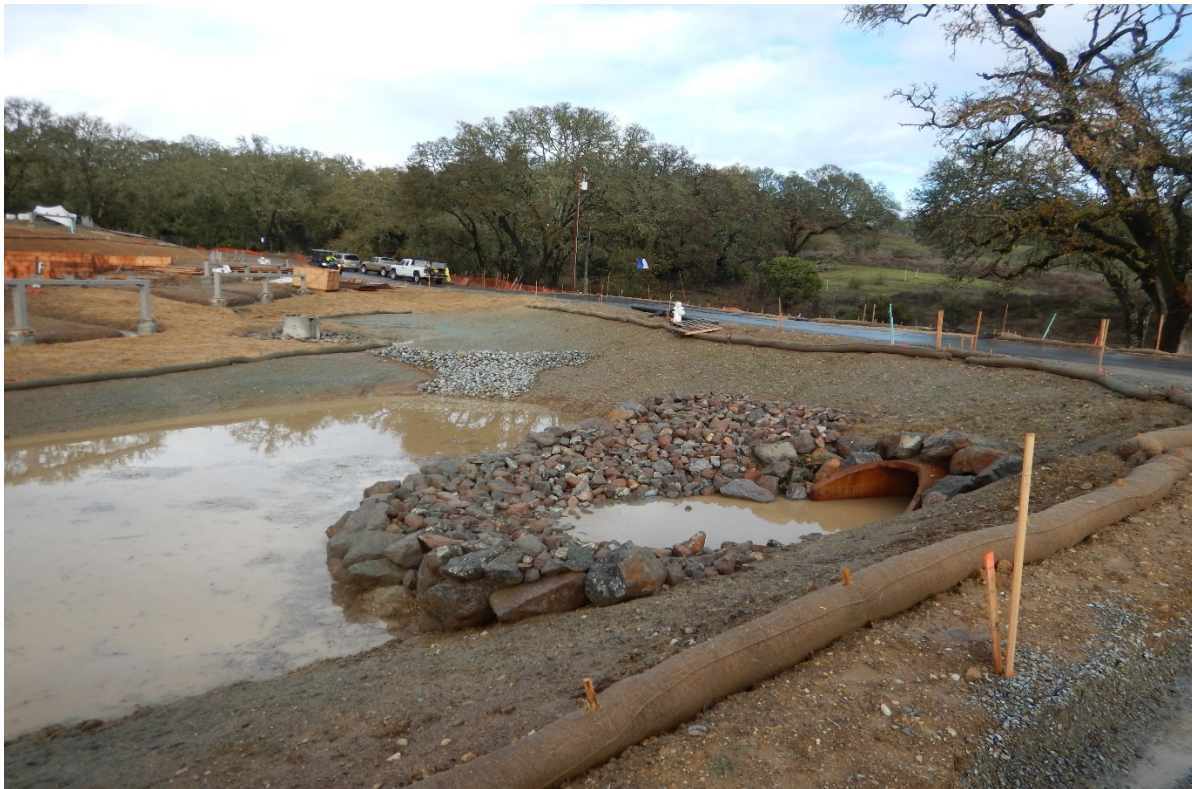
Picture 13 above. Resort Area. Instream sediment basin.
