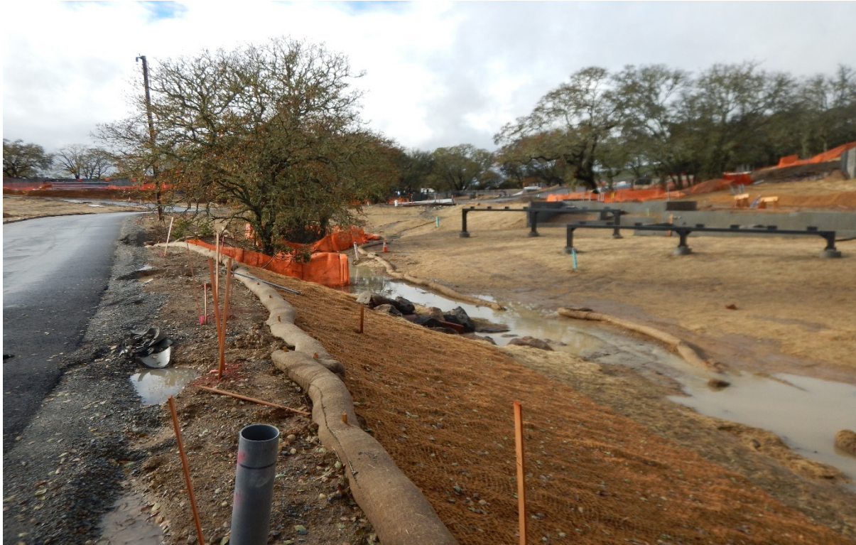
Picture 9 above. Resort Area. Shows waters of the state with BMPs along slopes and creek banks. BMP maintenance is needed: many areas are overwhelmed by flows. Straw appears to be placed in waters.
