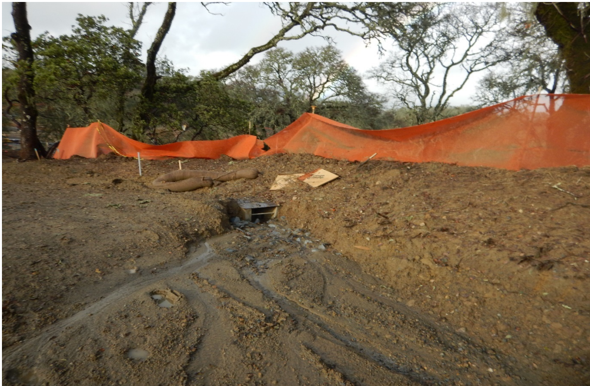
Picture 23 above. Resort Area. Inadequate erosion and sediment controls. Discharge to drain inlet.
