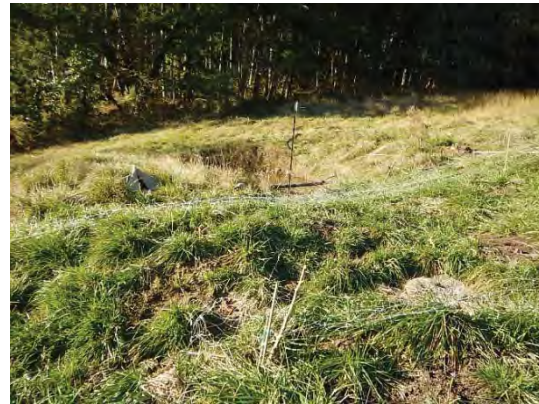
Figure 10. Small excavated area and berm in the wet slope. I observed ponded water, apparently due to hillside seepage from the wetland. This feature does not have a controlled outlet structure. The berm is small and well-vegetated. I did not observe evidence of erosion at the pond. Vegetation indicated fluctuating water levels.
