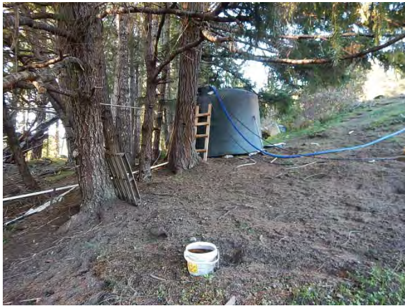
Figure 19. Water storage tank on an incline.
