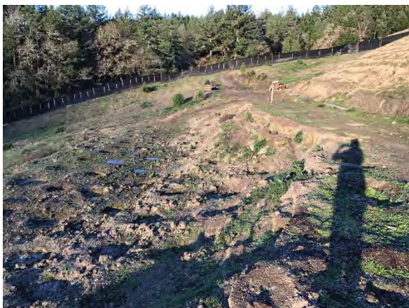
Figure 25. Fill failure on terraces at WQ-7.
