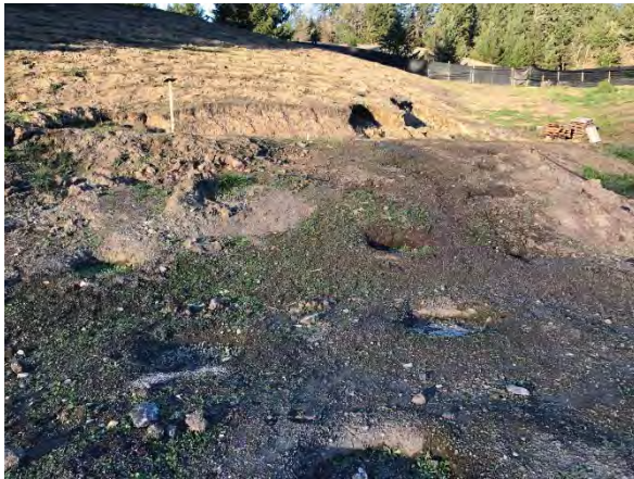
Figure 24. Cut bank failure at WQ-7.
