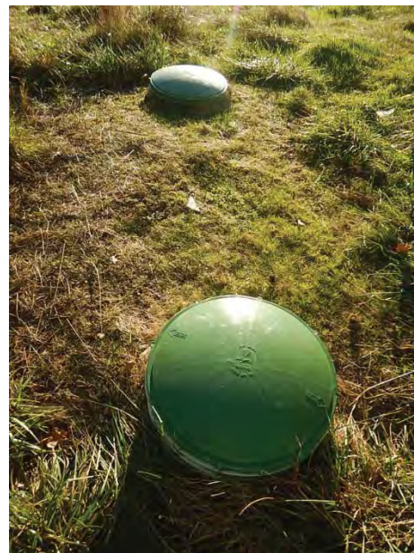
Figure 17. A septic tank adjacent to the house.
