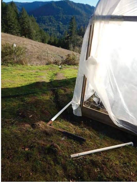
Figure 7. A ditch along the backside of the greenhouse runs directly to the nearby watercourse.
