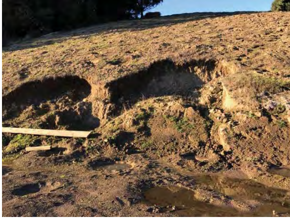
Figure 23. Two graded flat areas on the hillside. The cuts appear oversteepened, with emergent water, showing evidence of developing unstable features/conditions. Water has collected on the flats and the cultivation holes are saturated (WQ-7).
