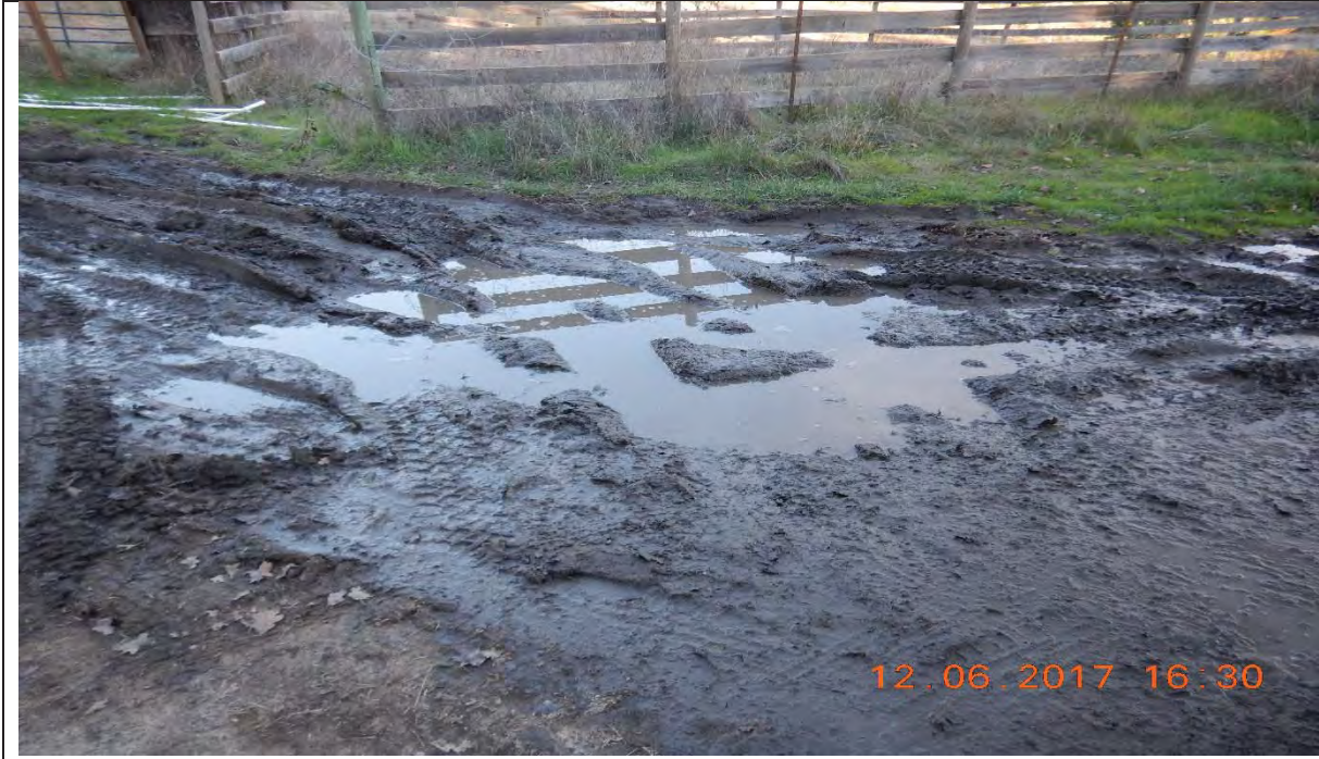
Photo 4. Ponded water on the road.
