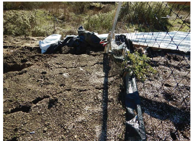
Figure 30. Another view of the fill failure along the southern side of.
