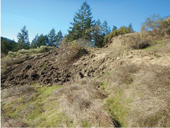
Figure 26. The flat between WQ-6 & WQ-7 is constructed with earthen material that has been pushed over the break in slope and within 20 feet of a class II watercourse associated with the slide.
