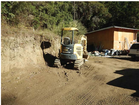
Figure 10. A mini excavator on the property, made by Komatsu Ltd, Model number PC27MP-2, and serial number 15587. The equipment was likely used in the recent earthwork observed on the property.
