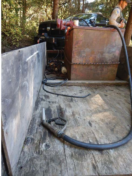
Figure 9. Generator and fuel tank located on property near the structure.
