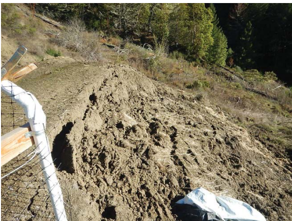
Figure 28. Fill failure along the southern side of the flat; this extends into greenhouse indicating potential discharge of potting soil and residual nutrients and chemicals.
