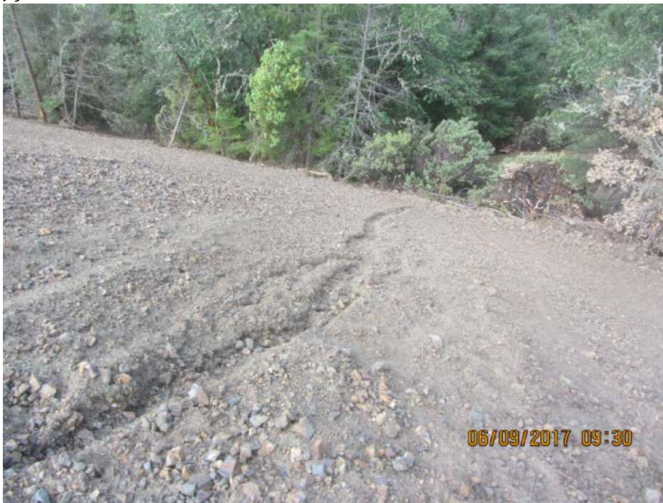
Figure 12: A 200-foot long rill has formed on the fill slope. (IMG_4094 S. Feiler)
