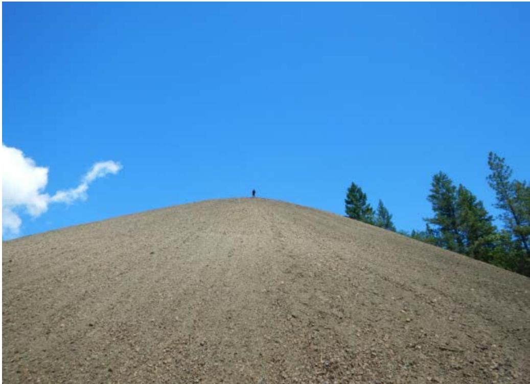
Figure 13: Looking up from WP-173 to the top of the expanded pad. The person standing at the top is approximately six feet tall (DSCN1285 Luders, J.).
