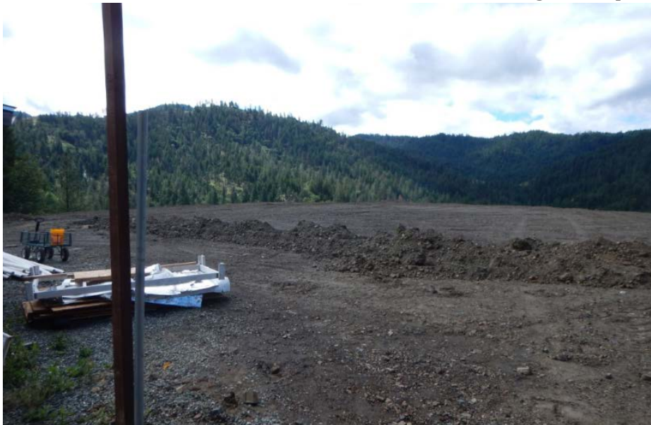
Figure 9: Recently constructed 11,200 square foot earthen pad expansion area. Note trench crossing the pad, possibly intended for placement of the irrigation pipe visible on the left (DSCN1211 Luders, J.).
