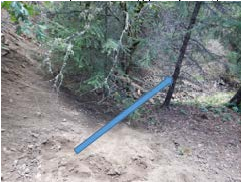
Figure 22: Blue line shows approximate historic alignment of the channel downstream of the roadway. Fill material placed in the stream channel is likely to fail and travel or be transported downstream during the winter period. View from WP-175 (DSCN1294 Luders, J.) (Edited by Luders, J.).
