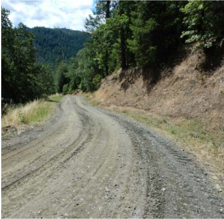
Figure 24: Access road is insloped into a ditch that concentrates surface runoff to a ditch relief culvert visible below, which then drains downhill from the road into an adjacent drainage area. View from WP-170 (DSCN1269 Luders, J.)
