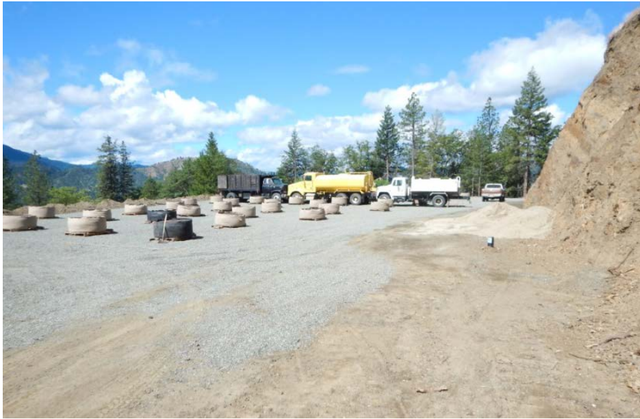
Figure 23: Fabric planters on the large earthen pad on the excavated ridgeline. WP-164 is located near the leftmost fabric planter pot visible in the photo (DSCN1236 Luders, J.).
