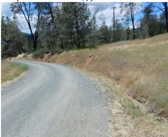
Figure 29: Inside ditch along the road that carries flows from the intercepted Class III watercourse (Figure 28) to an adjacent watershed beyond the ridge (DSCN1307 Luders, J.).
