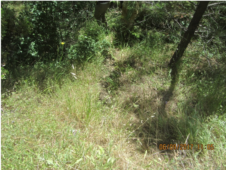
Figure 26: Slope below the ditch relief culvert outlet. An erosional channel is visible among the grasses. (IMG 4212 S. Feiler)
