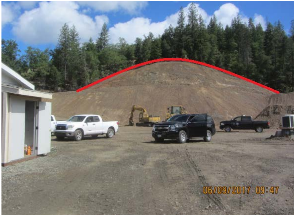
Figure 7: Ridgeline cut back to increase the size of the pad. The red line indicates the original contour of the ridge that had previously extended downhill towards the house. There is a terrace wide enough to drive a vehicle, midway up the cut face (IMG_4117 S. Feiler) (Edited by Luders, J.).
