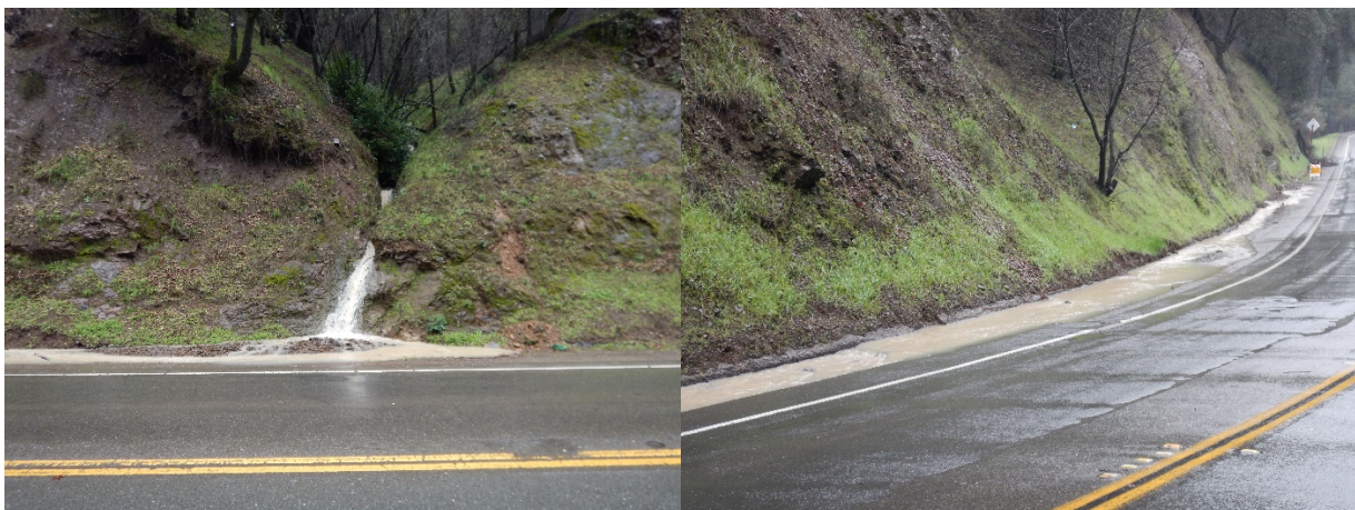
Photos 3 and 4: View of eastern drainage. Water bypassing drop inlet and flowing along roadway. Photographed by Paul Nelson.
