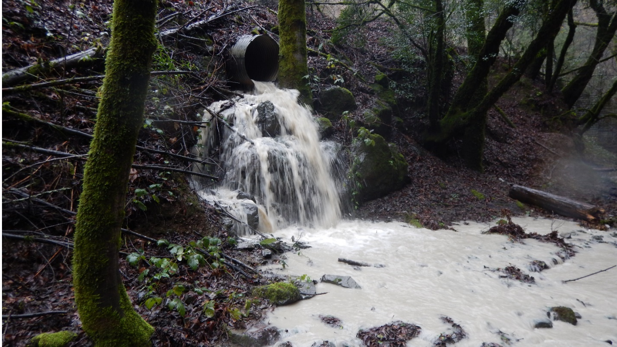
Photo 2: East culvert discharge to Porter Creek looking south from Porter Creek Road. Elevated sediment content is evident in the discharging water and confirmed by the analytical results. Photographed by Paul Nelson.
