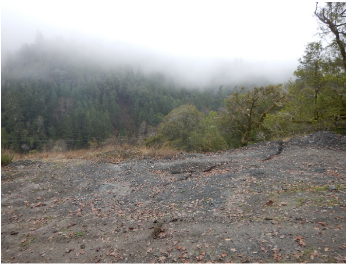
Photo 15: Cracking in road below pond berm adjacent to the Class II watercourse (DSCN4326)
