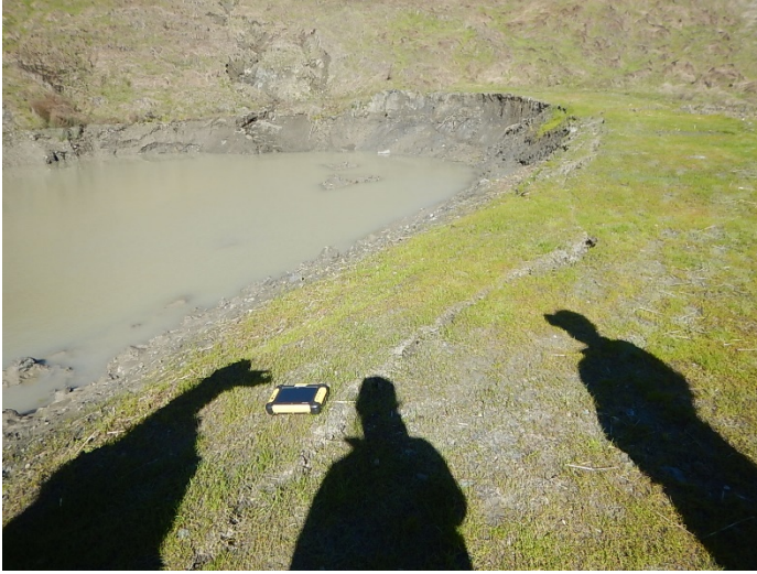
Photo 13: Cracking in exterior pond berm face (DSCN9357 photo taken by Adona White, February 18, 2019)
