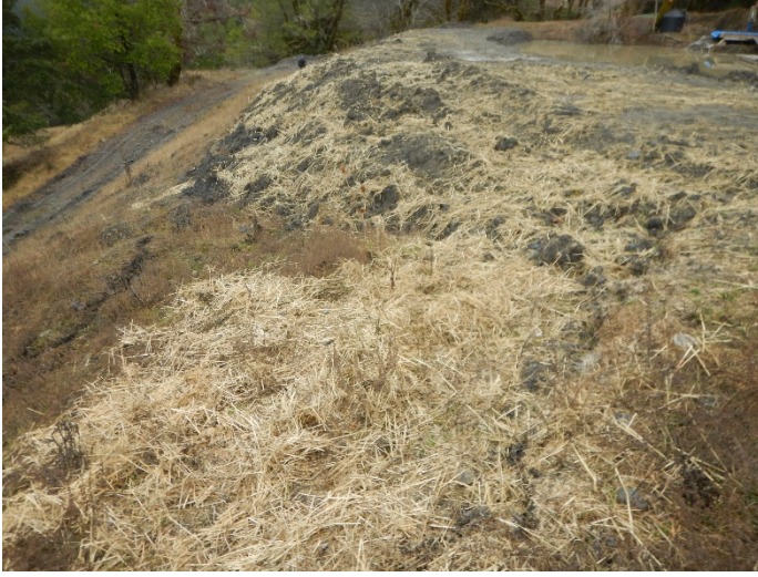
Photo 17: Cracking in the exterior face of the pond berm on the eastern side of the pond (DSCN4335)
