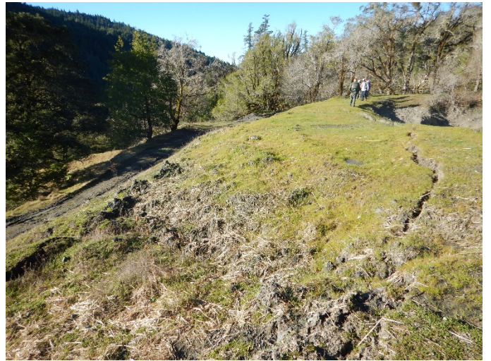
Photo 12: Pond berm showing cracks looking west (DSCN4436 photo taken February 21, 2019)
