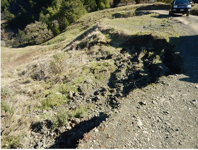
Photo 17: Road failure at road point RP1 looking south (DSCN9373 photo taken by Adona White, February 18, 2019)
