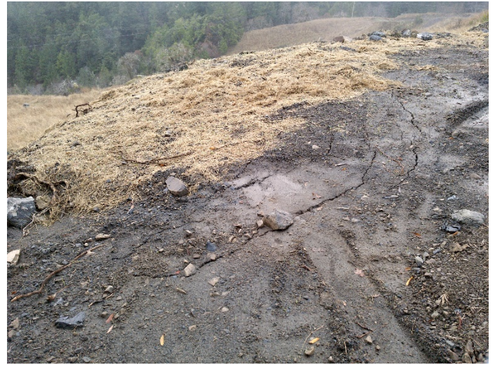
Photo 26: Cracking in fill at road point RP3 (DSCN0164 photo taken by Bryan Moore)
