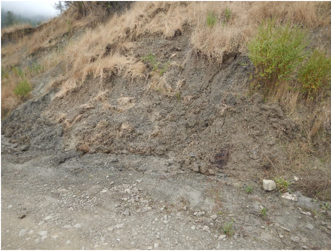
Photo 21: Slump on the main road (DSCN0141 photo taken by Sean Stout)
