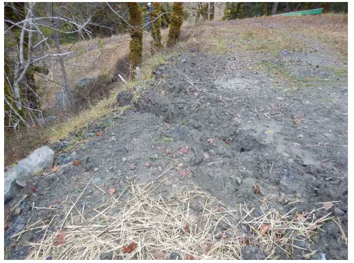
Photo 14: Cracking in the top of pond berm on the eastern side of the pond (DSCN4328)
