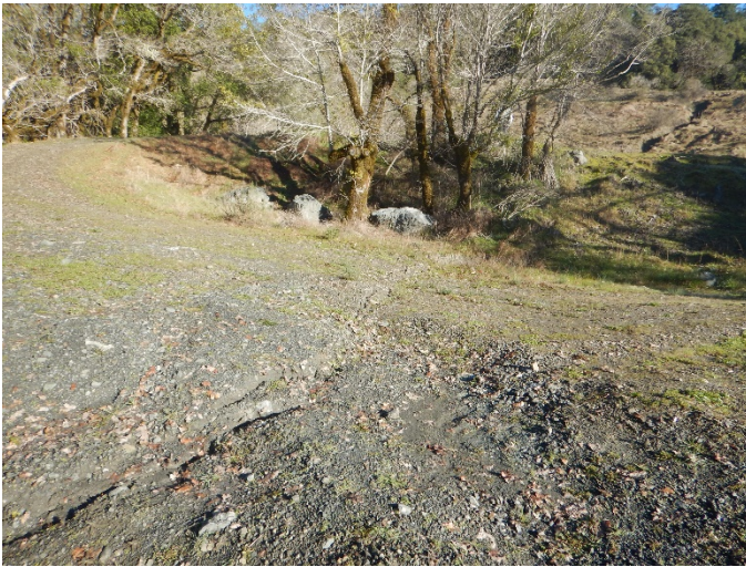
Photo 15: Lateral cracks on western side of pond (DSCN4426 photo taken February 21, 2019)
