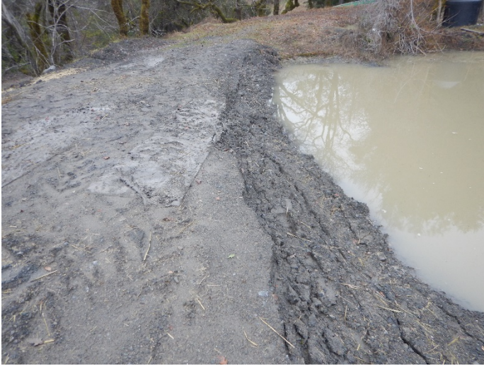
Photo 13: Cracking on the interior of pond berm (DSCN4307)
