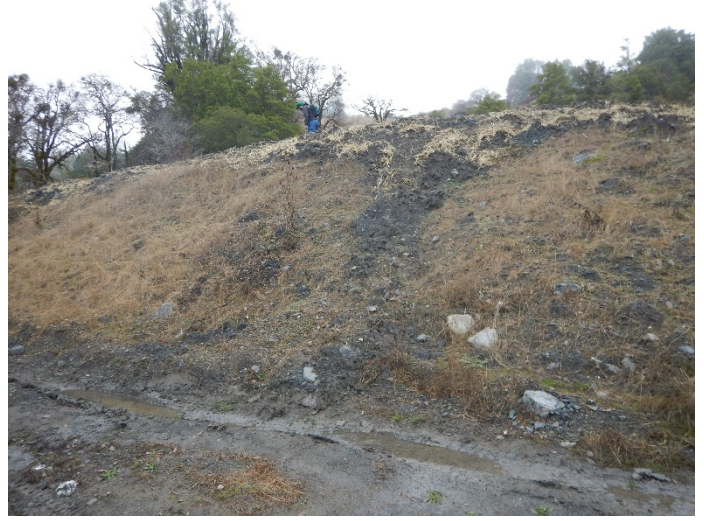
Photo 18: Exterior of pond berm with slumping (DSCN4330)
