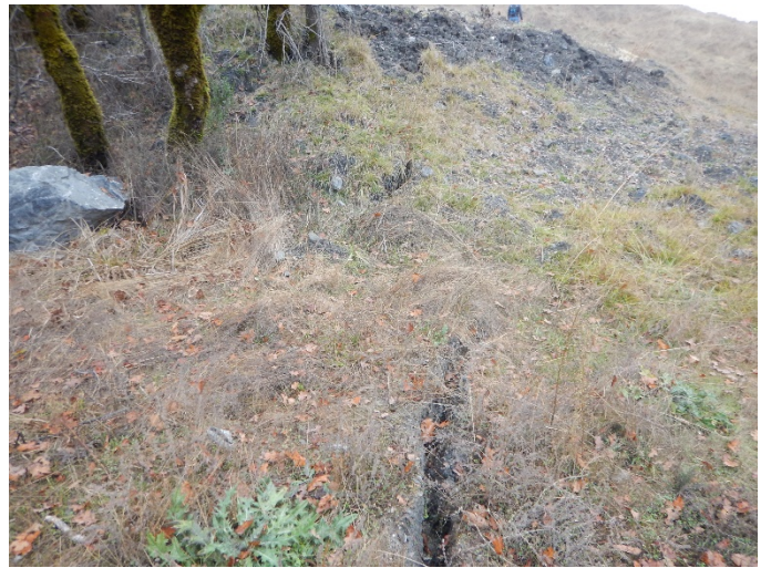
Photo 16: Closer view of cracking below the pond berm adjacent to the road (DSCN4327)
