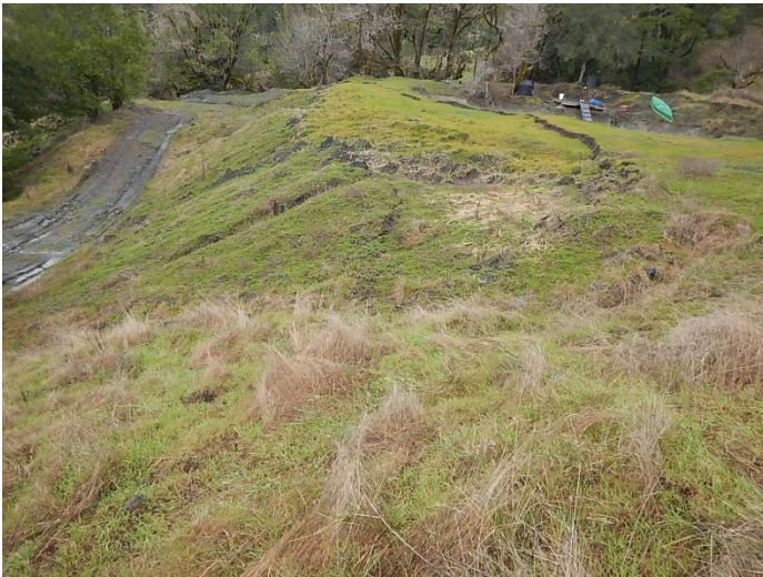
Photo 11: Cracking with pond berm (DSCN9469 photo taken by Adona White on March 1, 2019)
