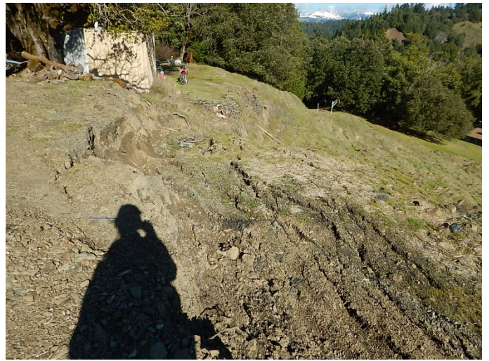
Photo 22: Road failure at road point RP3 looking north (DSCN9377 photo taken by Adona White, February 18, 2019)
