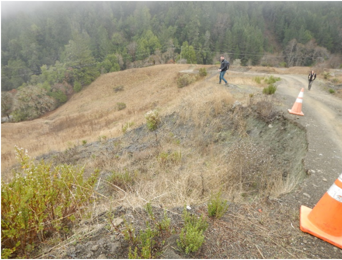
Photo 25: Edge of road collapsing at road point RP2 (DSC4340 photo taken by Bryan Moore)
