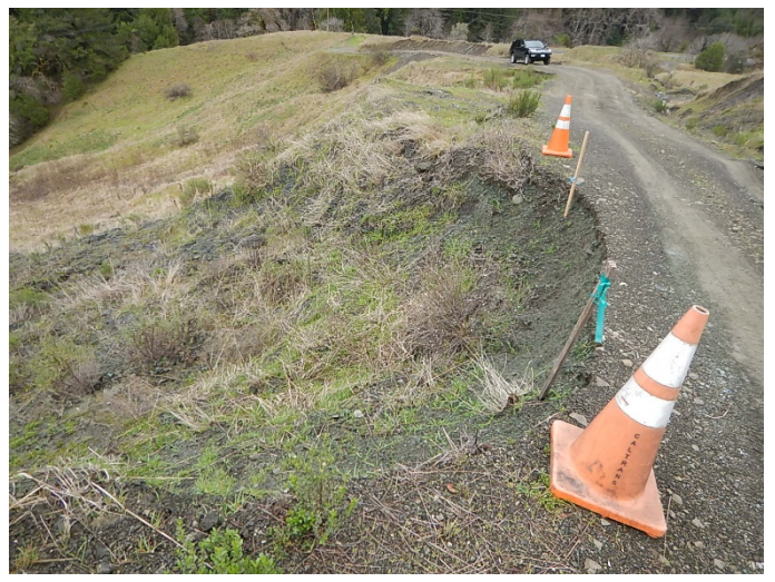
Photo 20: Road point RP2 uphill from RP1 (DSCN9538 photo taken by Adona White on March 1, 2019)
