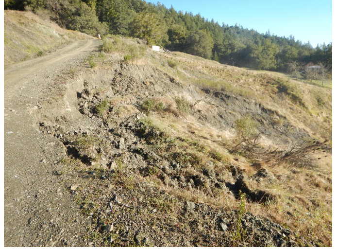
Photo 18: Road failure at road point RP1 looking north (DSCN4417 photo taken February 21, 2019)
