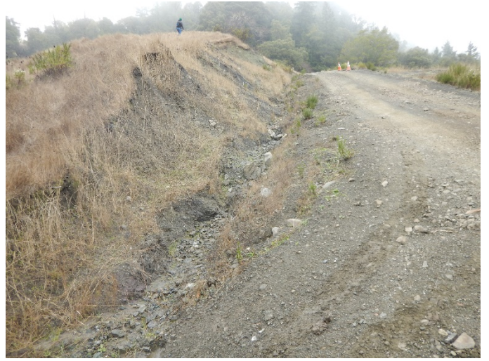
Photo 20: Main road with near vertical cuts and inside ditch adjacent to RP1 (DSCN4336)
