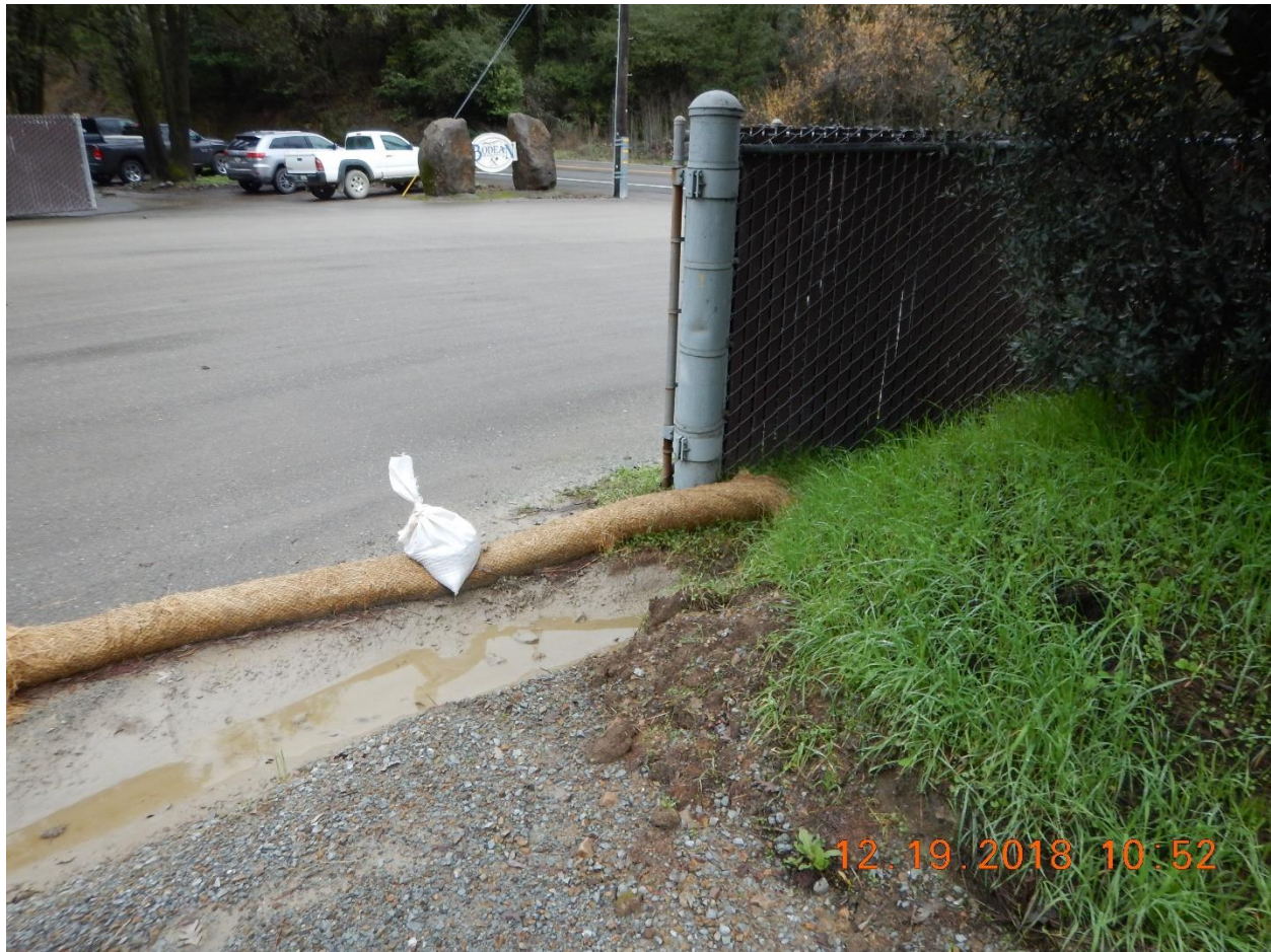
Photo 5 – View of quarry entrance and sediment buildup near gate. Photographed by Josh Luders.
