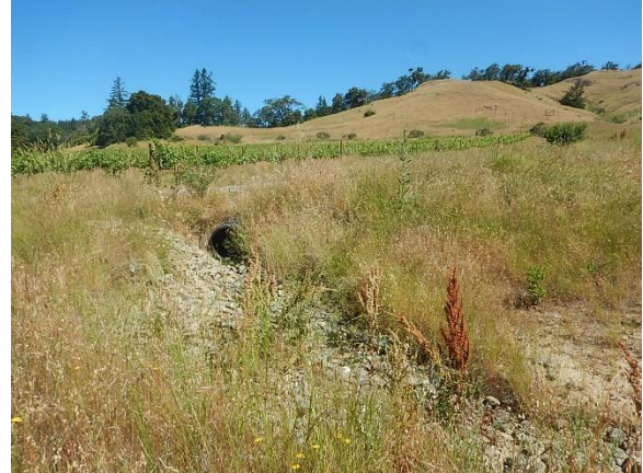
Figure 14. Where spillway goes under roadway and onto earthen surface before discharge to Class II watercourse.
