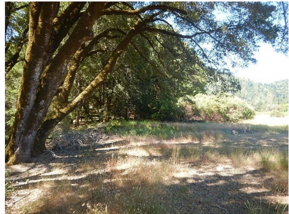
Figure 15. Downstream of spillway crossing, water flows over earthen surface before discharge to Class II watercourse. Water can mobilize fine sediment on its path.
