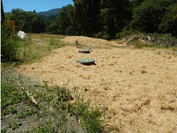
Figure 17. Recently installed mound septic system within 70' of top of bank of Class II watercourse.
