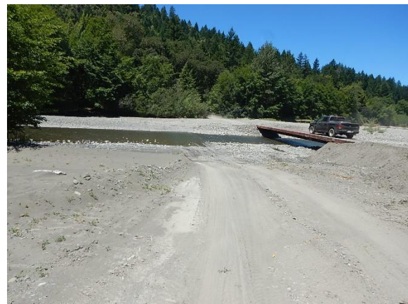
Figure 22. Low water bridge with unprotected embankments.
