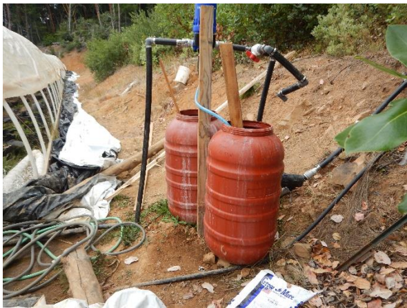
Photo 4: Fertilizer mixing tanks with no containment, leaking onto ground
