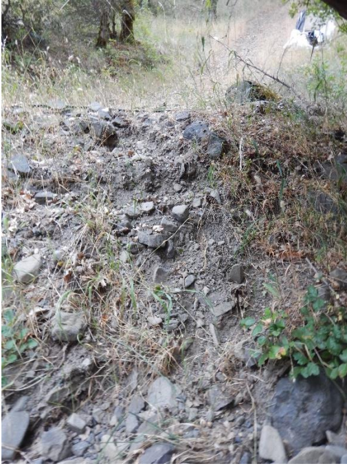
Photo 10: Sediment delivery from road above C1 to class II stream below
