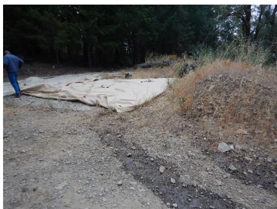
Photo 8: Bladder, B1, leaking its contents onto the road
