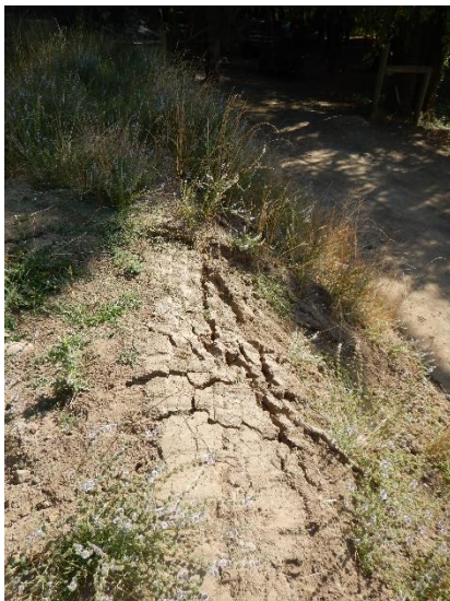
Photo 4: Tension cracking and sloughing on the fill face of P1
