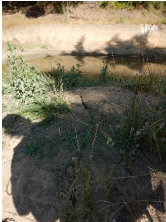
Photo 7: Deep tension cracks along berm of P1
