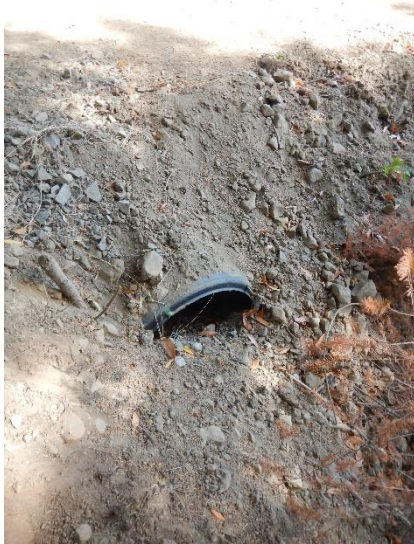
Photo 15: Buried outlet of C4
