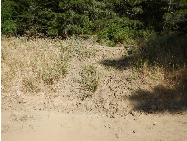
Photo 5: Sloughing of fill face material along P1 berm
