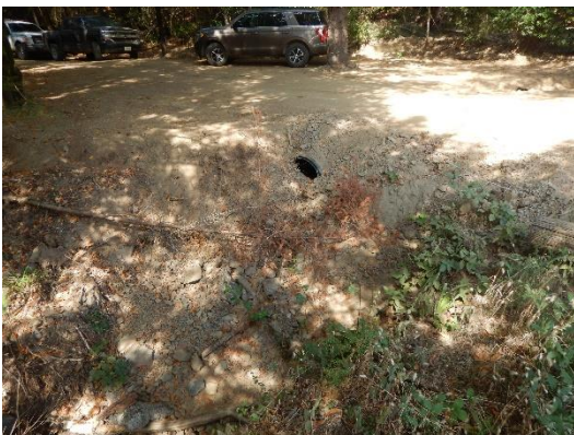
Photo 14: Buried outlet of C4 with recent pushed, loose, fill around the culvert
