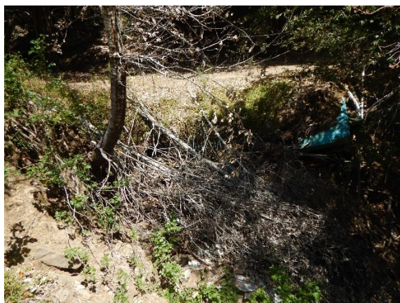
Picture 14: C2 outlet, blocked by brush and an old car is used to stabilize fill associated with crossing
