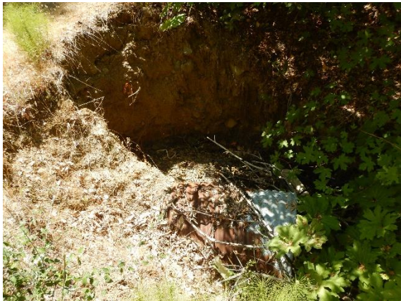
Picture 15: C3 inlet, scour around inlet evident
