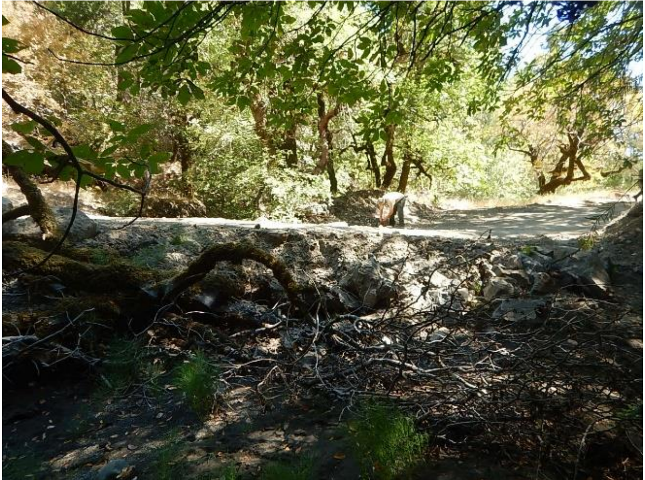
Figure 2. Crossing FORD, looking downstream at crossing fill. The crossing consists of rip rap in the channel, an undersized culvert near the right bank (facing downstream, on the far right of the photo), and loose fill placed over the watercourse as the road surface. The left road approach is hydrologically connected and in its current condition, will deliver sediment to the watercourse. This crossing has a high probability of plugging, failure, and sediment discharge in winter flows.
