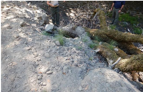
Figure 3. Rock and loose fill in the crossing, looking from the road surface. Cut tree is felled into watercourse upstream of the culvert.
