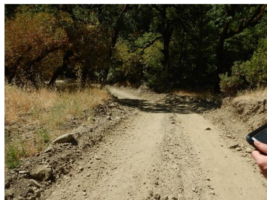
Figure 7. Left bank road approach to crossing FORD is hydrologically connected to the watercourse; the road is steep, and the condition creates the threat of sediment delivery to the Class II watercourse.
