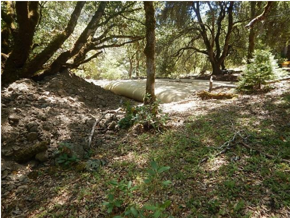
Figure 14. Pushed fill associated with the construction of the bladder pad.
