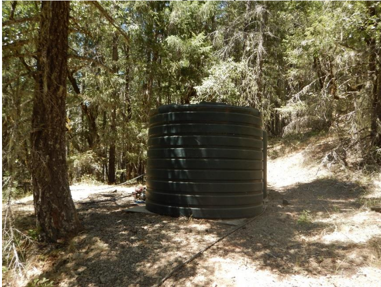
Photo 17: water storage tank near to inspection point C4
