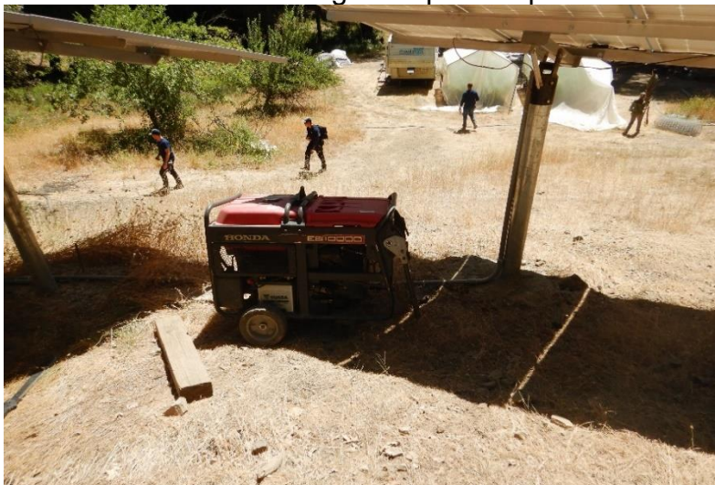
Photo 12: Uncovered or uncontained generator at inspection point GH4-5
