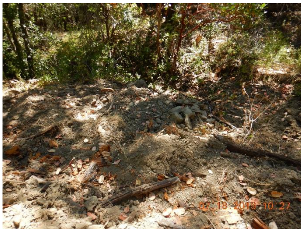
Photo 15 – Sediment in Class 3 (Crossing 2)
