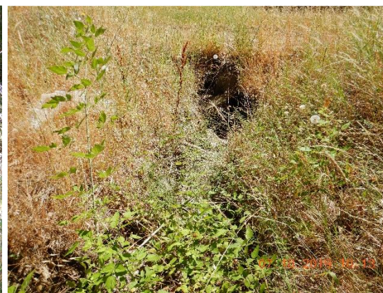
Photo 3 – Crossing 1 Upstream (undersized culvert)
