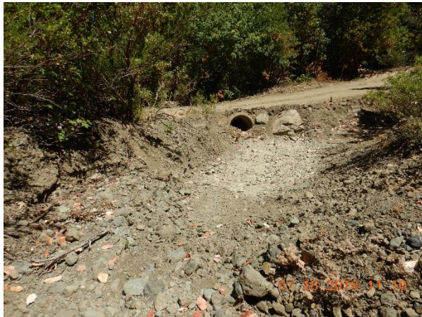
Photo 47 – Fine sediment deposits from pooled water showing impeded flow (upstream Crossing 6)
