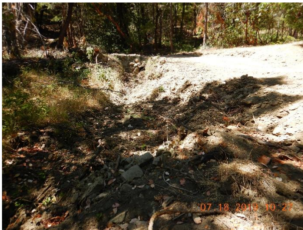
Photo 18-Sediment in Class 3 (Crossing 2)
