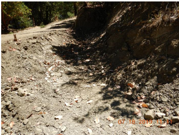
Photo 49 – roadside ditch leading to Crossing 4 showing sediment transport.
