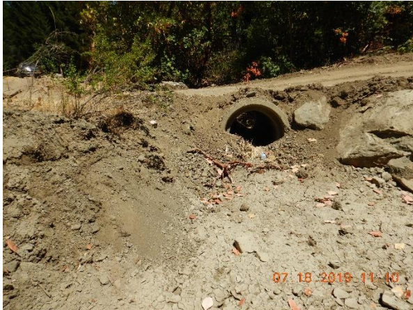
Photo 46 –partially obstructed and undersized culvert (Crossing 6)
