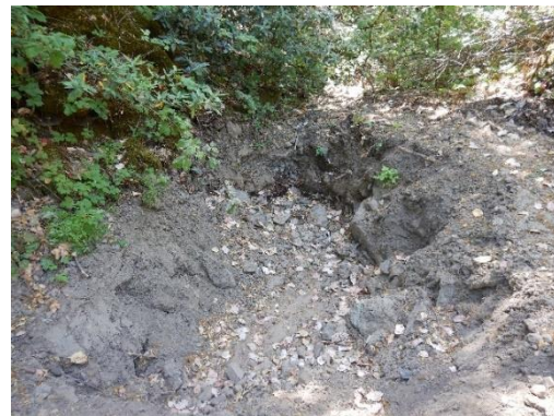
Photo – 8 Disturbed streambank and riparian area upstream of culvert.
