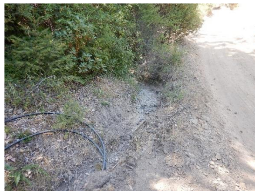
Photo – 10 Watercourse channel with road fill pushed into it. In addition, the watercourse channel shows signs of streambank disturbance from heavy machinery.
