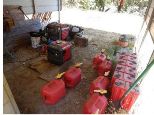
Photo – 6 Generator and gas tanks.
