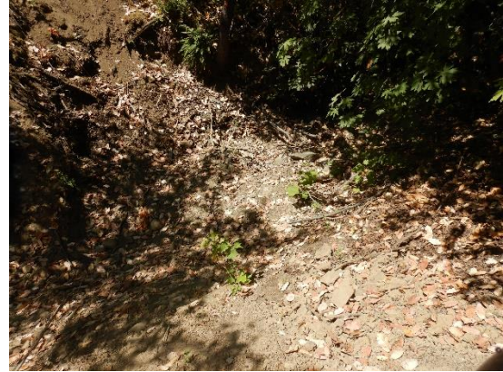
Photo – 15 Road fill extending into watercourse channel downstream of culvert outlet.
