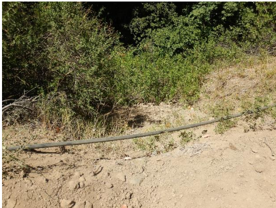
Photo – 16 Road fill pushed into watercourse.
