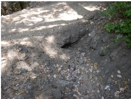
Photo – 9 Downstream view of culvert inlet filled with road fill and sediment. The streambank is disturbed along with riparian area. The banks show signs of heavy machinery work. The inlet of the culvert is cracked.
