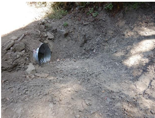
Photo – 12 Disturbed riparian area, 2-foot culvert, and bare, unstable soil in and around the stream channel.
