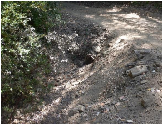
Photo – 7 Road built through a watercourse. A mostly buried culvert is visible in the loose fill and unstabilized fill slope.
