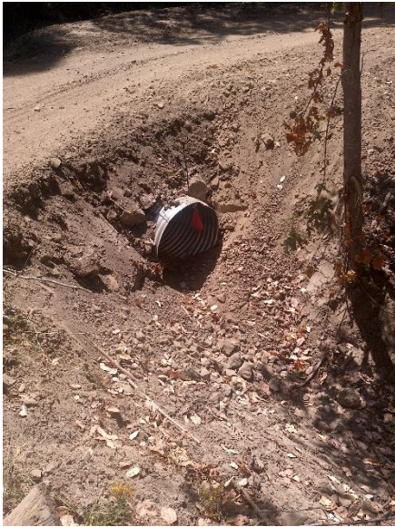
Photo – 14 Culvert outlet with discharged sediment and loose road fill into watercourse.
