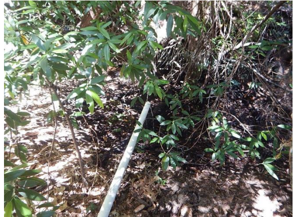
Figure 49. Discharge pipe for overflow water from water diversion to tank.
