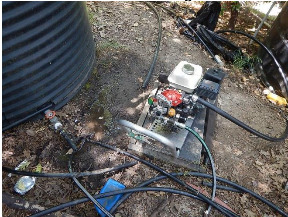
Figure 47. Gas powered water pump used to divert water from watercourse to tanks.
