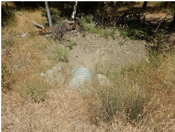
Figure 3. Culvert outlet with sediment deposition restricting capacity.
