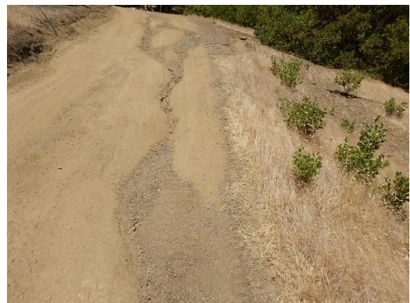
Figure 41. Concentrated water has formed rills in the road surface to CA4.
