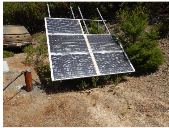
Photo – 2 Well head with solar pump.
