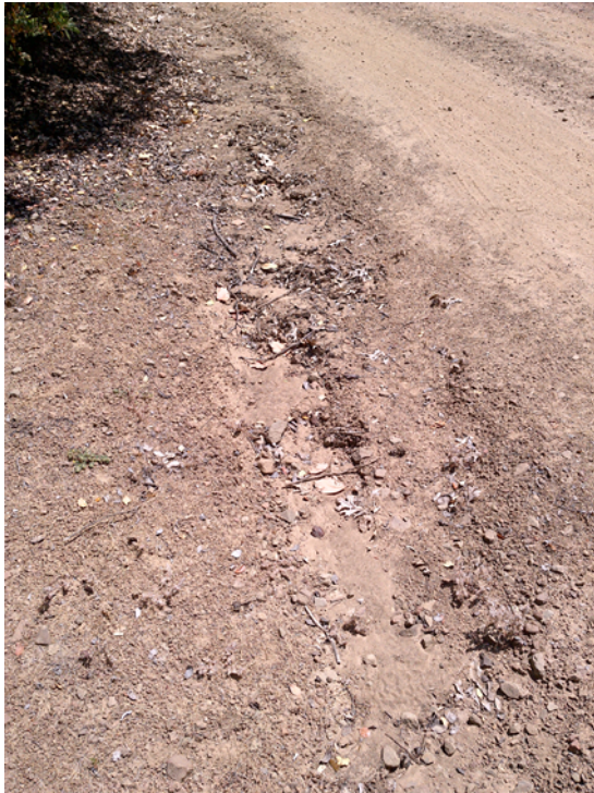
Photo – 3 Outboard road erosion.
