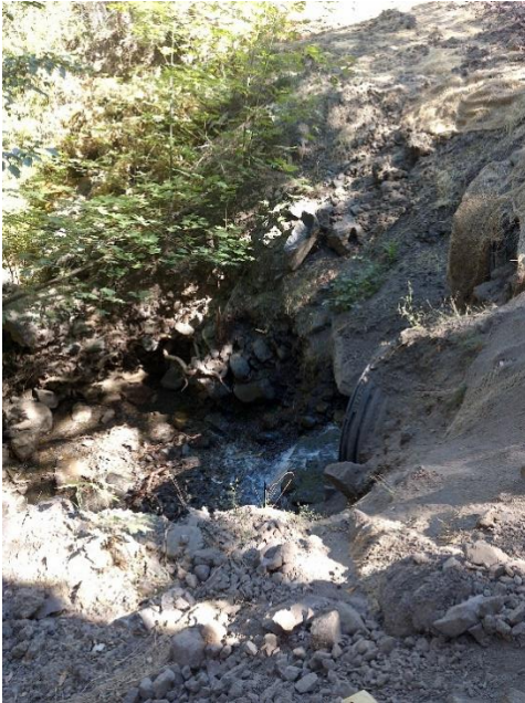
Photo 11 – Double culvert outlet with unstable fill slope.
