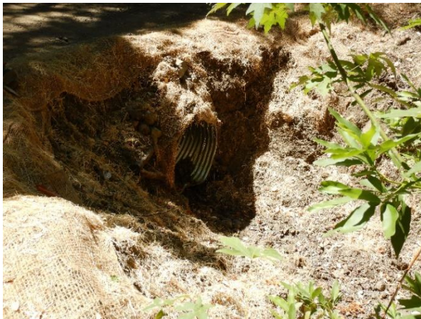
Photo 23 – Culvert outlet with unstable fill slope and damage to the bottom lip of the culvert.
