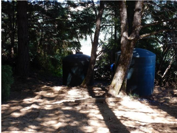
Photo 21 – Water storage tanks.
