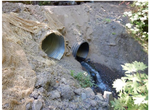
Photo 14 – Culvert outlets and unstable fill slope.
