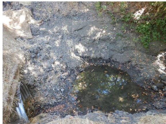
Photo 22 – Culvert inlet and streambank and channel disturbance.
