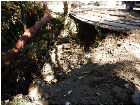
Photo 17 – Landslide area discharging into watercourse.
