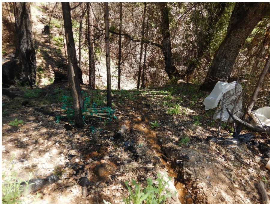
photo 5 – Continuation of trench shown in photo 4, in the vicinity of WQ 2. Valley in background of image contains a watercourse.
