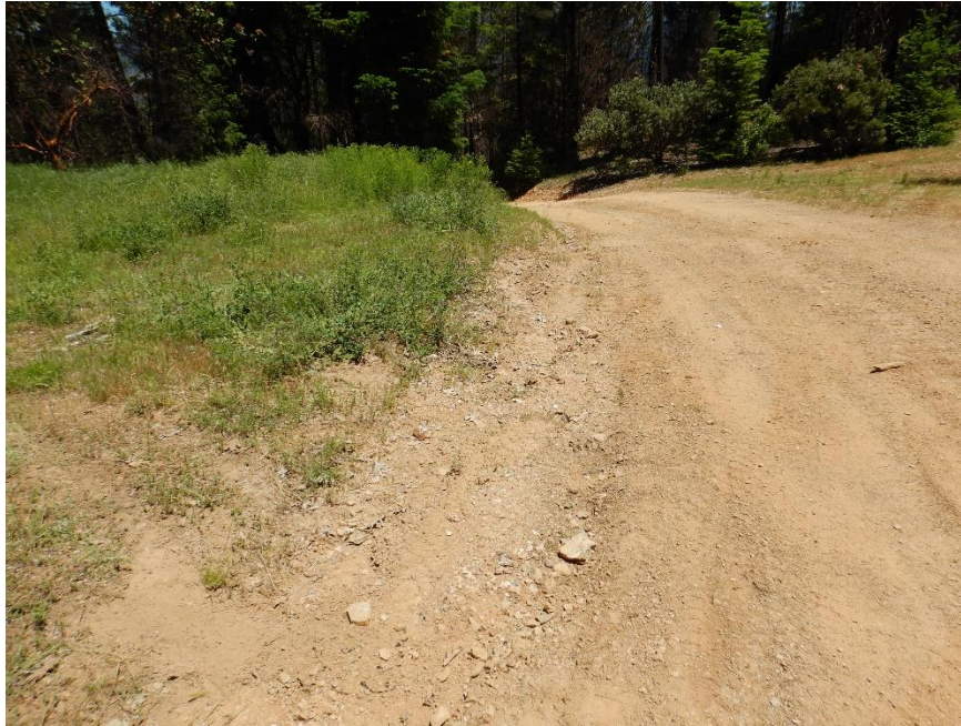
photo 11 – Rilling on road-surface; evidence the road is susceptible to erosion by stormwater.
