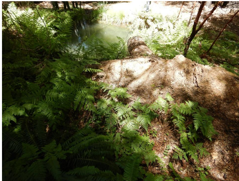
photo 12 – Reservoir excavated in watercourse at road crossing at WQ 5. The reservoir is approximately 8 feet deep. Impounding fill is approximately 8 feet high, 30 feet wide and 40 feet long.
