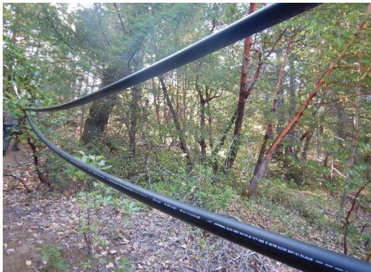
Photo 11 – Large irrigation lines leading to water storage tanks.
