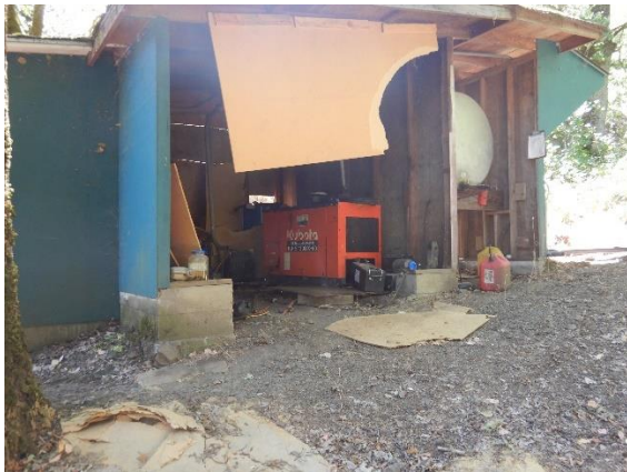
Photo 21 – Large diesel generator and large fuel storage tank.
