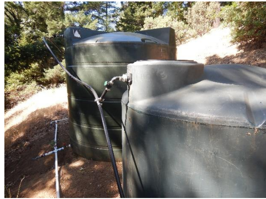
Photo – 14 Primary water tank storage area.
