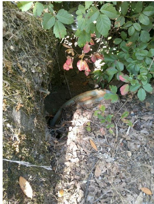
Photo – 16 An undersized culvert with sediment discharge.
