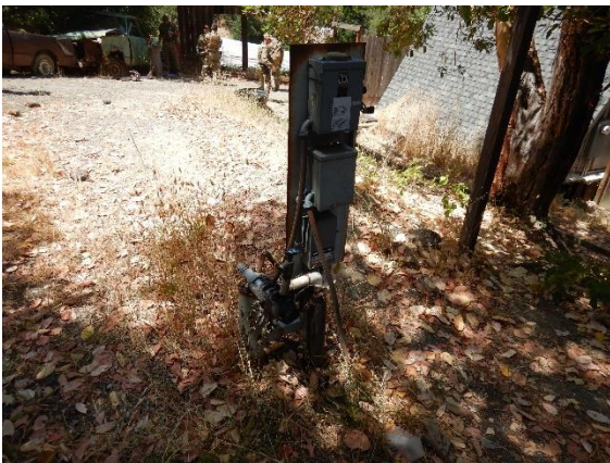
Photo 3 - Ground water well and pump.
