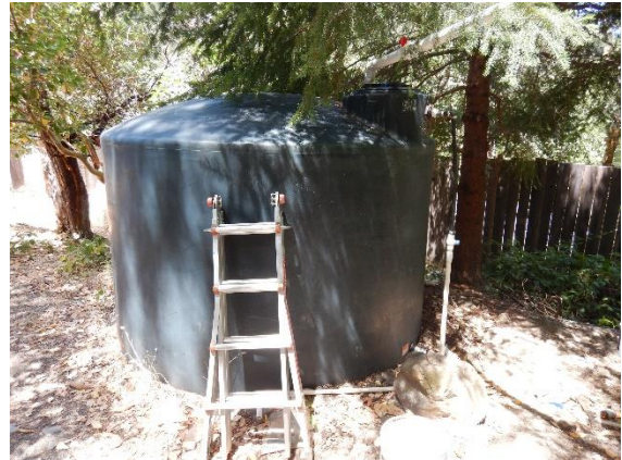
Photo 2 – Water storage tank.
