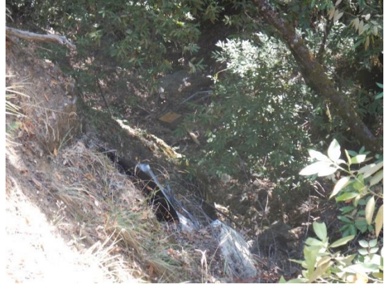
Photo – 18 View of stream channel with trash and debris.
