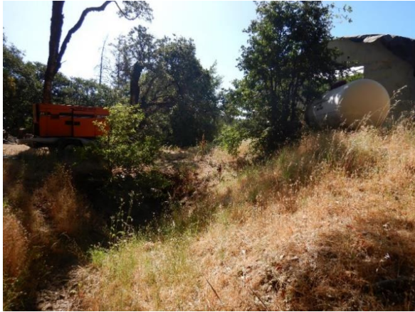
Photo 5 – Diesel generator above the culvert inlet at inspection point Cannabis cultivation area #2 and fuel tank are visible in this image and are less than 50 feet from the Class III watercourse at this location. (Inspection points 3, 4, and 5)
