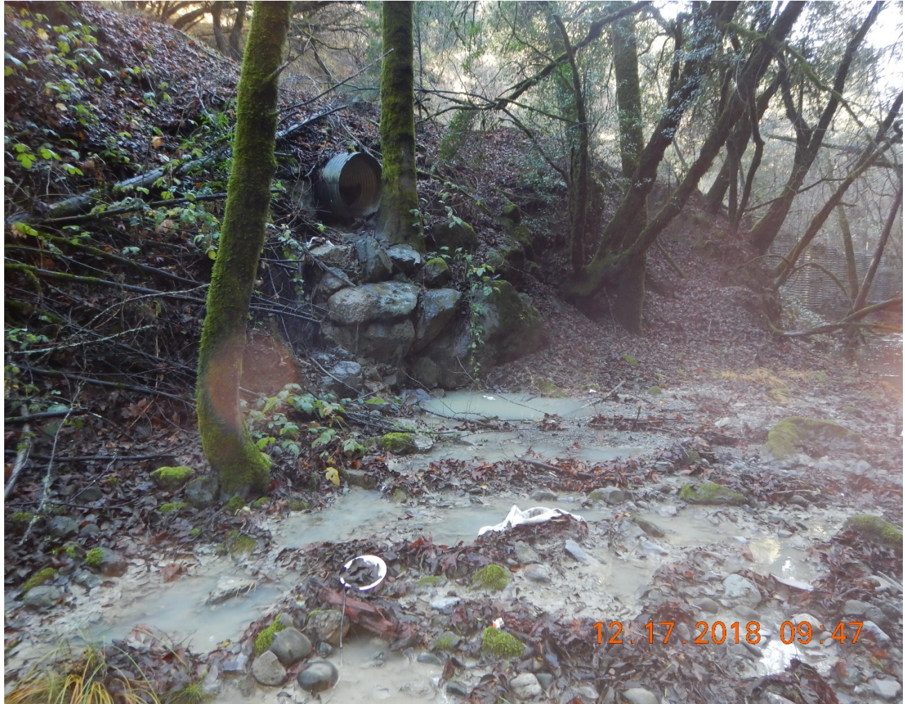
Photo 4: Photograph of sediment below eastern outfall pipe from Mark West Quarry to Porter Creek taken by Paul Nelson.
