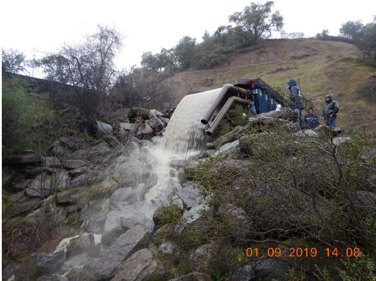
Photo 4: View of discharge from settling tanks at the top of east culvert drainage. Runoff from the site exceeded the capacity of the collection and settling system. Photographed by Josh Luders.
