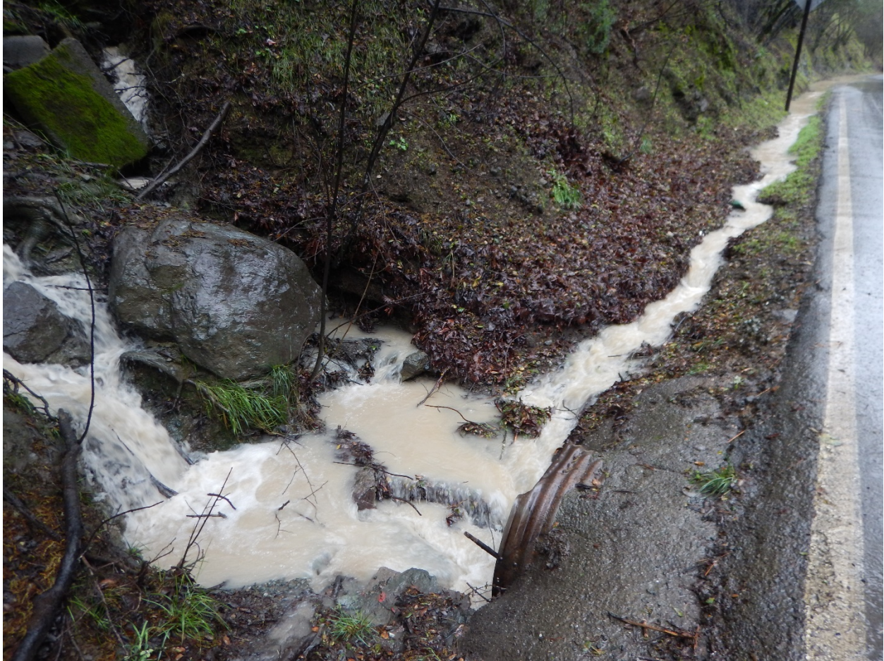
Photo 5: View of culvert and confluence of water from east drainage. Turbid water evident in drainage and confirmed by turbidity results. Photographed by Paul Nelson.
