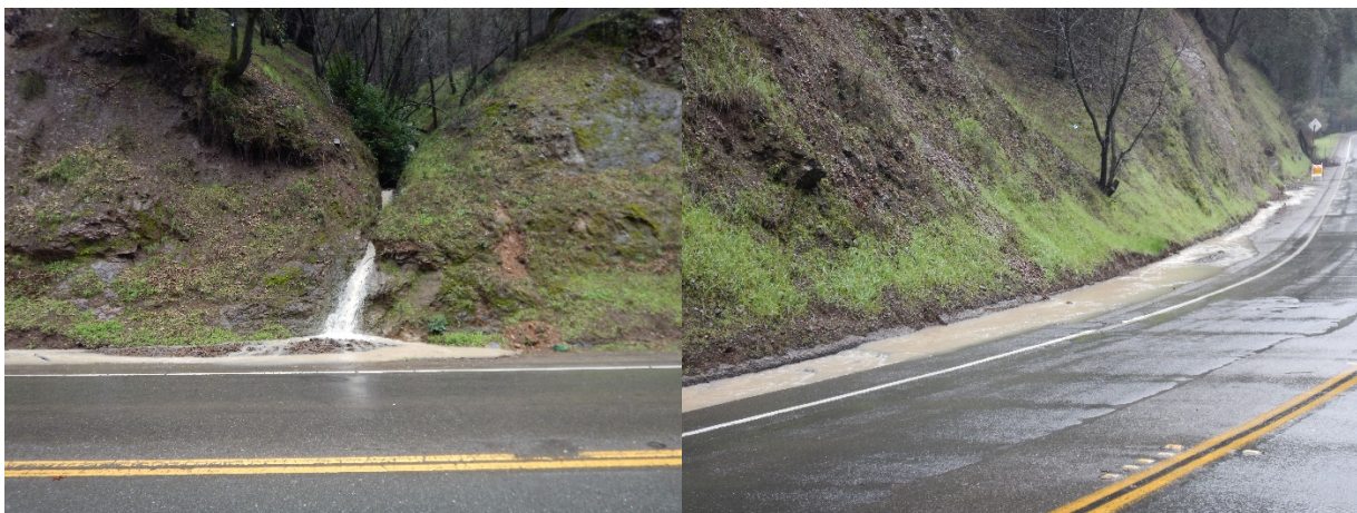
Photos 3 and 4: View of eastern drainage. Water bypassing drop inlet and flowing along roadway. Photographed by Paul Nelson.
