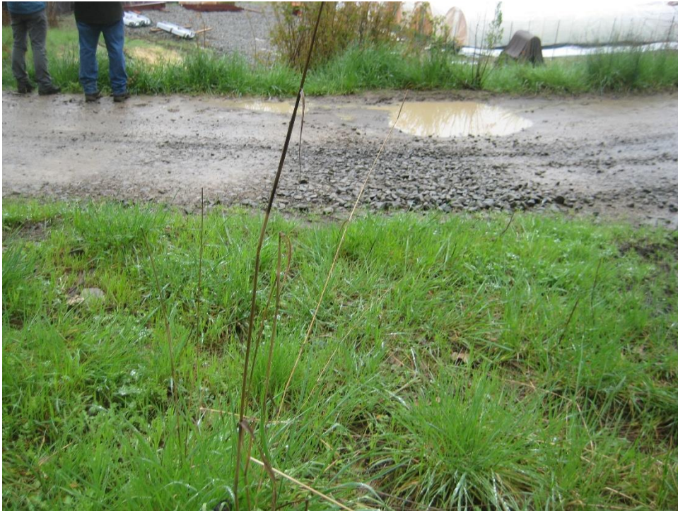
Photo 16. Site 2 road at plugged culvert crossing.
