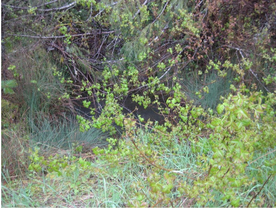
Photo 15. Site 2 upstream of plugged culvert road crossing. Note pooled water.
