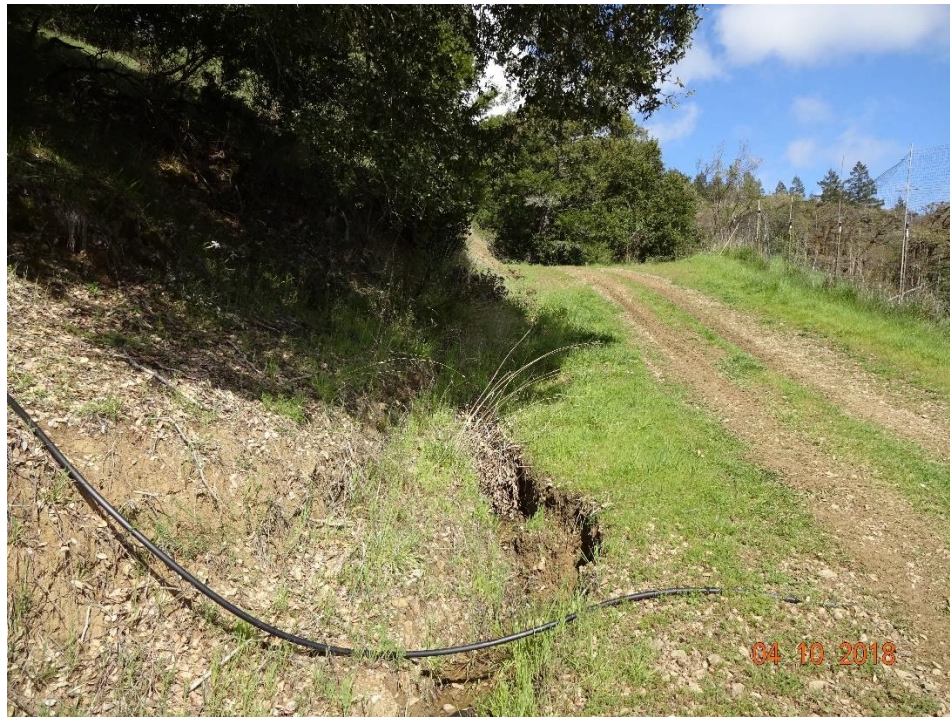
Photo 39. Road leading to Site 7, water running down inboard trench.
