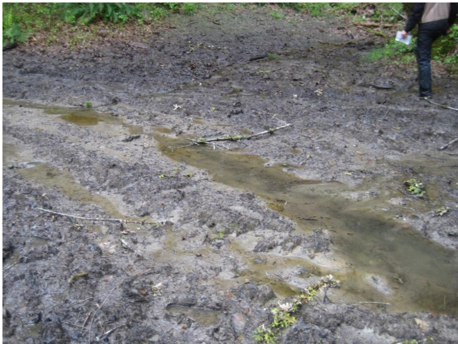
Photo 28. Site 3, Water flowing over road surface.
