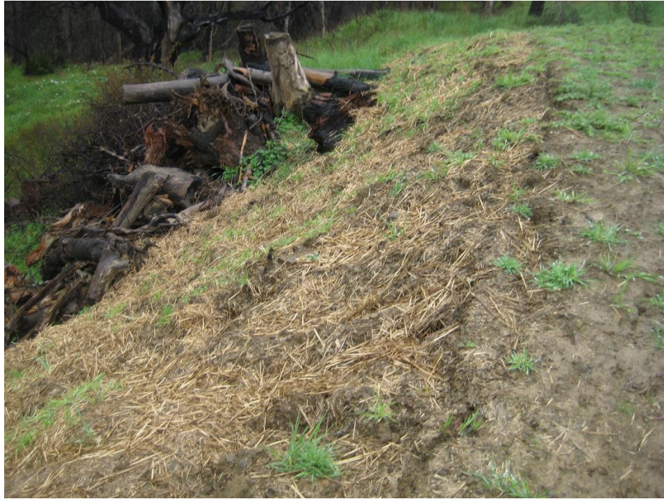
Photo 19. Site 2, tension cracks on east face of recently expanded fill pad.
