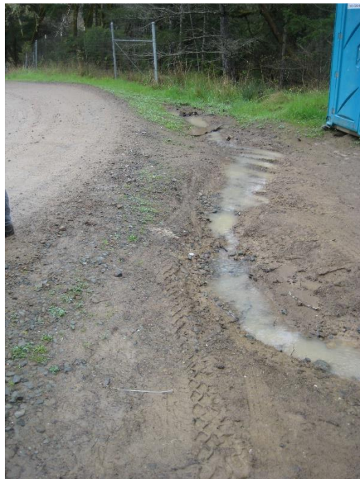
Photo 24. Road south of Site 2, water from ditch, flows over road-surface.
