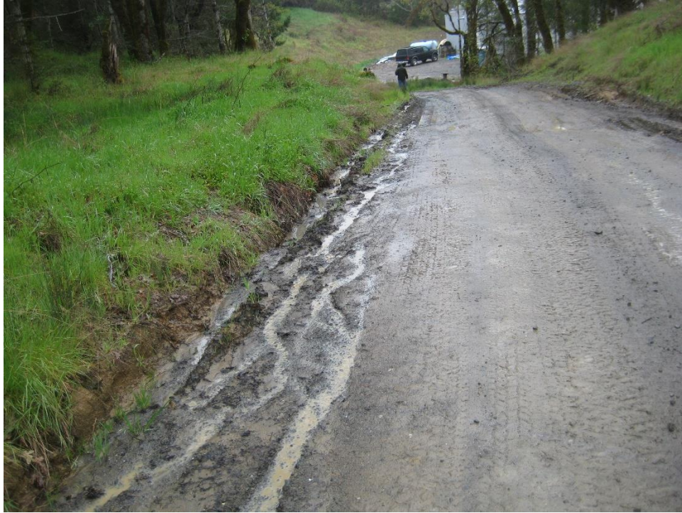
Photo 7. Water flowing over road-surface on road leading to Site 1 Glass House.
