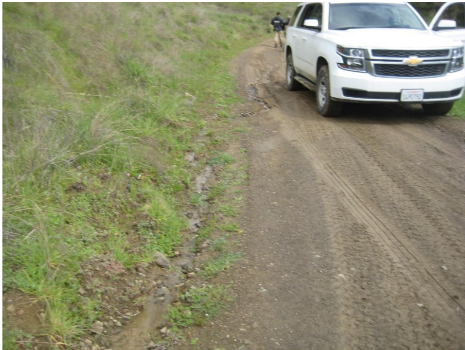
Photo 36. Water flowing from trench, over road-surface between Sites 5 and 6.
