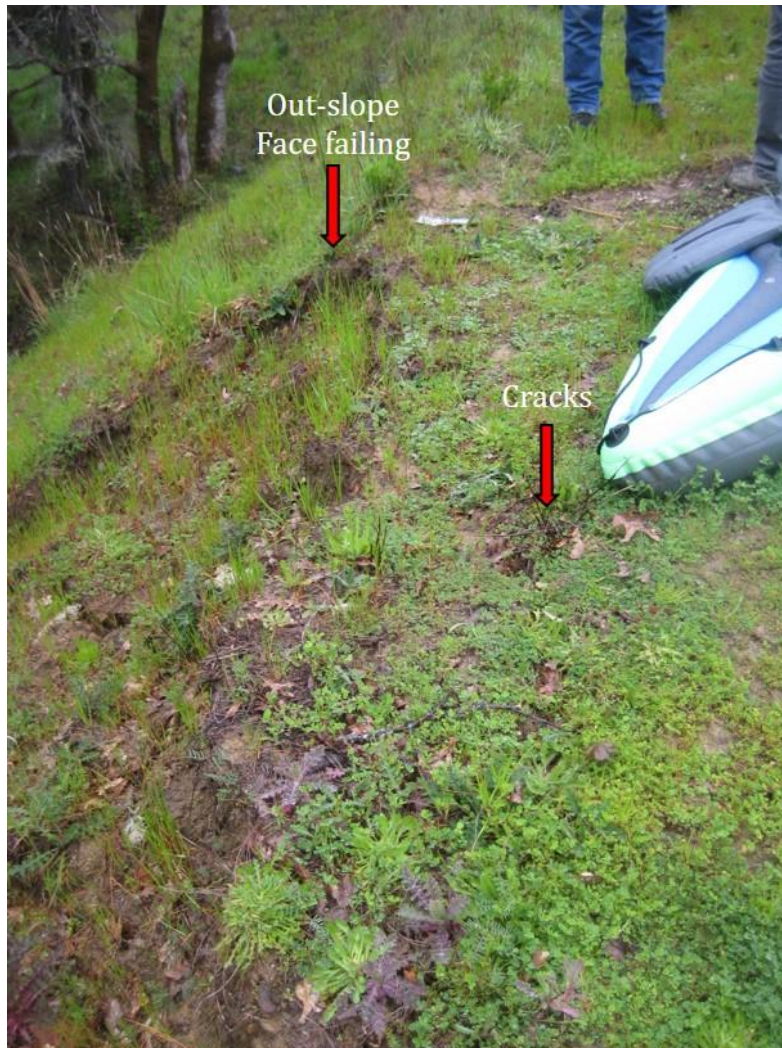
Photo 2. Cracks and slumping on out-slope face of the northwest pond buttress, southwest of the spillway.
