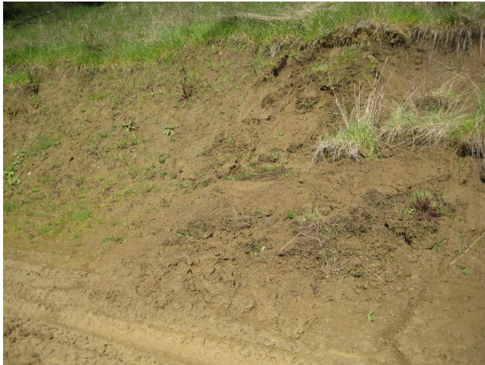
Photo 38. Road leading to Site 7, water seeping out of cutbank onto road.
