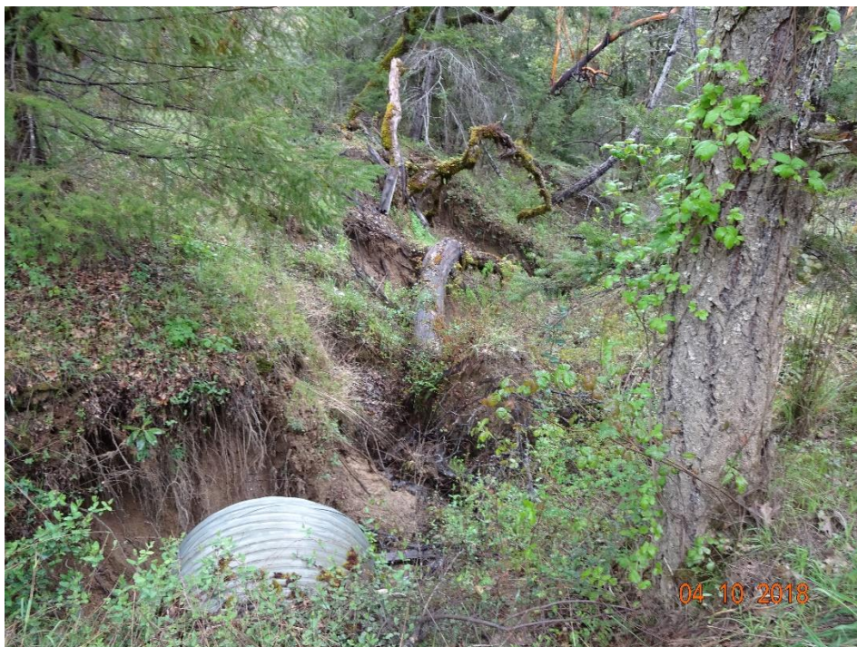
Photo 30. East of site 4, incised gully at culvert outlet.
