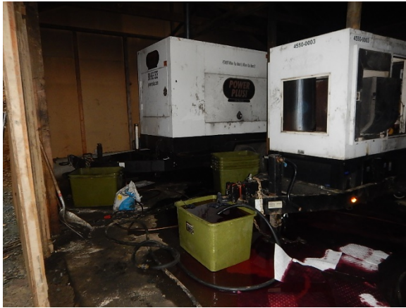
Figure 62. The landowner representative opened the generator shed, where there were three large generators. The fuel line from the storage tank to the shed had overtopped a tote with a crack in it and spilled over the floor of the shed building. The concrete floor appeared to have contained the spill while we were there.
