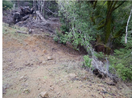
Figure 20. Decommissioned crossing at Site 45, looking downstream. The WRPP indicates that the earthen ford Class III crossing was pulled per an approved LSAA agreement. The Regional Water Board has no record of submission of an instream workplan or 401 application for the instream work. The crossing appears to have stabilized but lacks evidence of replanting or regrowth.
