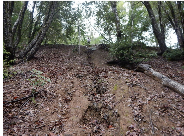
Figure 29. The water from site 44 has formed a gully that extends downslope and is eventually dissipated by some downed trees.
