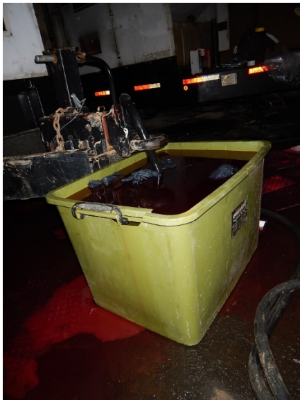
Figure 63. Tote overflowing and spilling onto floor.
