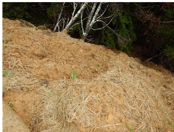
Figure 125. CAA: Recent fill slope erosion where wattle was not adequate.
