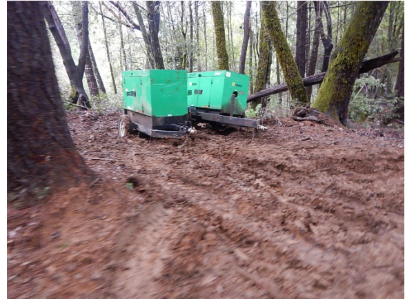
Figure 16. South of CAJ, I observed another two generators that were recently placed and are uncovered. Native soil was disturbed in the placement and had not been stabilized.
