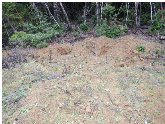
Figure 143. Gully erosion at CAC.
