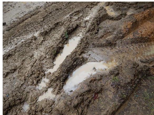
Figure 13. Tire ruts were evident on the native road surface. The road surface is inadequate for winter use. I observed a slight sheen on the surface of water that was pooled in the ruts.
