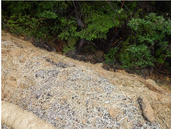
Figure 126. CAA: Potting soil over edge of fill slope.
