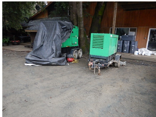
Figure 48. Two generators located at the residence.
