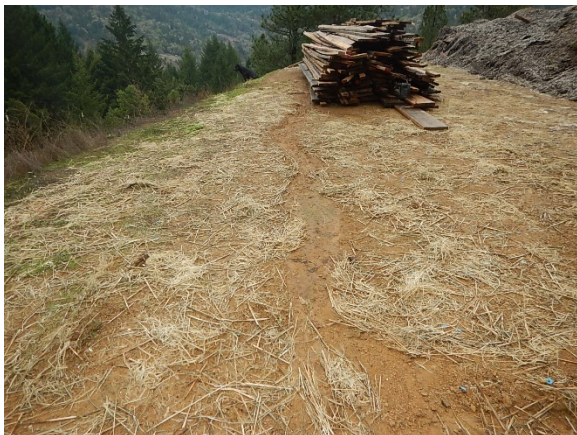
Figure 87. The flat at CAH has not been stabilized and the surface is eroding.
