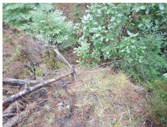
Figure 103. Edge of landing at CAD is eroding in some locations and should be stabilized.
