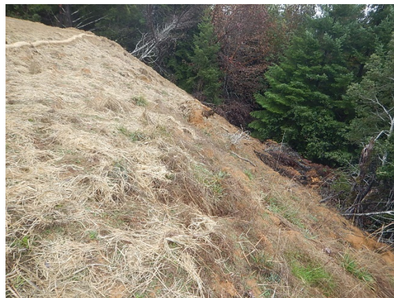
Figure 123. Slumping fill slope at CAA.
