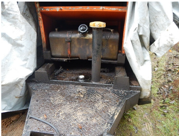
Figure 10. One of the generators had petroleum product drips on the trailer.
