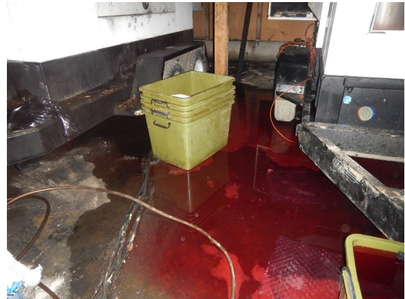
Figure 64. Diesel on floor.
