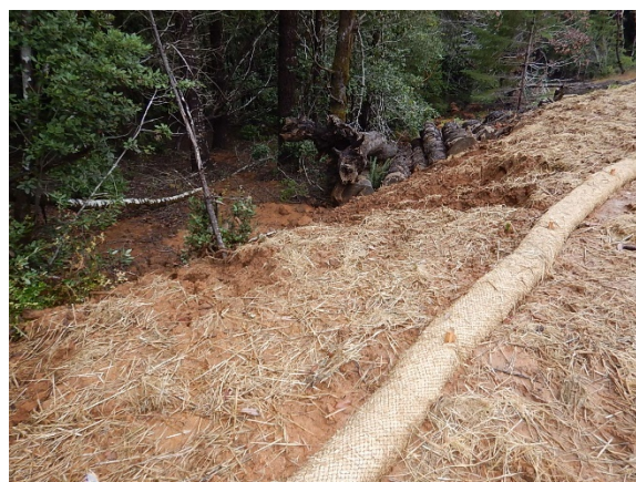
Figure 137. Fill slope is eroding at CAC. Concentrated road runoff, Inadequate
