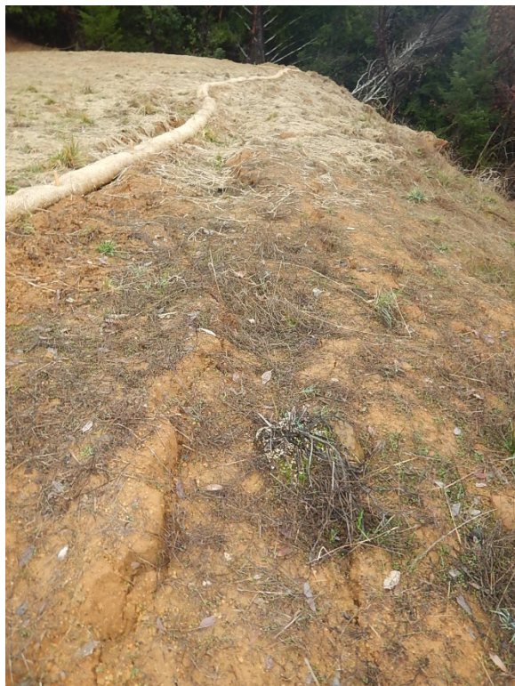
Figure 122. Fill slope cracks at CAA.
