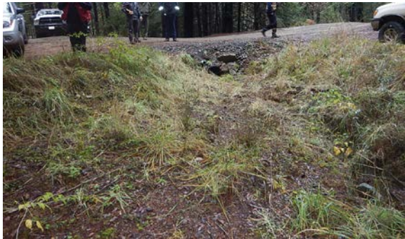
Figure 78. Corrugated plastic pipe at site 19.
