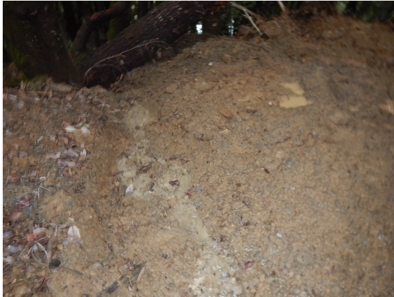
Figure 77. Drain out with erosion and transport on upper road to CAH.
