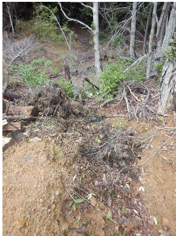
Figure 144. CAC fill gully.
