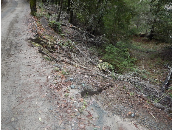
Figure 91. Site 18 hydrologically connecting a long run of road surface to surface waters.
