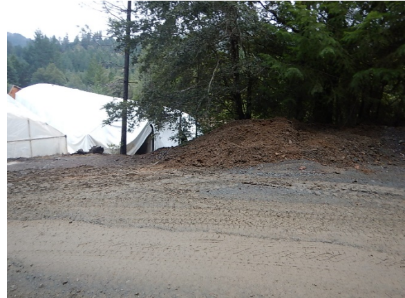
Figure 51. The road drainage from the north east is eroding spoils of earthen material above the cultivation area CAI, which is constructed on a cut and fill flat below the northern road.
