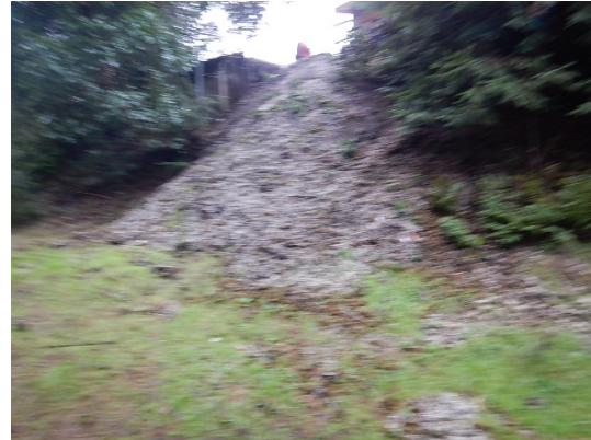
Figure 33. Potting soil pile placed below the residence is not stabilized and is eroding, transporting, and at least threatening to deliver to watercourses downslope along with the blackwater.
