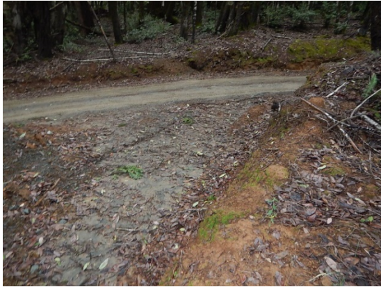
Figure 108. Site 15: Road surface drainage bypasses the drain-out and discharges to surface waters.
