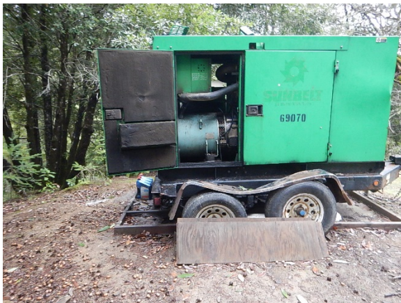
Figure 36. Generator located near the residence is not covered,
