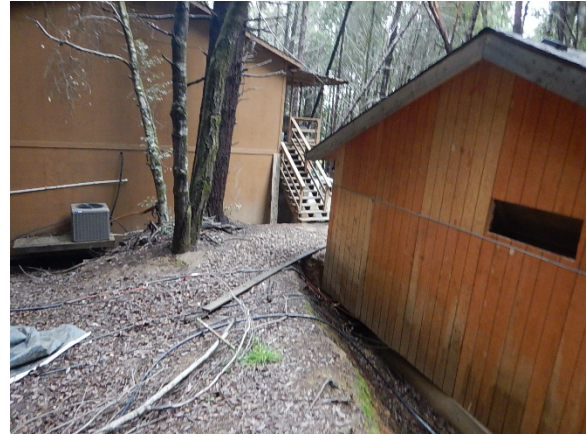
Figure 60. The generator shed is not attached to the foundation along the back side of the building. Below the generator shed are two 2-story indoor cultivation facilities. I did not view the interior of the indoor cultivation buildings.
