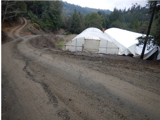
Figure 49. The gully at the residence (site 42) is fed by water entering the area via four different road segments and the cultivation area CAI. This photo shows the north eastern road, with concentrated drainage going down the road and into the cultivation area CAI. The south eastern road (upper left of photo) brings runoff to site 42 also.
