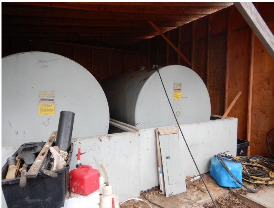
Photo 12—Covered fuel storage with secondary containment.
