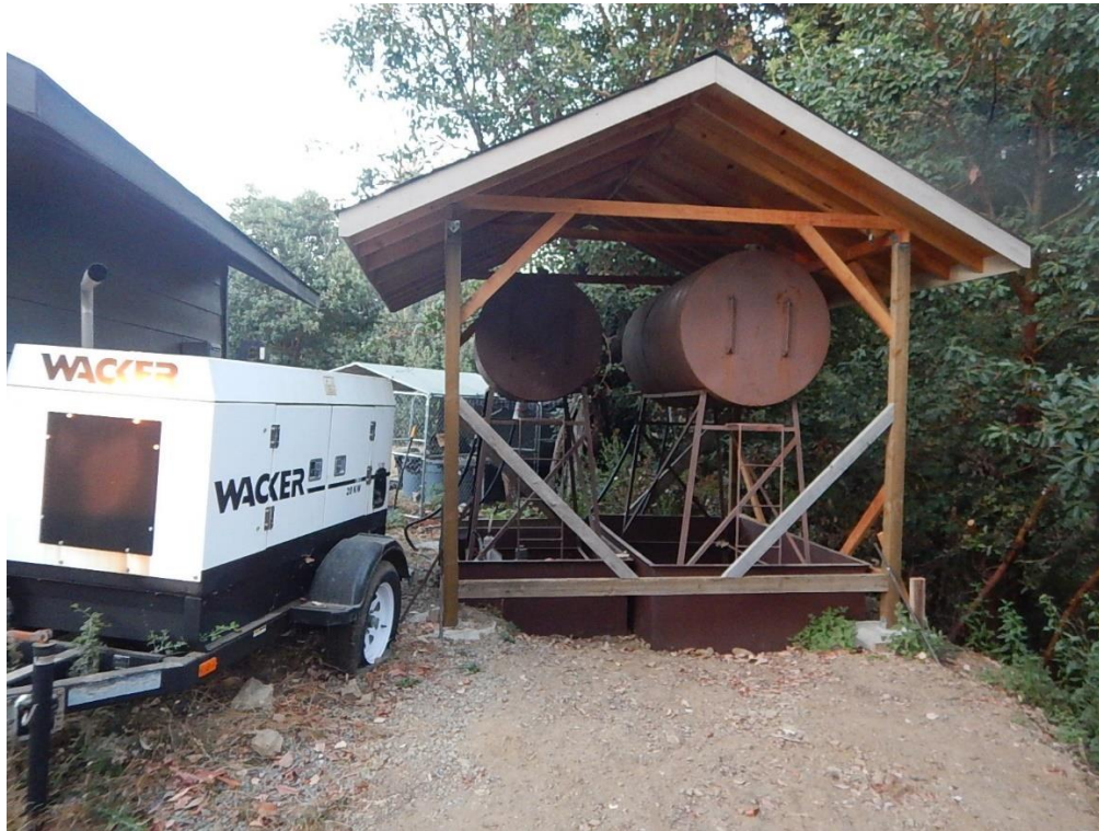
Photo 5, Petroleum and generator at inspection point Fuel
