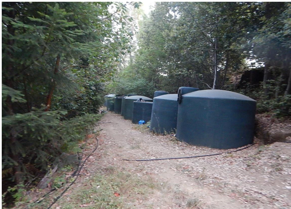
Photo 6, Water storages at inspection point WST2
