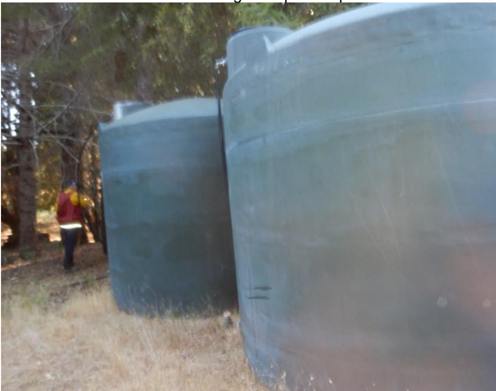
Photo 2 water storage tanks at inspection point WST1
