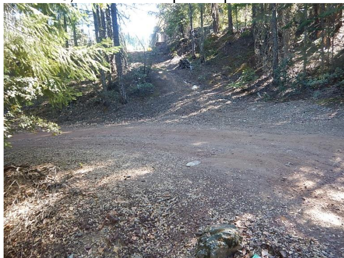
Photo 19, Threatened sediment delivery from the road near SC2
