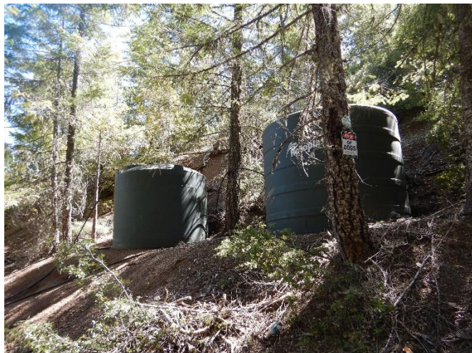
Photo 3 water storage tanks at inspection point WSTG1
