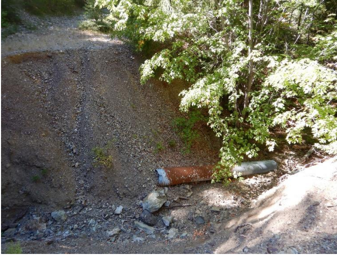
Photo 15 blown out stream crossing at inspection point SC3
