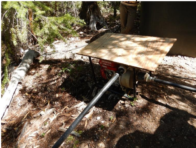
Photo 8 uncontained pump at inspection point Tank pump
