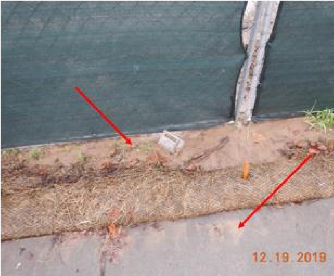
Photo 3: The red arrows show sediment deposition from the uncovered disturbed soils on the other side of the fence. Sediment buildup was seen at numerous locations along the sidewalk. Photo taken and edited by Joshua Luders.
