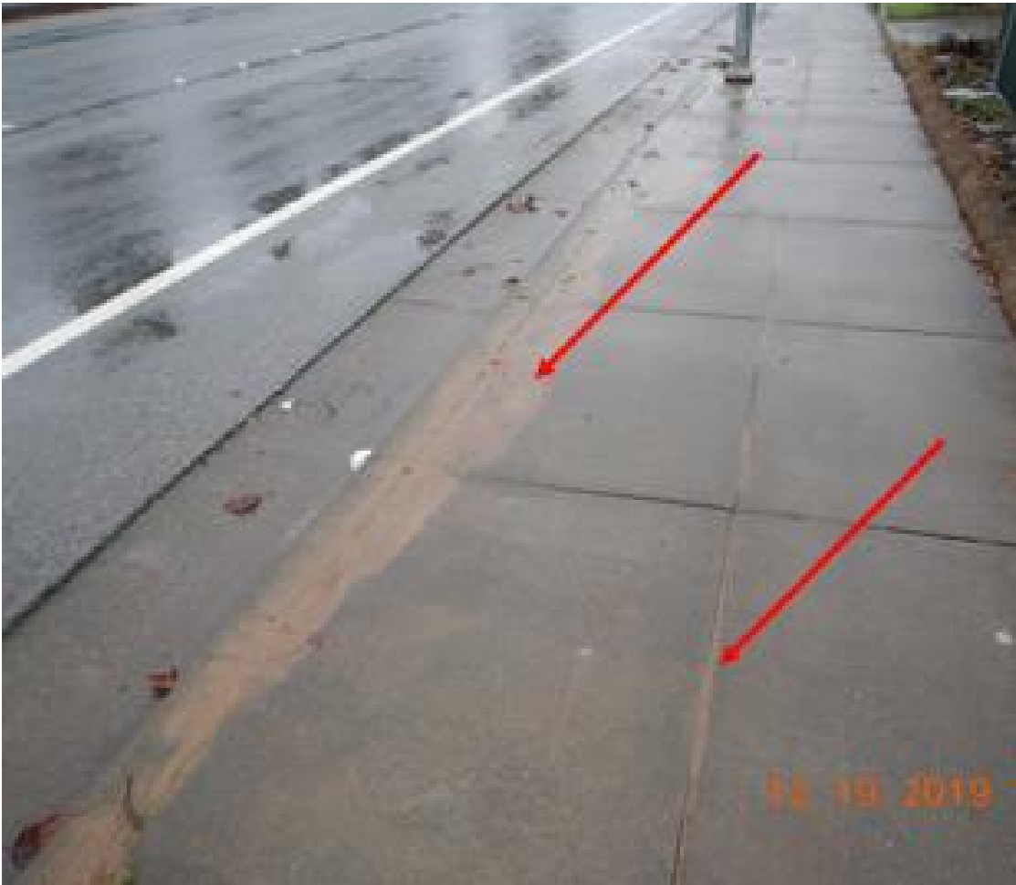
Photo 4: Sediment deposition was found along the sidewalk near the City's storm drain system. Sediment deposition(s) seen on the side walk could be correlated to the deposition seen along the fence line and near the wattles, like that depicted in Photo 3. Photo taken and edited by Joshua Luders.
