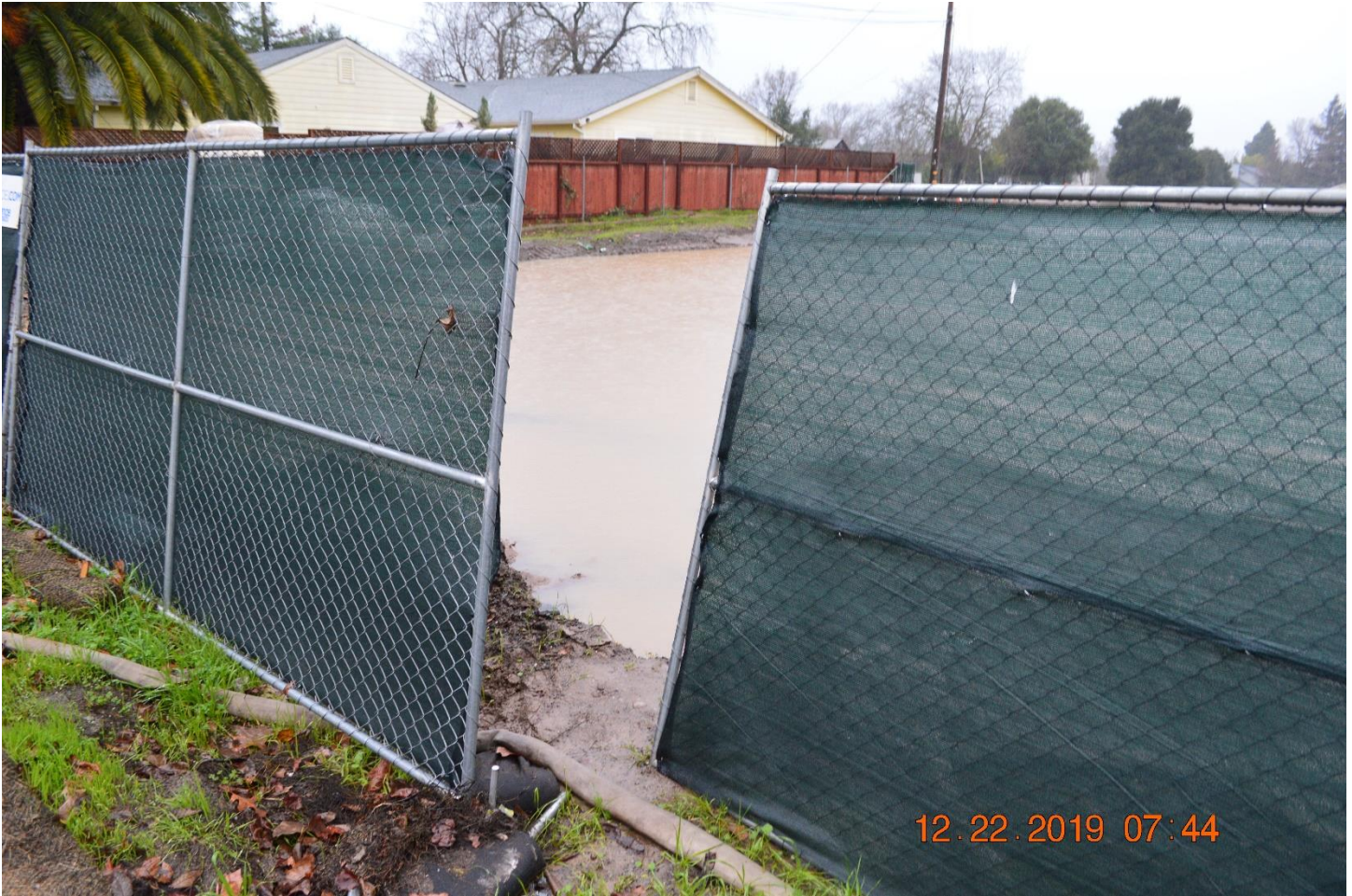
Photo 3: Ponding of turbid waters observed on the construction site near the sidewalk on Guerneville Road. Photo taken by Joshua Luders
