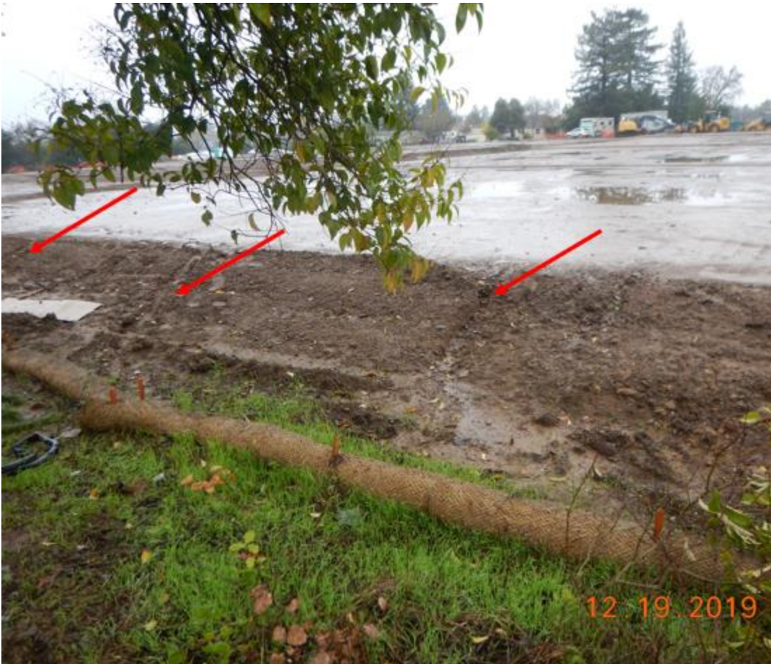
Photo 2: The red arrows indicate locations where erosion had already occurred. Sediment deposition from these rills can be seen leading towards Marlow Road. Photo taken and edited by Joshua Luders.
