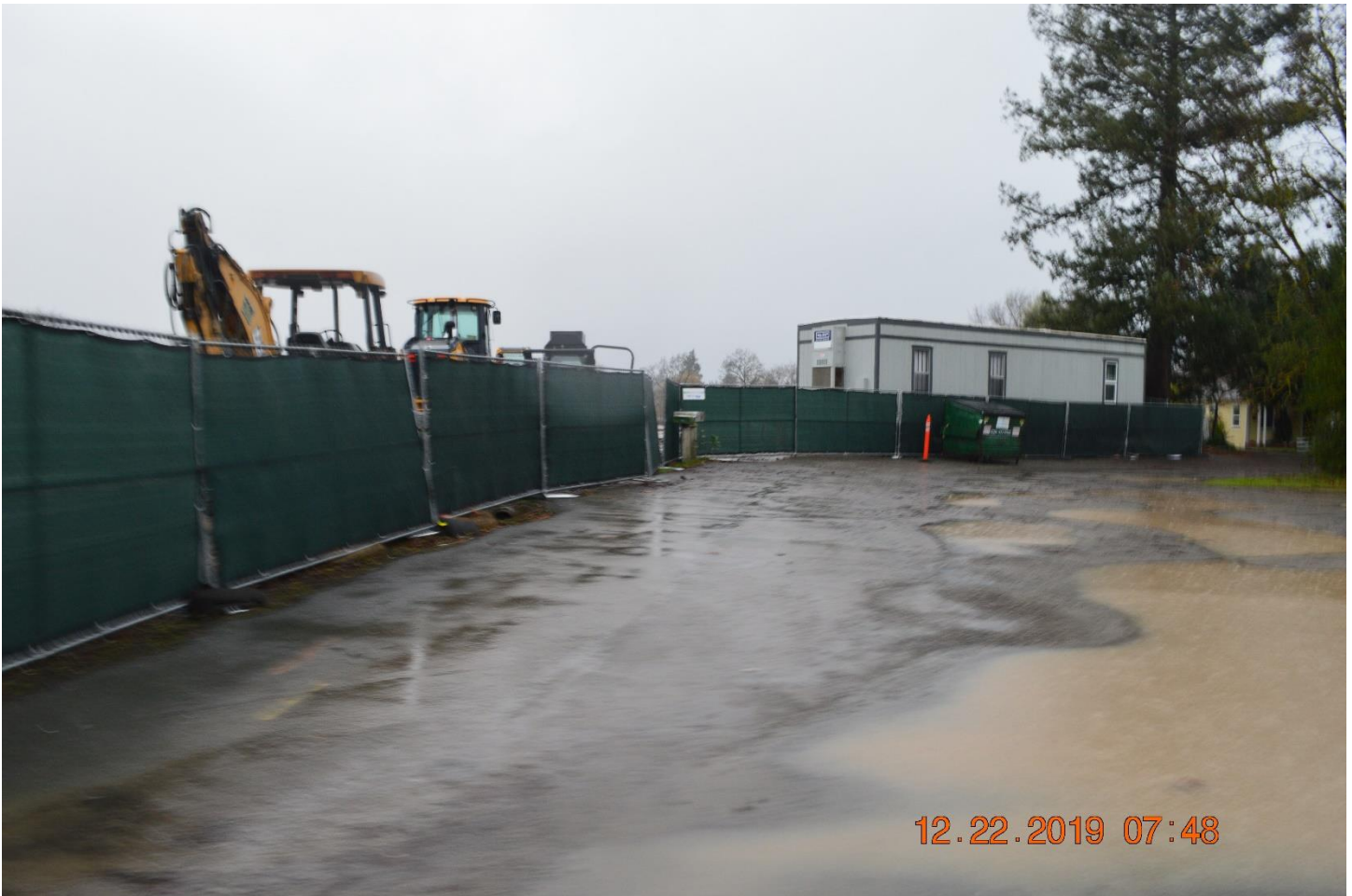
Photo 2: Construction entrance near Marlow road is closed. Photo taken by Joshua Luders.
