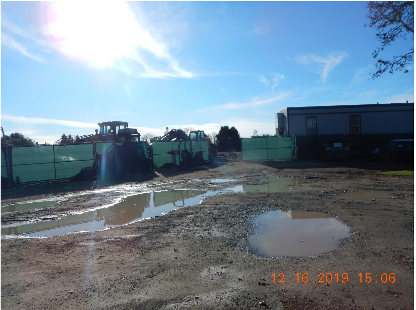
Photo 5: Construction entrance near Marlow Road. Photo taken by Joshua Luders during inspection on December 16, 2016.
