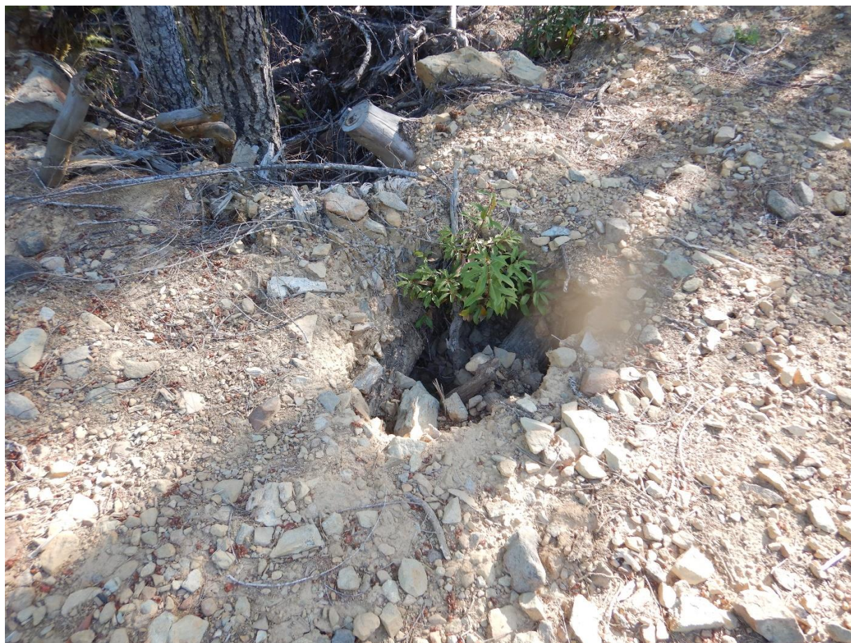
Photo 6— Downstream edge of road fill in the vicinity of WQ 6. Note the hole in fill showing woody debris in the matrix of material.
