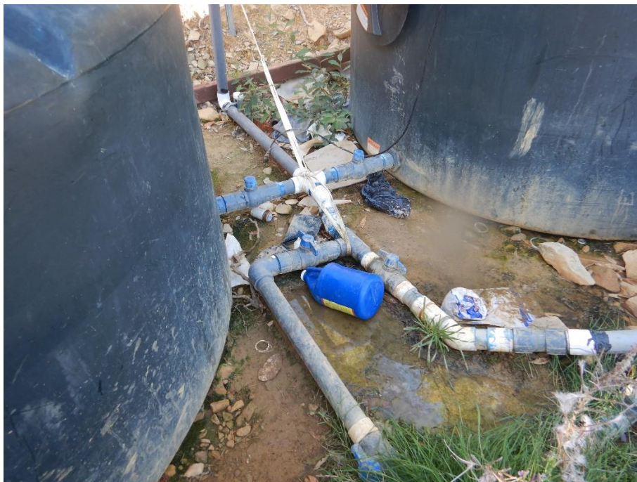
Photo 1—Tanks located at WQ 1
