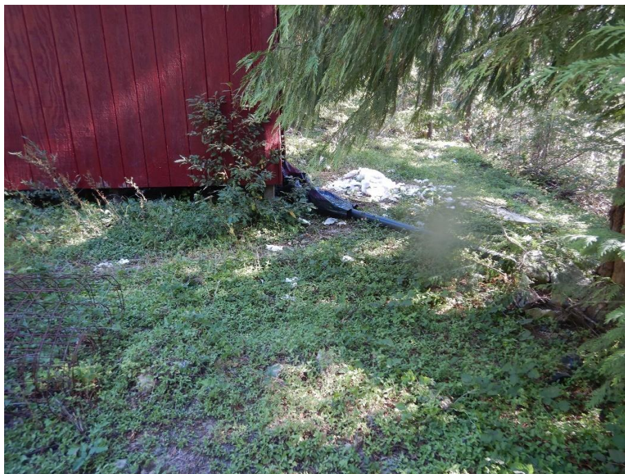
Photo 12— Outhouse discharging human waste where it is likely to enter receiving waters. Note the pile of soiled toilet paper at the back of the structure which is also likely to enter receiving waters.
