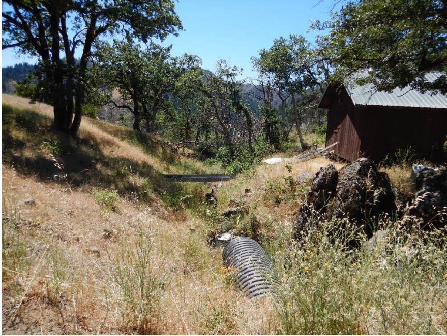
photo 15 —Picture taken looking south at undersized culvert outlet located at WQ 13.
