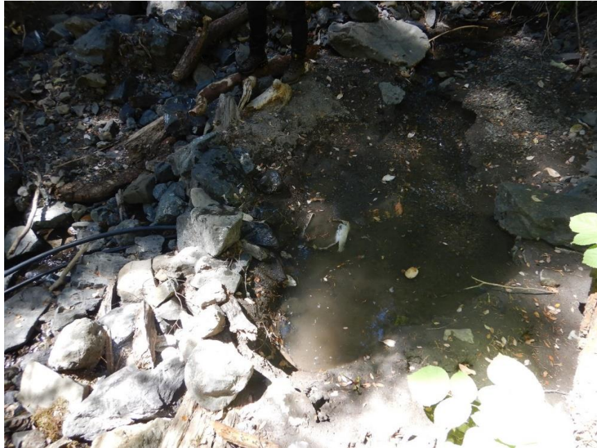
photo 13 —Watercourse dammed in the vicinity of WQ 15, to facilitate a water diversion.
