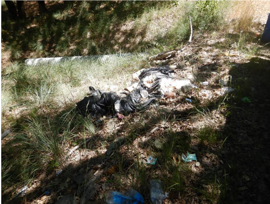
Photo 7—Refuse above culvert outlet in the vicinity of WQ 6.
