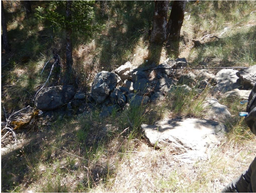
Photo 3—Pond outflow discharges to watercourse. Note a relatively uniform distribution of small boulders fill the small headwater channel.
