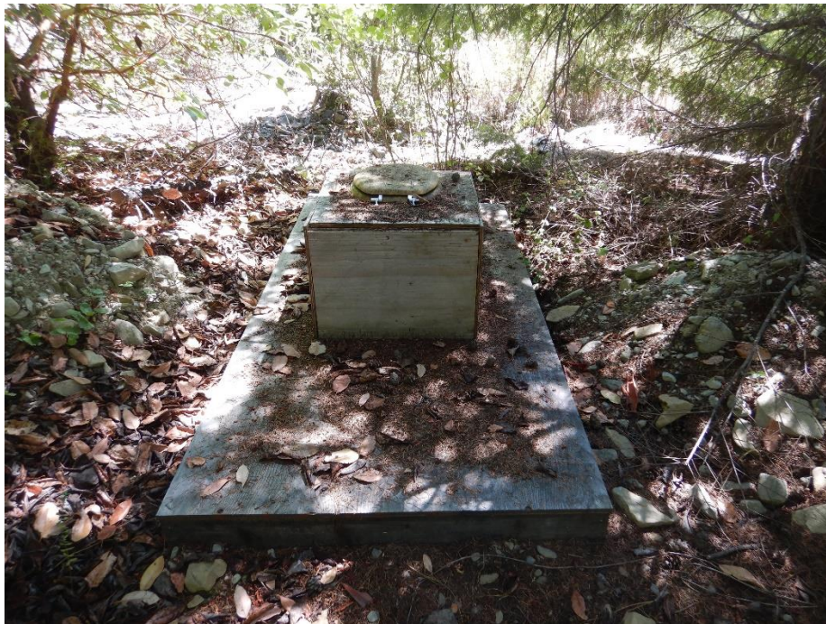
Photo 4—Pit Toilet located at WQ 4.
