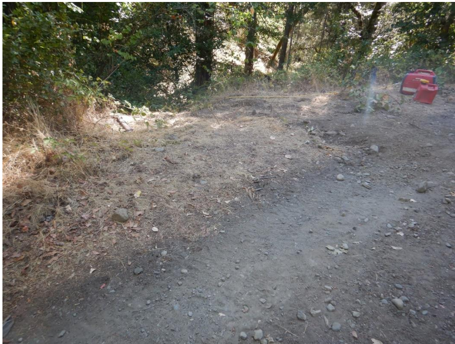
Photo 8—Trail leading to point of diversion at WQ 4. The footpath hydrologically connects the road to the watercourse.
