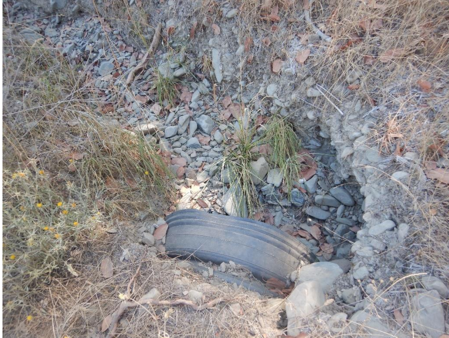
Photo 7—Inlet to culvert located at WQ 3. The upstream gradient is shallow and the culvert diameter is close to that of the channel width. The culvert is not aligned with the watercourse upstream and the bank has eroded upstream from the culvert inlet.
