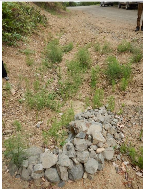
Photo 4 – FR2; culvert inlet surrounded by rock and view of road ditch discharging to culvert
