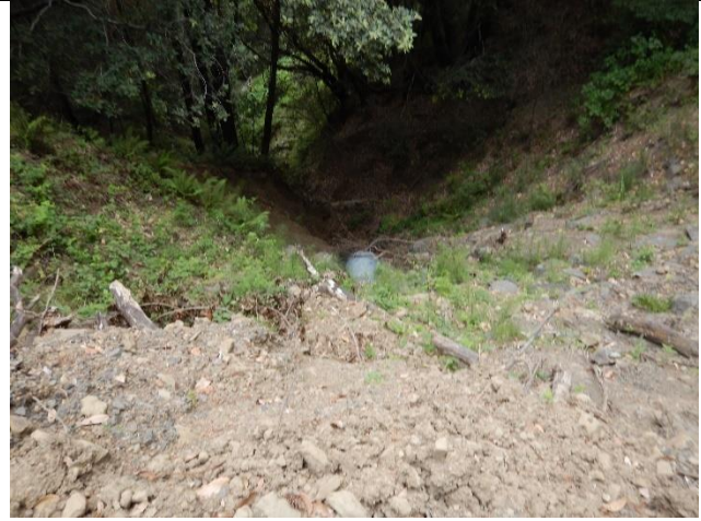
Photo 2 – FR1; looking down at culvert outlet standing on fill placed above the watercourse
