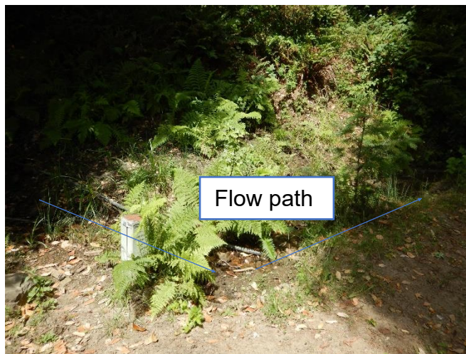
Photo 15 – FR10; watercourse with diversion pipe running through buried culvert and water diverted down ditch along road
