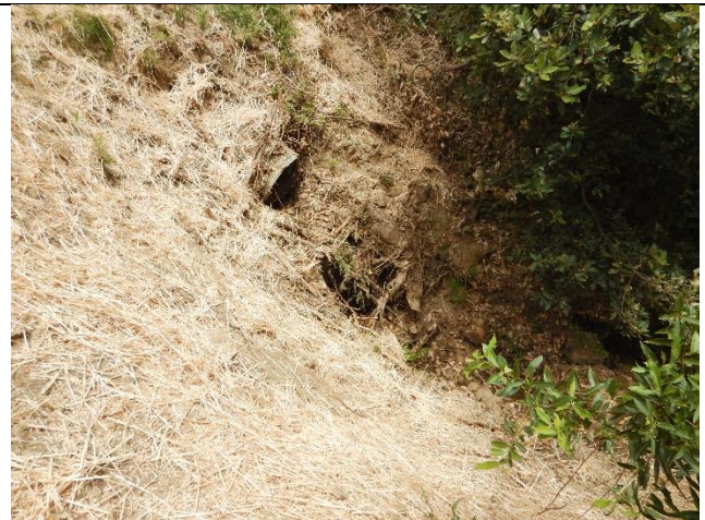
Photo 20 – FR15; culvert outlet perched above the watercourse channel
