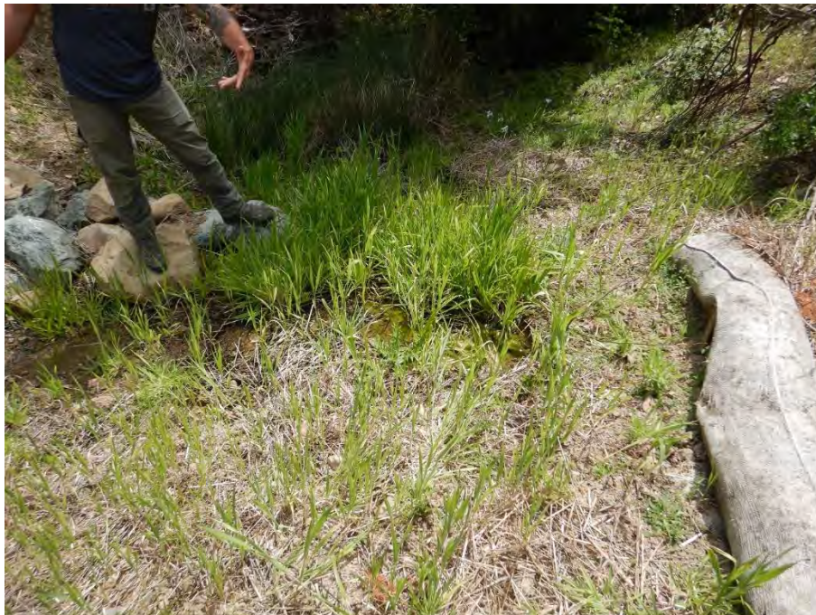
Photo 4—Groundwater seeping out of placed fill. Location identified as “seep” in Photo 1.
