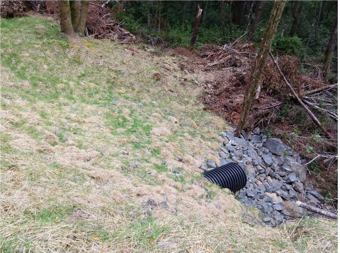
Outlet 1600 Crossing #11 (WRPP Site 13) New 30" culvert crossing adequately installed on grade with inlet and outlet armoring, and energy dissipater below outlet.
