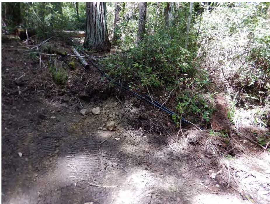
Photo 22—Looking upstream at earthen ford located at Map Point 19. An ephemeral watercourse can be seen parallel to the waterline among the duff. Heavy equipment tracks are visible on the road in the foreground of the image.
