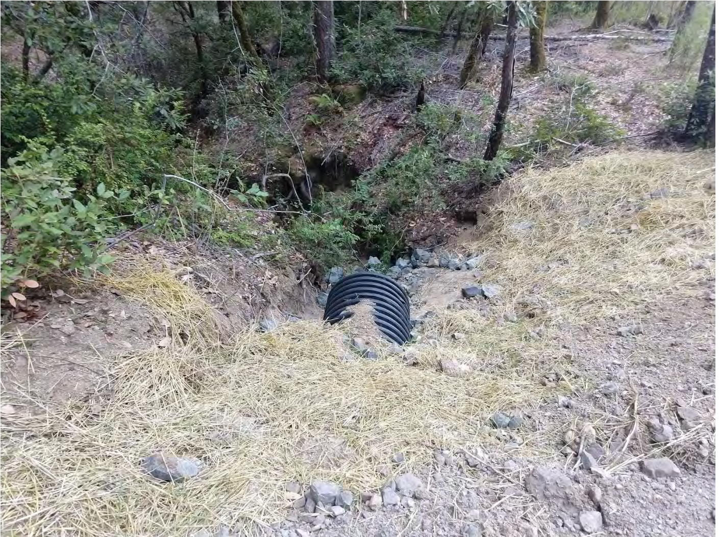
Outlet 1600 Crossing #6 (WRPP Site 07) New 24" culvert crossing adequately installed. Culvert is as close to grade and alignment as possible. Rock armor at inlet and outlet, energy dissipater below outlet.
