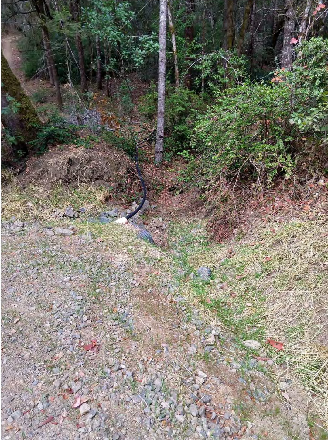
Inlet 1600 Crossing #10 (WRPP Site 12) New 30" culvert crossing adequately installed on grade with inlet and outlet armoring, and energy dissipater below outlet.
