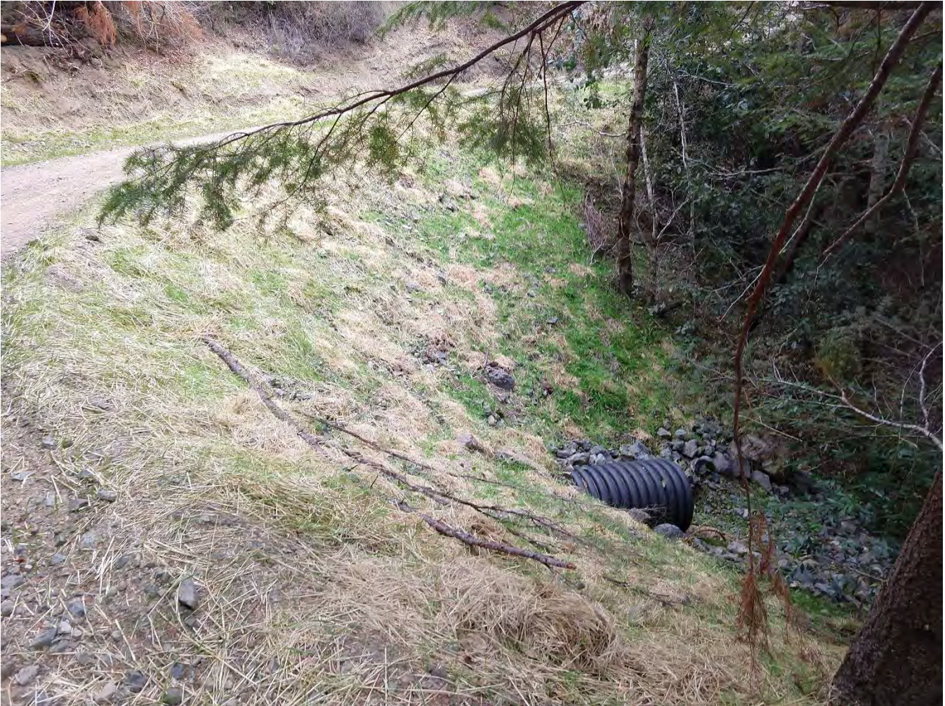
Outlet 1600 Crossing #12 (WRPP Site 14) New 36" culvert crossing adequately installed on grade with inlet and outlet armoring, and energy dissipater below outlet.
