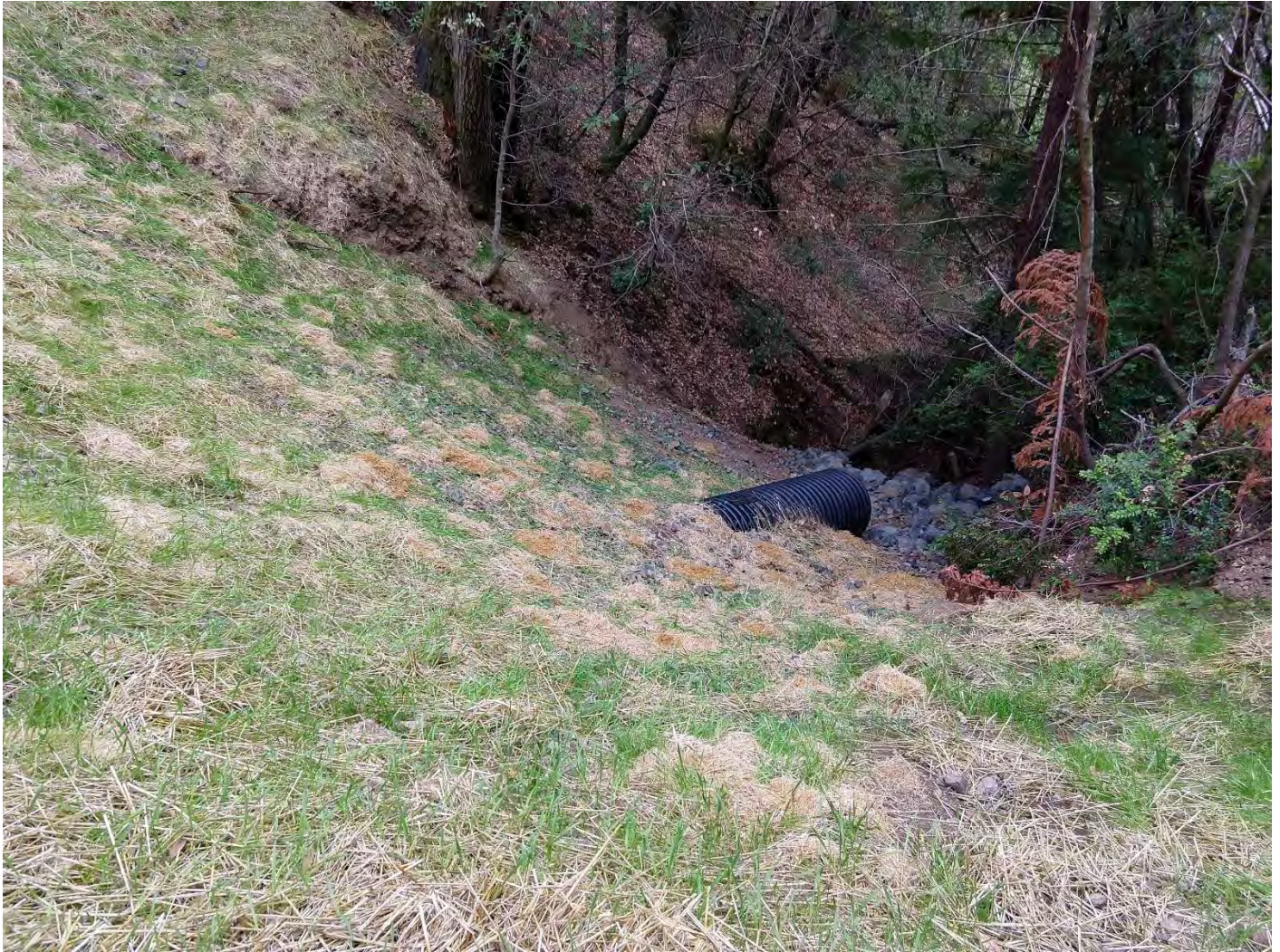
Outlet 1600 Crossing #13 (WRPP Site 15) New 36" culvert crossing adequately installed on grade with inlet and outlet armoring, and energy dissipater below outlet.
