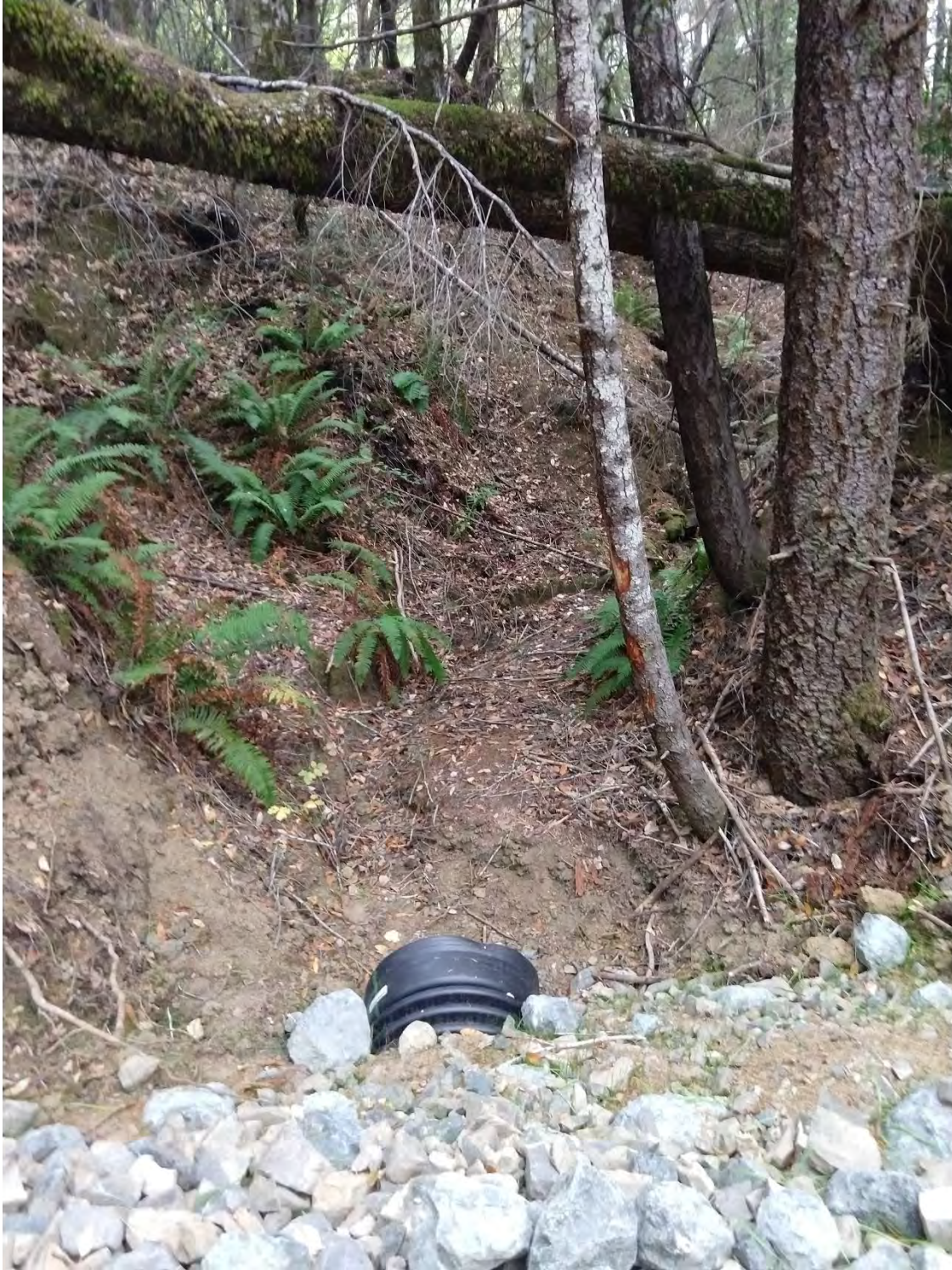
Inlet 1600 Crossing #8 (WRPP Site 10) New 18" culvert crossing adequately installed to grade with inlet and outlet armoring, and energy dissipater rock below outlet.
