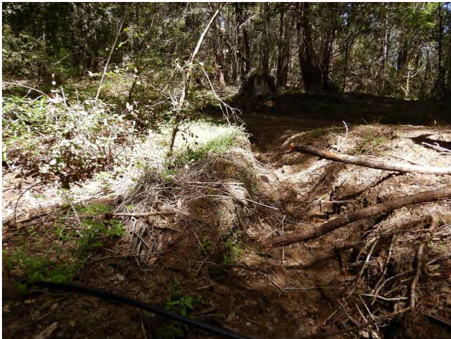
Photo 26—Looking north east in the vicinity of Map Point 17. Stormwater from the road in the upper left of the picture, flow down the ditch where the photographer is standing before entering a watercourse.
