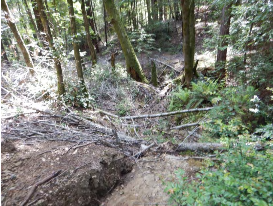
Photo 25—Looking south west in the vicinity of Map Point 18. Shows ditch that delivers stormwater from the road pictured in above photo.
