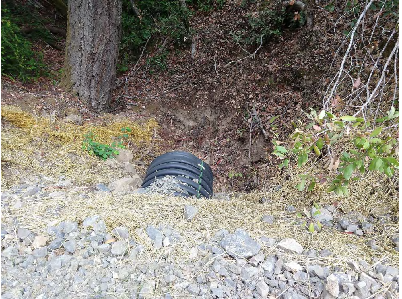
Inlet 1600 Crossing #7 (WRPP Site 08) New 30" culvert crossing adequately installed near grade with energy dissipater below outlet.
