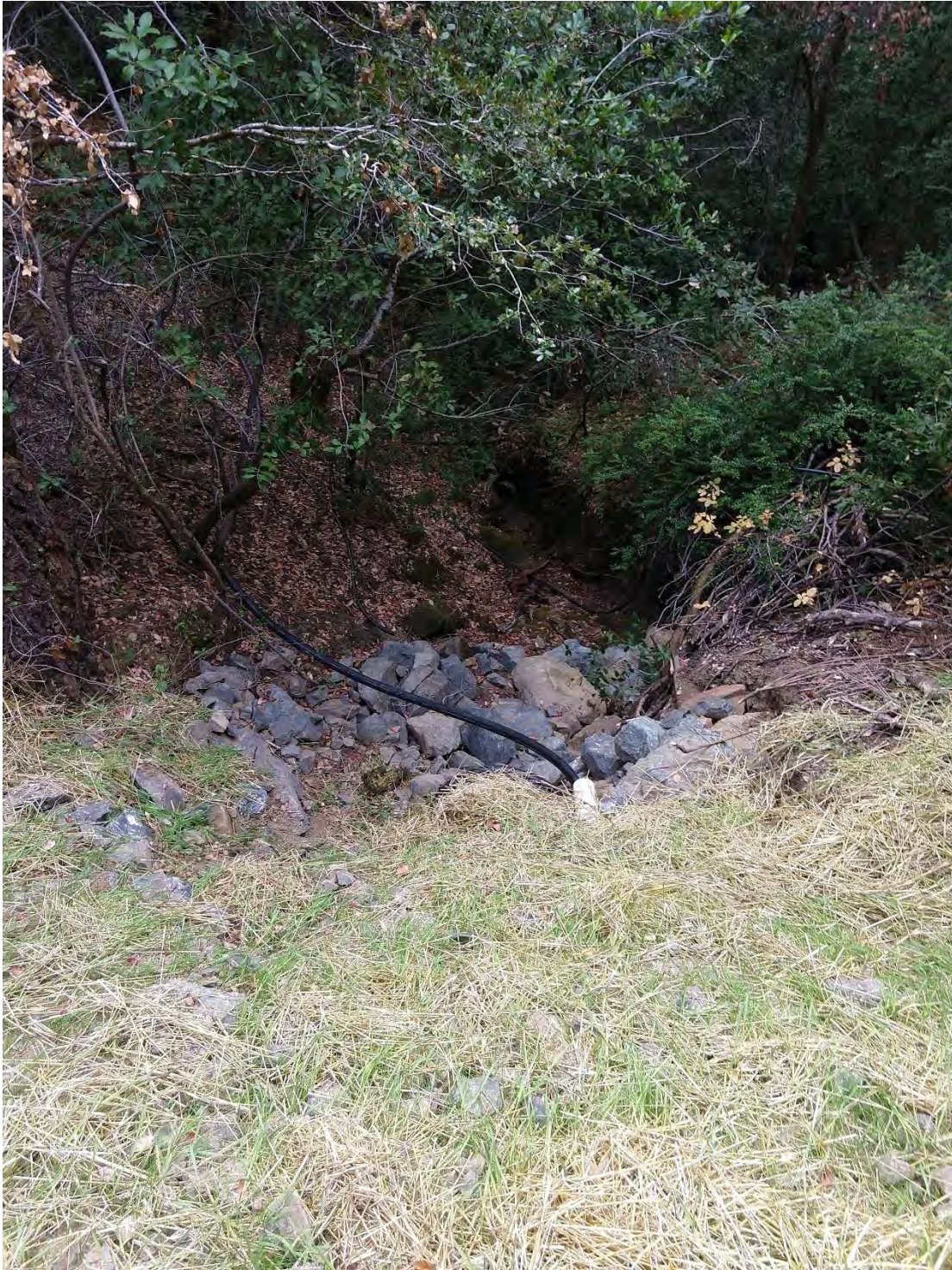
Outlet 1600 Crossing #10 (WRPP Site 12) New 30" culvert crossing adequately installed on grade with inlet and outlet armoring, and energy dissipater below outlet.
