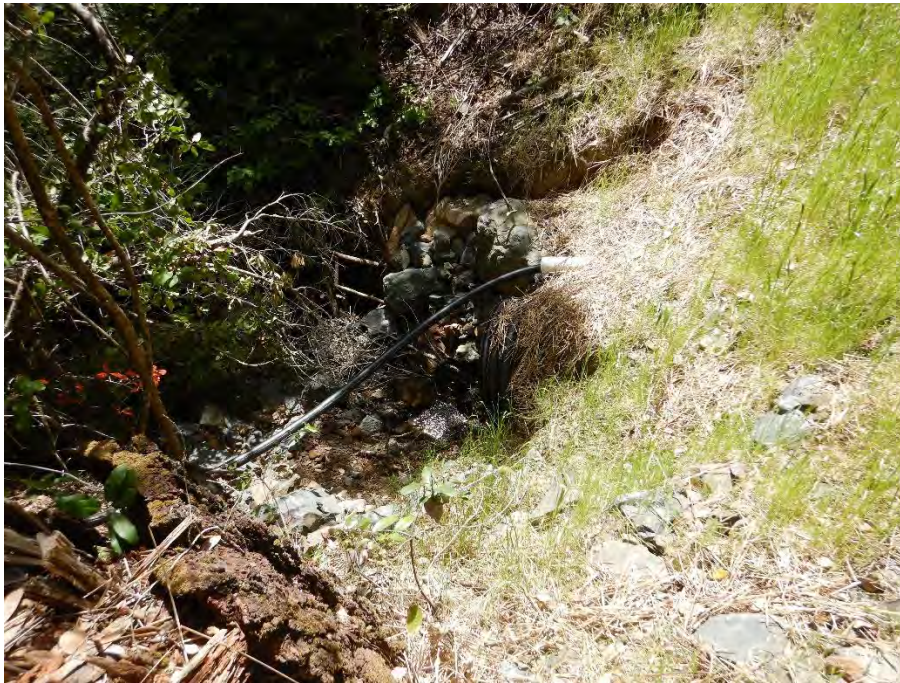
Photo 28—The culvert outlet at Map Point 12 is perched approximately one foot.
