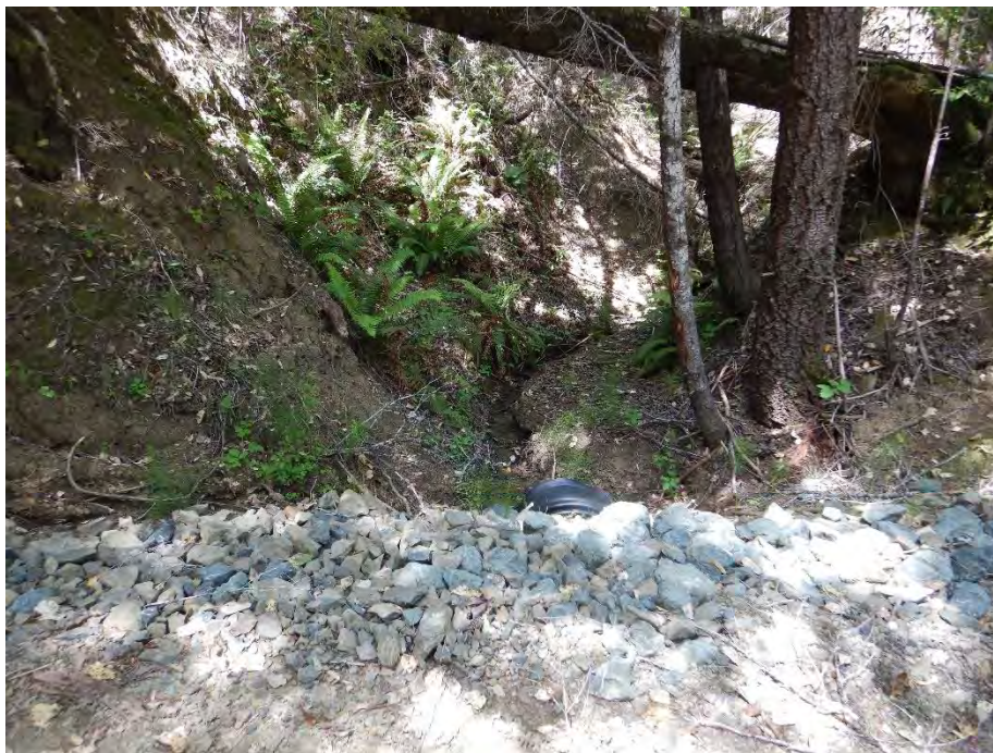
Photo 30—Looking at the inlet of the 18-inch diameter culvert at Map Point 10. The inlet is armored with small boulders and the active channel width is approximately 12 inches.
