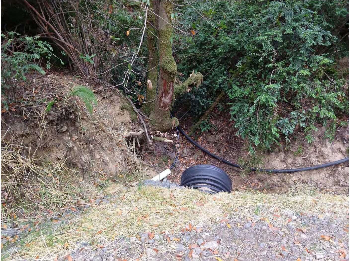
Inlet 1600 Crossing #11 (WRPP Site 13) New 30" culvert crossing adequately installed on grade with inlet and outlet armoring, and energy dissipater below outlet.
