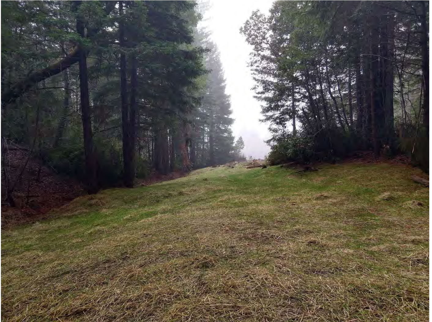
1600 Map Point #18 (WRPP Site 25) Fill removed from watercourse and slopes re-contoured well. Erosion control measures in place. Vegetation plan not yet implemented.
