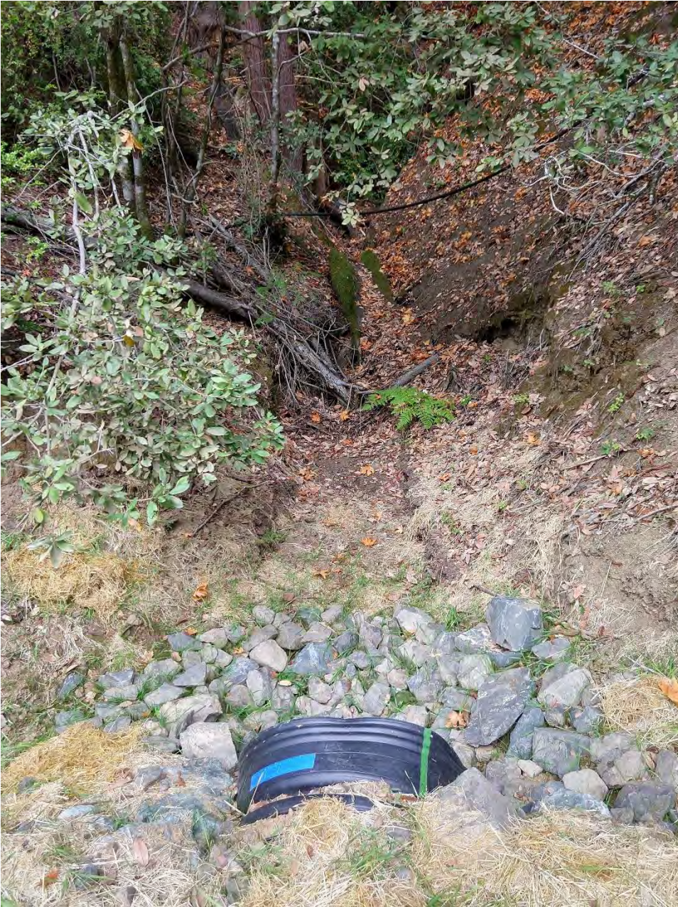
Inlet 1600 Crossing #13 (WRPP Site 15) New 36" culvert crossing adequately installed on grade with inlet and outlet armoring, and energy dissipater below outlet.
