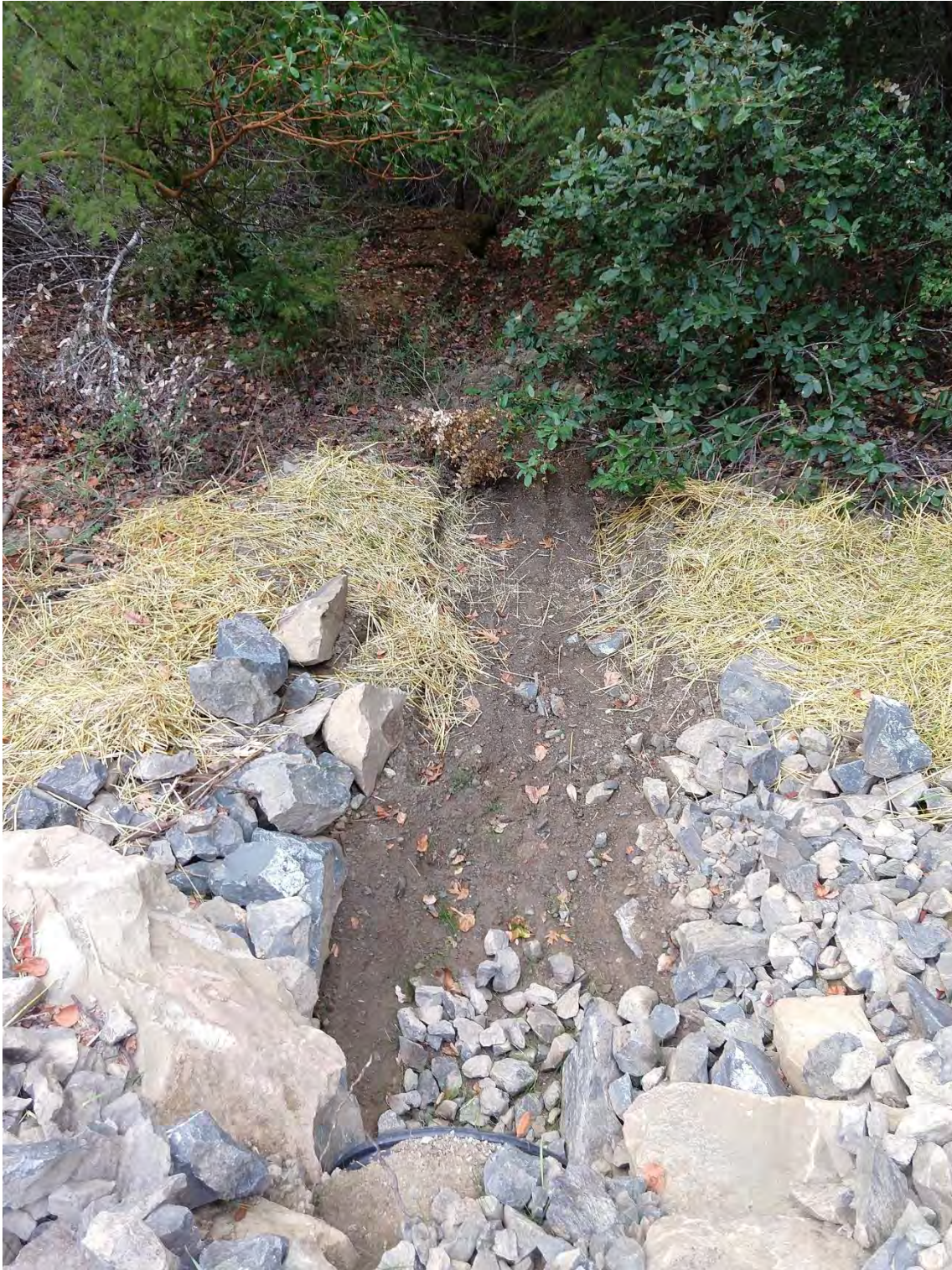
Outlet 1600 Crossing #9 (WRPP Site 11) New 24" culvert crossing adequately installed on grade with inlet and outlet armoring.
