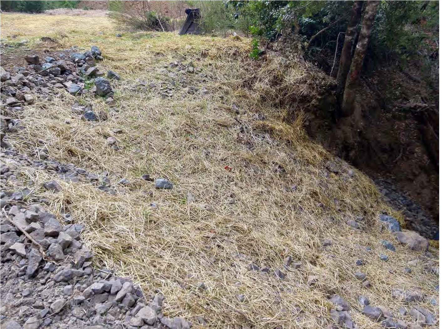
Erosion Control 1600 Crossing #7 (WRPP Site 08) New 30" culvert crossing adequately installed near grade with energy dissipater below outlet.
