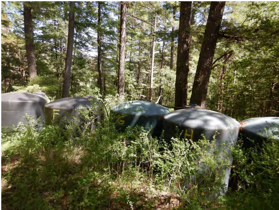
Photo 32—Water tanks located east of Map Point 5. Water was overflowing the top of Tank G.
