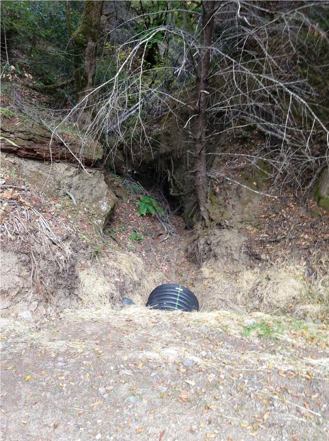
Inlet 1600 Crossing #12 (WRPP Site 14) New 36" culvert crossing adequately installed on grade with inlet and outlet armoring, and energy dissipater below outlet.
