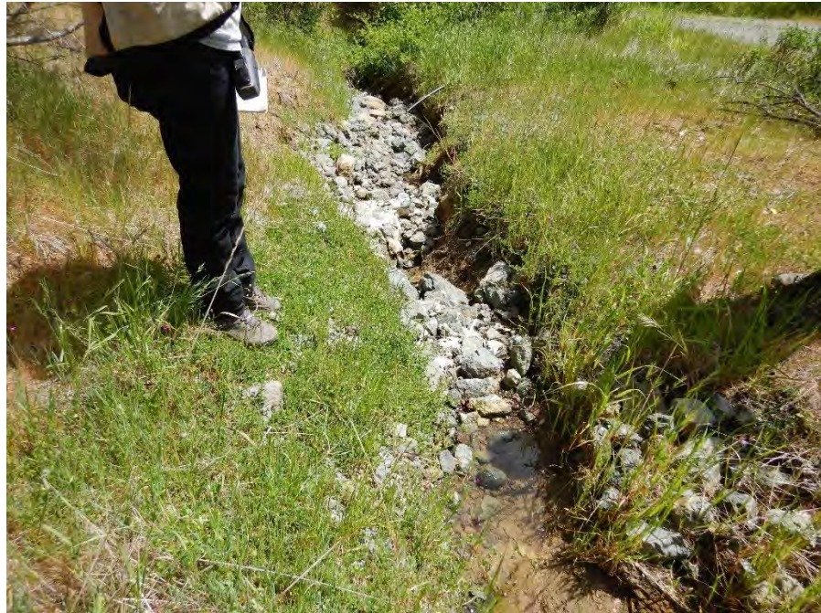
Photo 10—Watercourse in the vicinity of Map Point 23, downstream from the location pictured in the previous image. Note water is flowing and large cobbles had been added, armoring the watercourse.
