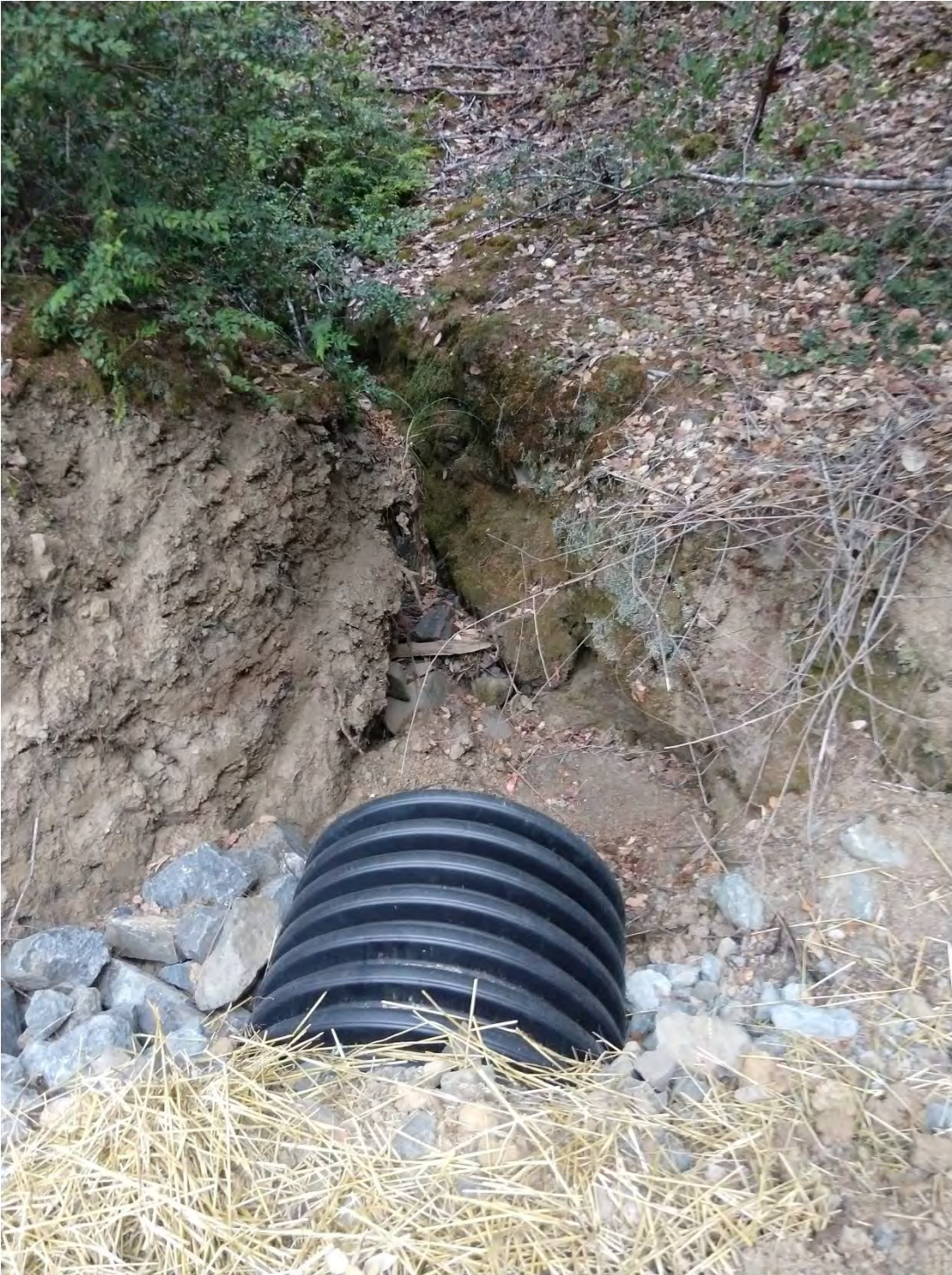
Inlet 1600 Crossing #6 (WRPP Site 07) New 24" culvert crossing adequately installed. Culvert is as close to grade and alignment as possible. Rock armor at inlet and outlet, energy dissipater below outlet.
