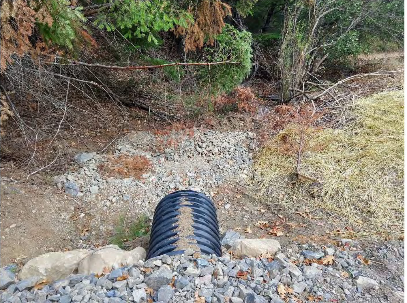
Inlet 1600 Crossing #9 (WRPP Site 11) New 24" culvert crossing adequately installed on grade with inlet and outlet armoring.
