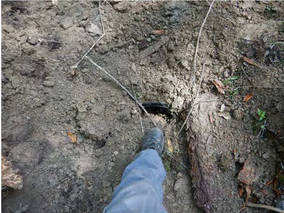
Photo 31—Undersized pipe with buried inlet in the vicinity of Map Point 5.
