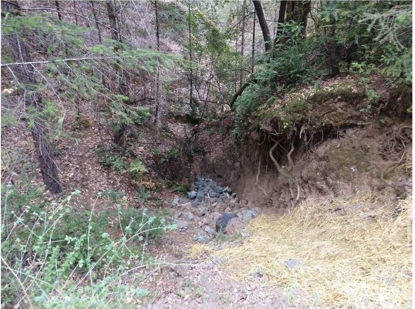
-1600 Crossing #5 (WRPP Site 06) Energy dissipater rock installed below existing outlet appears adequate.
