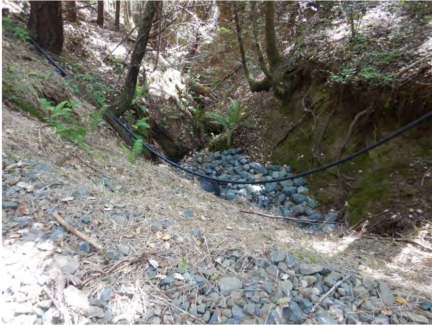
Photo 29—Looking at the outlet of an 18-inch diameter culvert at Map Point 10. The channel bed is armored with small boulders and turns approximately 15 degree to the left immediately downstream from the culvert outlet.
