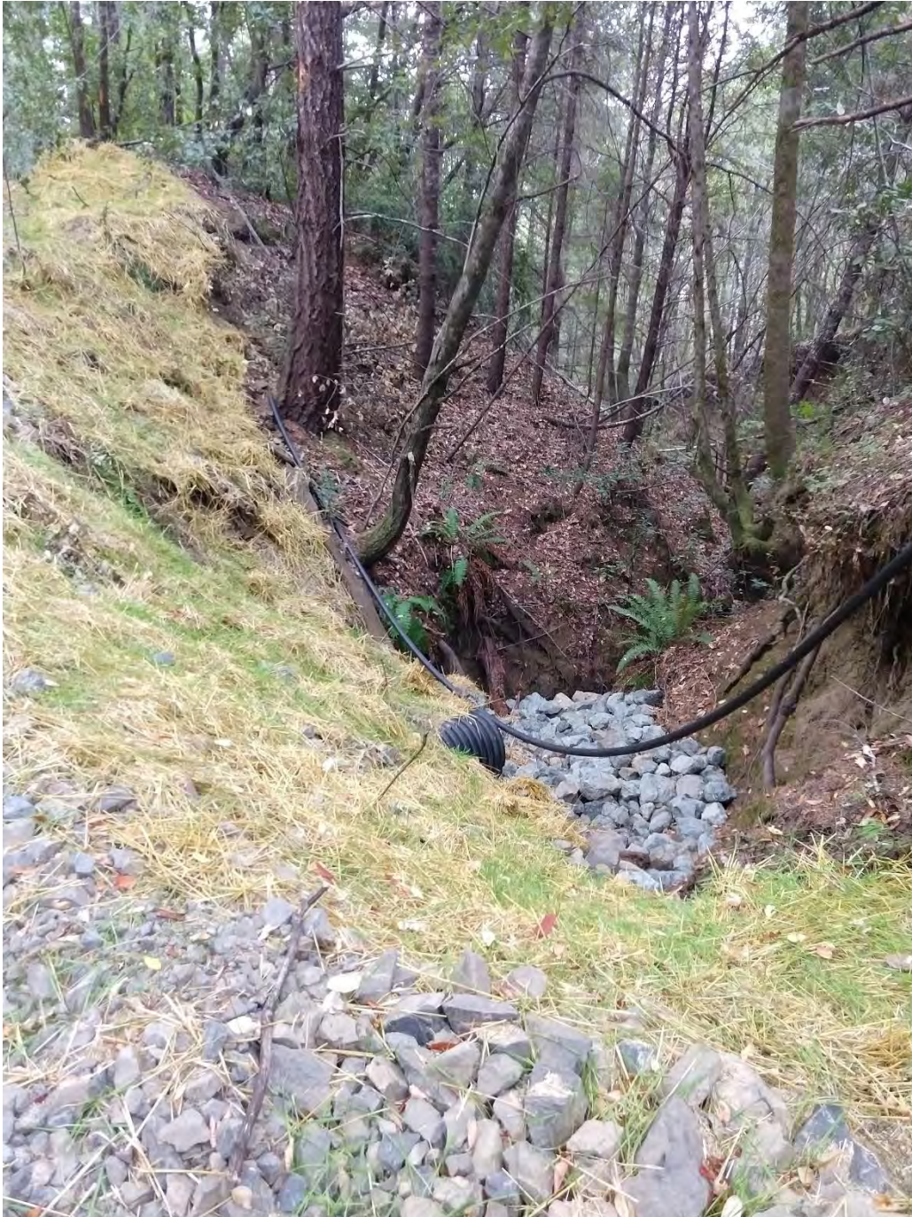
Outlet 1600 Crossing #8 (WRPP Site 10) New 18" culvert crossing adequately installed to grade with inlet and outlet armoring, and energy dissipater rock below outlet.
