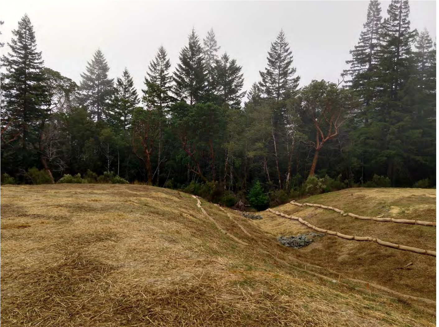
1600 Crossing #15 (WRPP Site 24) Excavation of fill material placed in channel. Channel reconstruction appears adequate. Grade is consistent with natural topography and adjoining channel. Rock check-dams installed at regular intervals for grade control. Side slopes laid back to 30%. Straw wattles installed on channel banks. Erosion control measures in place for disturbed soil surfaces. Vegetation plan not yet implemented.
