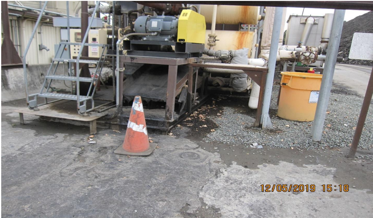
Picture 7 – View of industrial equipment in processing area. Oily material was observed in this area under the equipment. Spill prevention kits were not available on-site during the inspection. No containment controls BMPs were installed.
