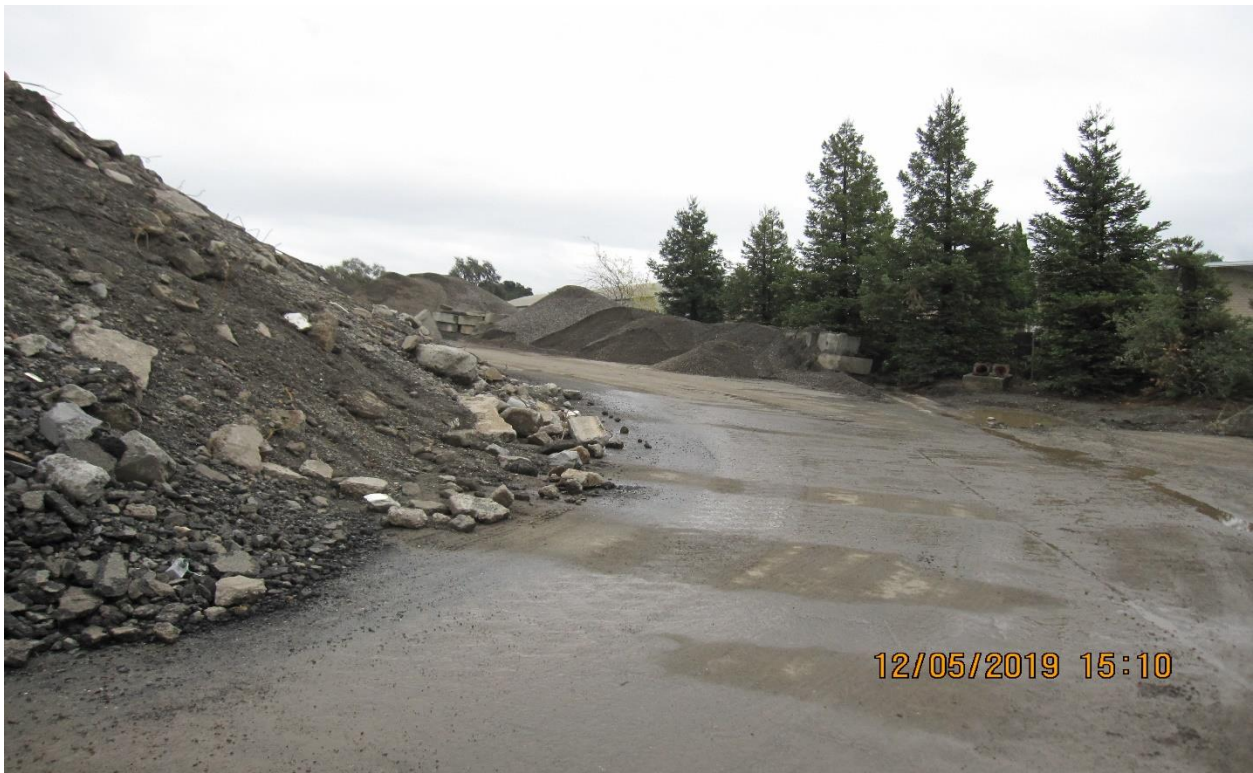
Picture 6 – View of unprotected asphalt recycling material and aggregate stockpiles located upstream of the settling tanks and ponds. No stockpile protection or perimeter control BMP installed.
