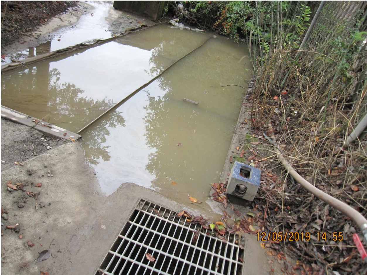
Picture 1- View of muddy settling tanks at the end of the bio swale. Significant sediment accumulation observed, and the inlet is not protected. Oil sheen observed in some areas.
