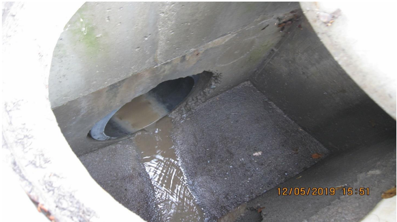
Picture 8 – View inside the public storm drain system of the discharge leaving the facility. This location the sampling point for the facility. The entire facility drains to this location and is the only source of the discharge. The discharged water is turbid. (Refer to the attached site map for location)
