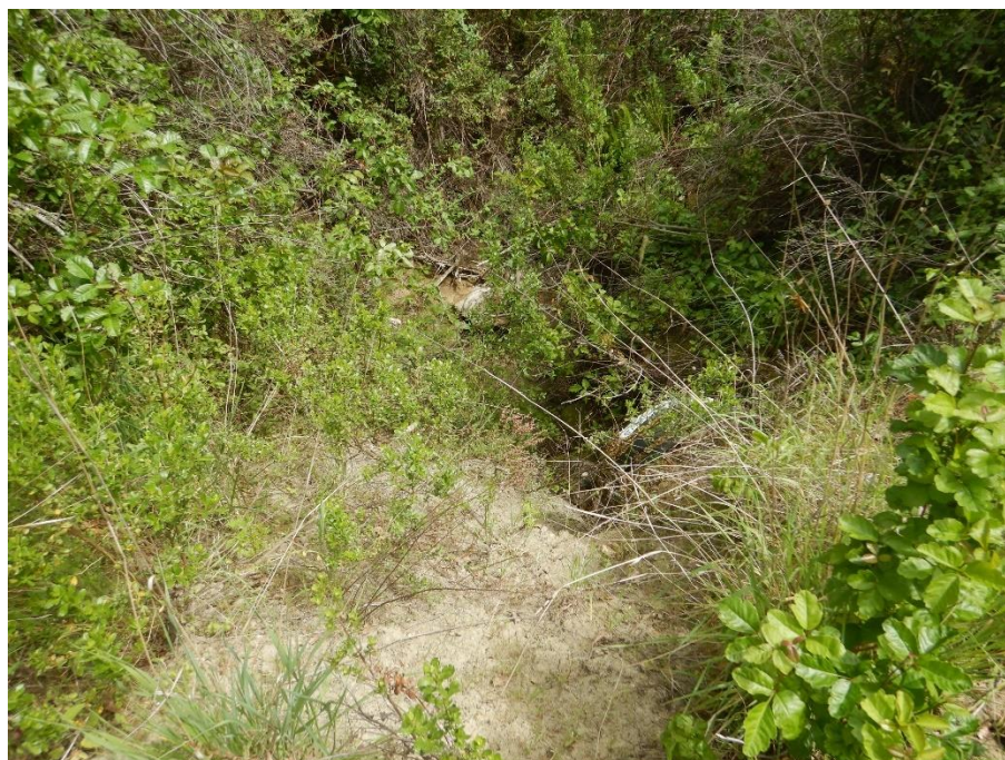
Photo 28—Looking east from the easternmost road, west of Buck Mountain Creek, which exits the property to the south. A culvert receiving flow from two watercourses. The watercourses are incising both upstream and downstream from the culvert.
