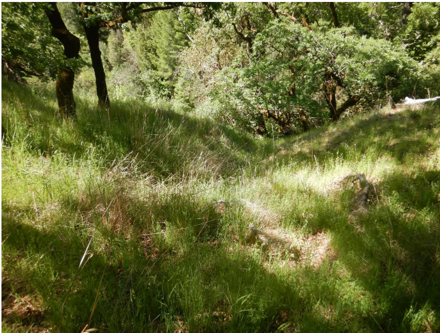
Photo 10—Swale where channelization is evident 170 feet downstream from the previous image. The channel steepens precipitously past the first row of trees in the back of the image before joining Panther Canyon.
