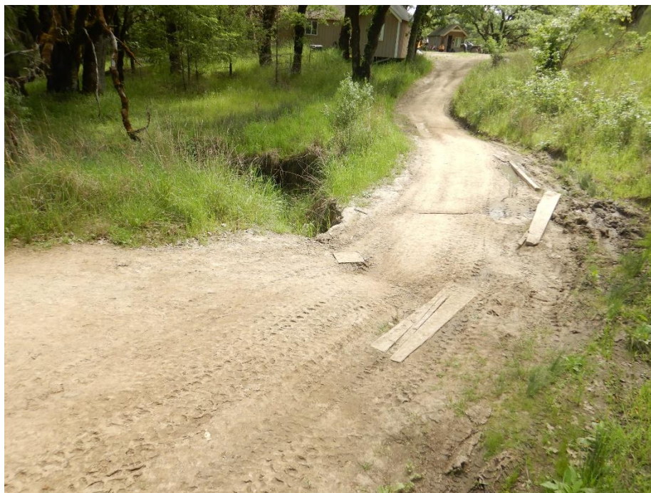
Photo 23—Stormwater from the road leading to Site 4 (Photo 21), the ditch in Photo 22, and a watercourse converge and flow over the road in the center of the image.
