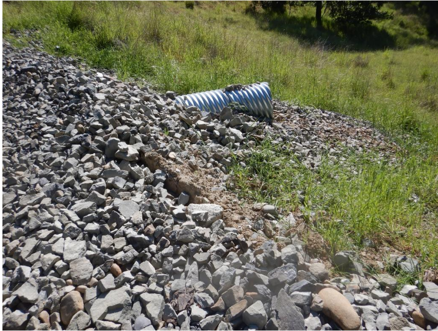
Photo 3—Outlet of the ditch relief culvert on steep section of road approaching Site 7.
