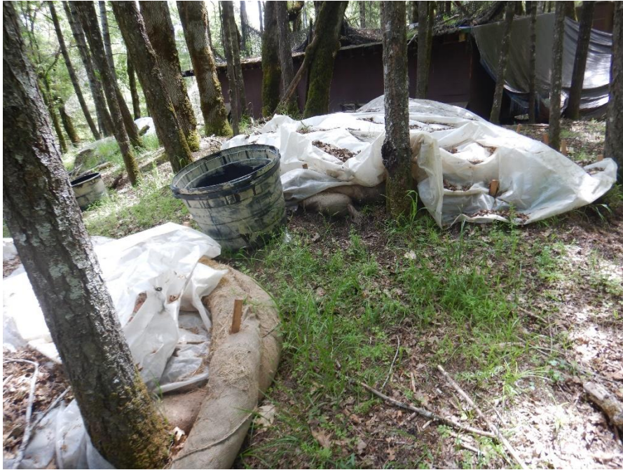
Photo 31—Three piles of imported potting soil covered and surrounded by wattles at Site 3.
