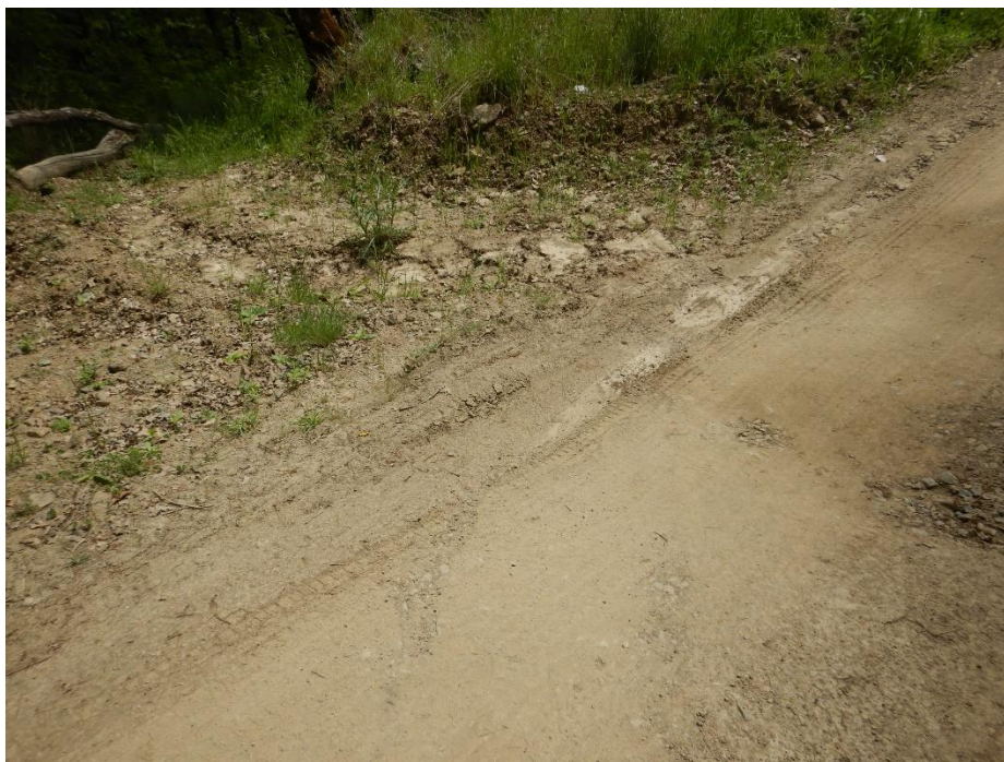
Photo 27—Location where stormwater exits the dirt-surfaced parking area in front of the small cabins pictured in previous image.
