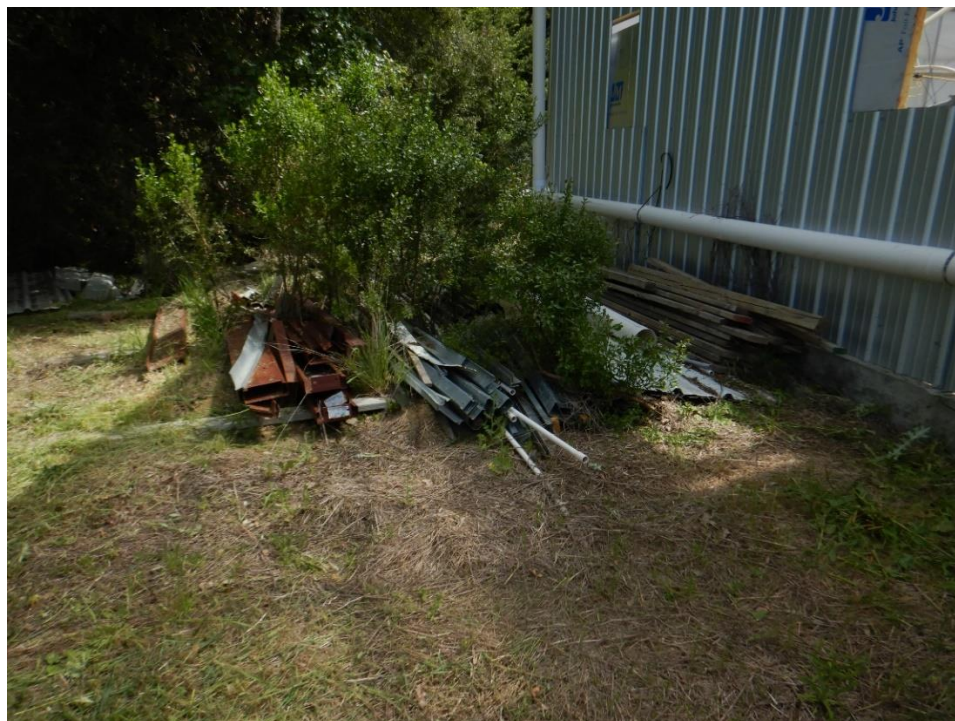
Photo 15— The northern exterior of the Glass House at Site 1. The piping strapped to the side of the building conveys stormwater collected by the roof to an area east of the pad.
