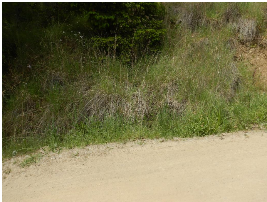
Photo 22—Location where spring-flow enters a roadside ditch instead of being conveyed across the road.
