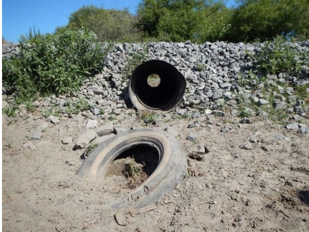
Culvert inlet. Probably 24-inch diameter. Tire is from neighbor's past discharge upstream.
