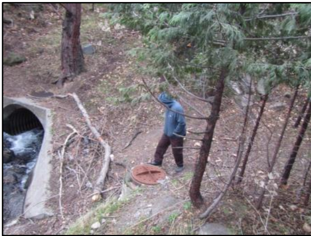
Photo 3: Inspection of the manhole located where the SSO occurred which is immediately adjacent to Boles Creek. The City was unable to lift the manhole cover at time of the inspection.
