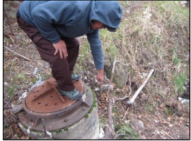
Photo 6: Inspection of manhole barrel revealed solid materials present.
