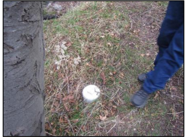
Photo 8: A white-capped cleanout was observed approximately 50 feet east of the manhole adjacent to Boles Creek. The City staff said they were unaware of this asset and unsure of its purpose.
