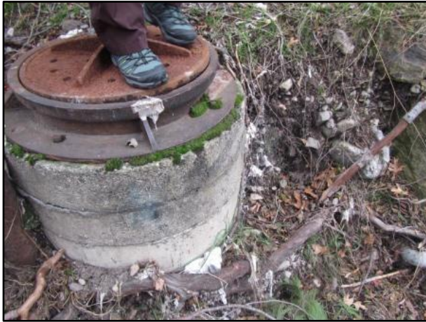
Photo 7: Close-up of the solid materials. Note the manhole cover was a slightly lifted from its base ring.
