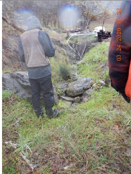
Photo 12 – Squashed culvert stream crossing
