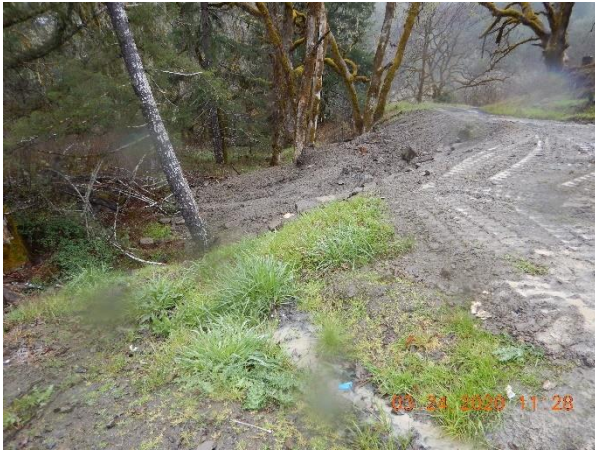
Photo 11 – Road fill pushed into and perched above watercourse
