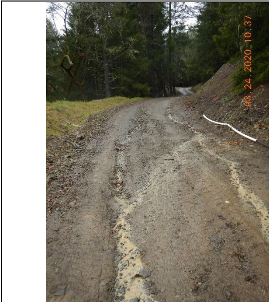
Photo 3 – Surface erosion on road
