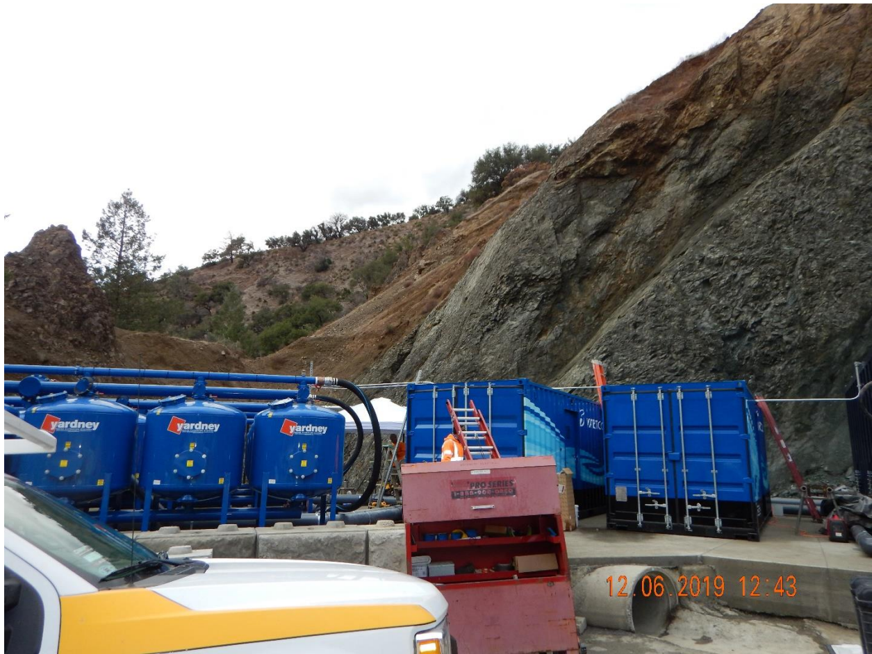
Figure 2: Newly installed treatment systems # 1 & 2
