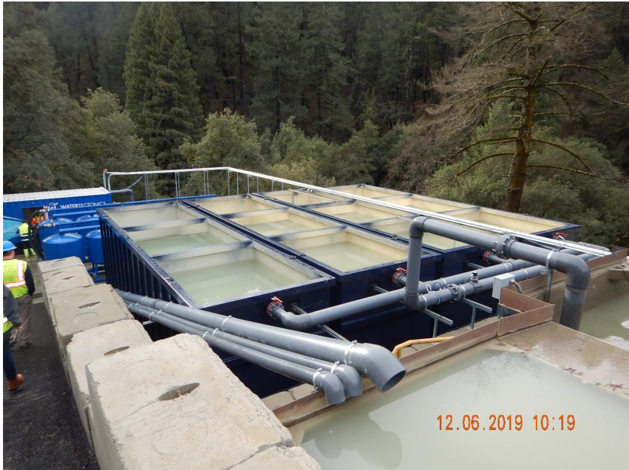
Figure 3: Newly installed treatment systems # 3
